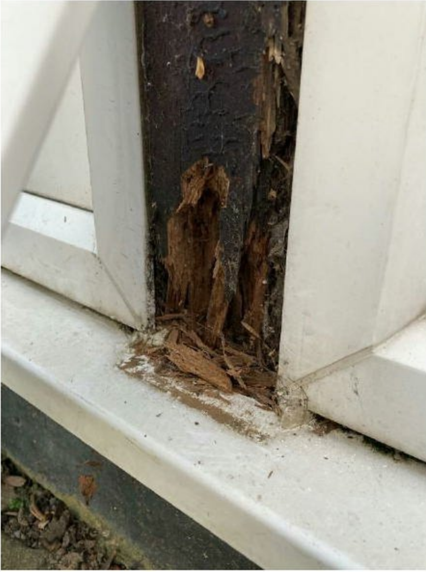
Figure 4 - Localised damage observed to the base of a structural timber column.
