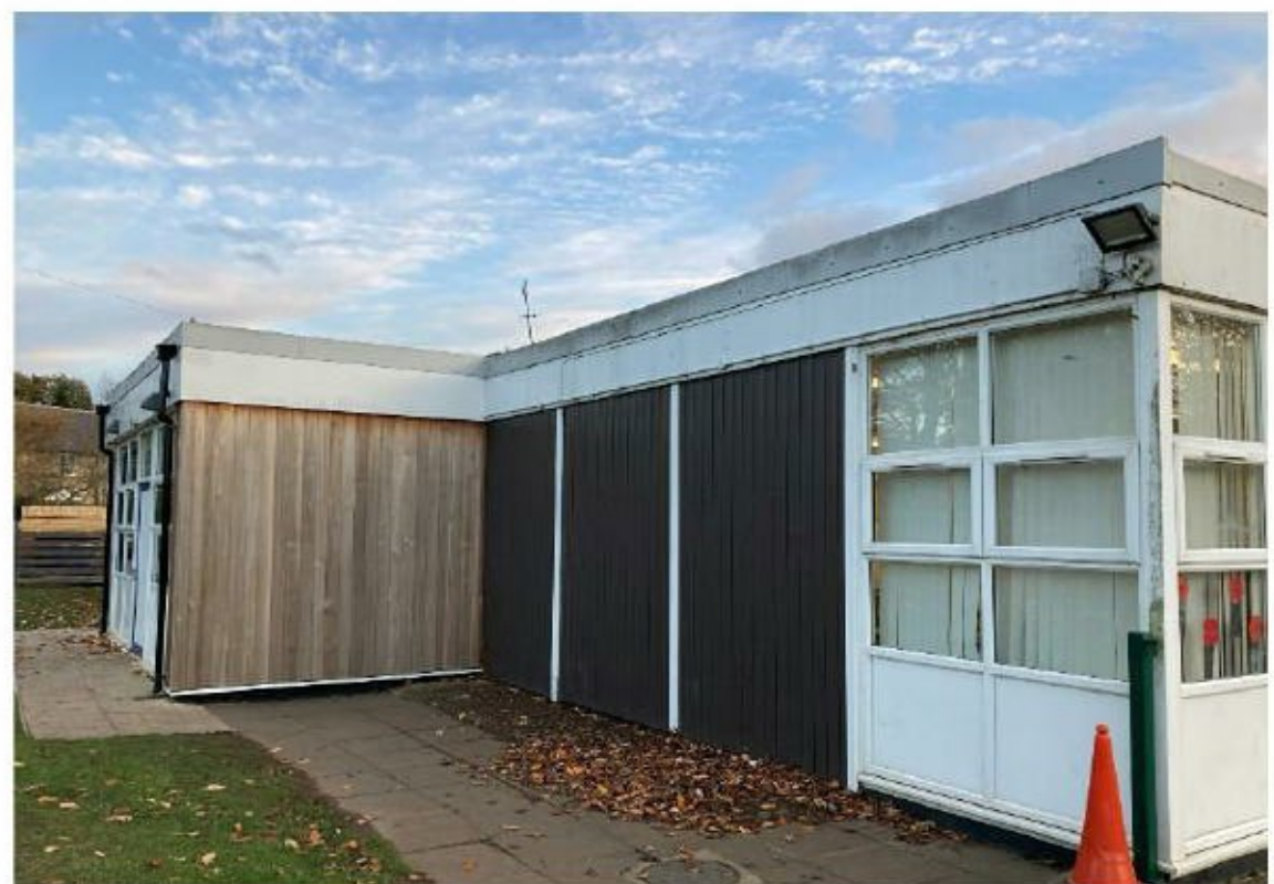
Figure 1 - Ovingham First School, showing the junction between an original and a relatively new element of the building.
