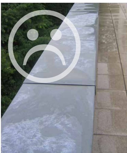
Zinc hydroxide formation due to insufficient slope
