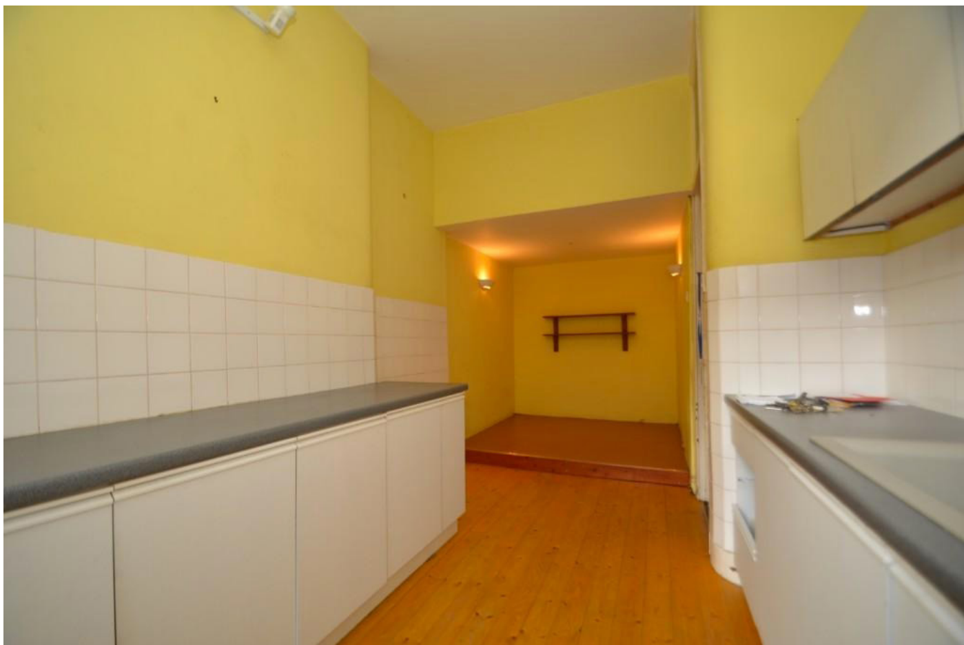
Chimney brest on left to be partially removed. Raised floor and boxed in ceiling to be removed to gain full height
