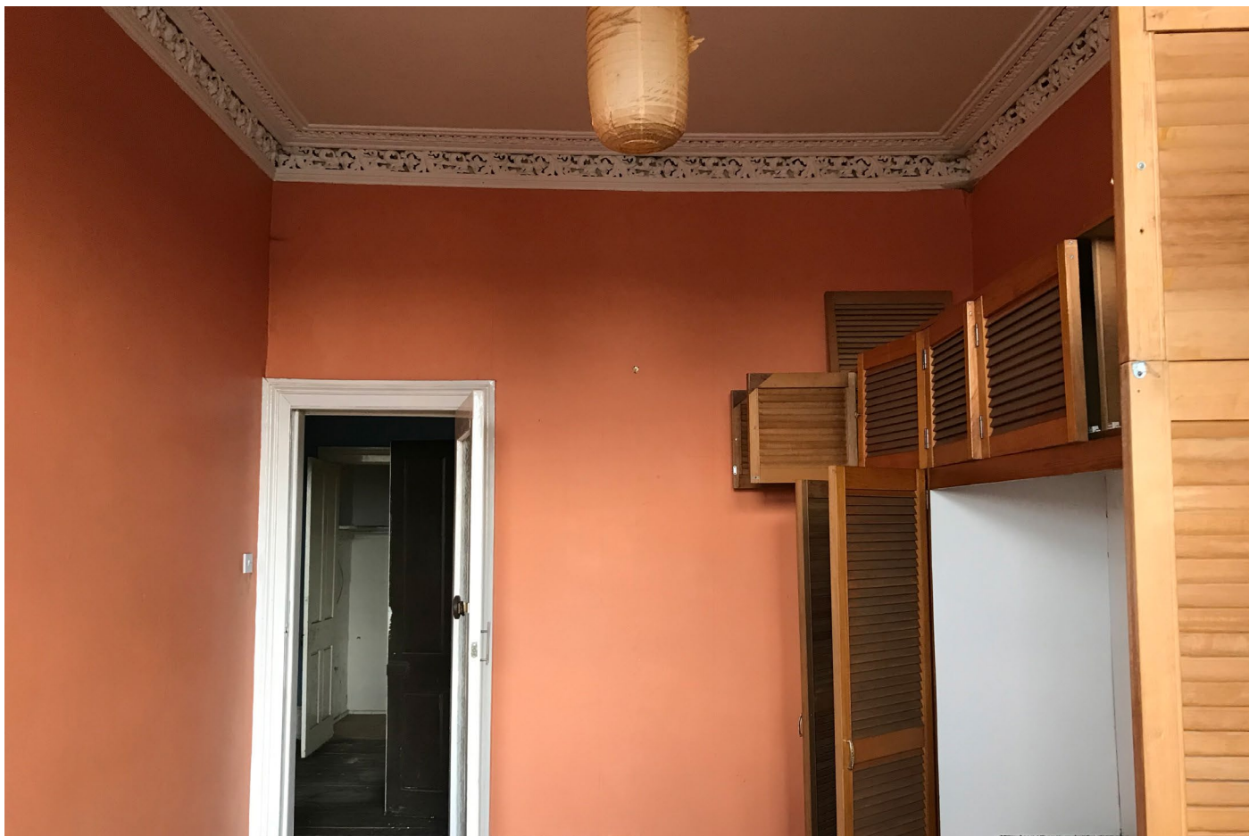
Wall affected by new high level window. See relevant drawings for details
