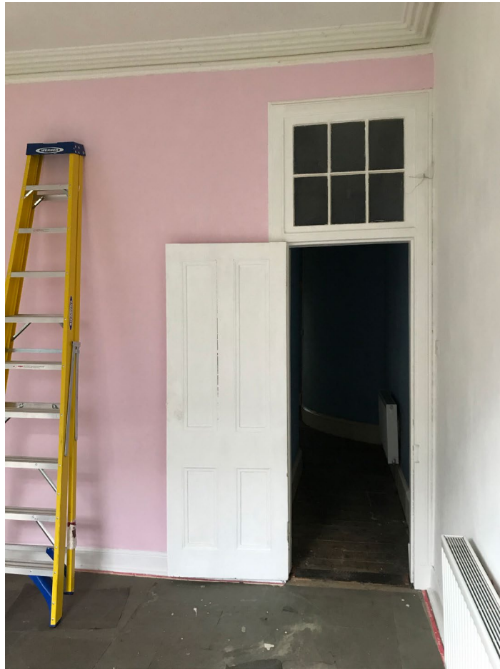
New transom windows to kitchen and living room to mimic this one in bedroom 1
