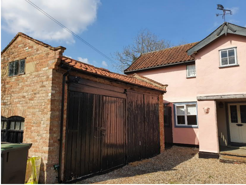
Photo 2: - View looking at the existing garage showing the access to the door is blocked by the porch.
