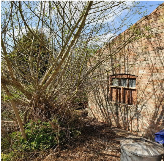
Photo 4: - Side view of garage showing the willow which has undermined the foundations.
