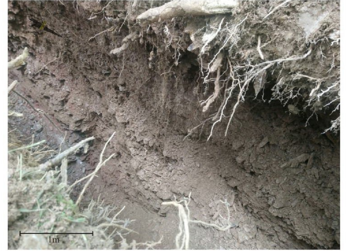
Photograph 3. Southern edge of quarry marked by shelf of intact weathered metamorphic bedrock at 2.5m beneath present surface level. Note uniform stony fill to north, confirmed to extend to approximately 4.5m beneath surface levels.
