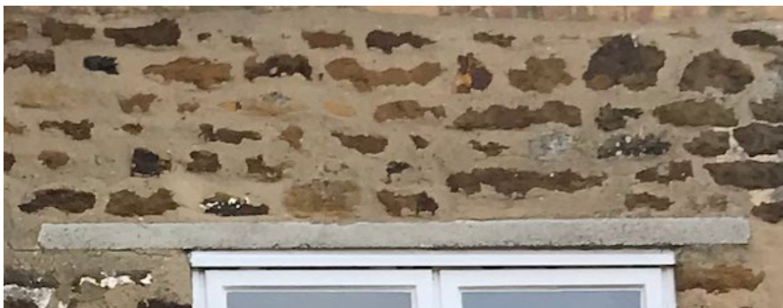
Fig. 11: Example of unsympathetic cement strap pointing on north elevation.
