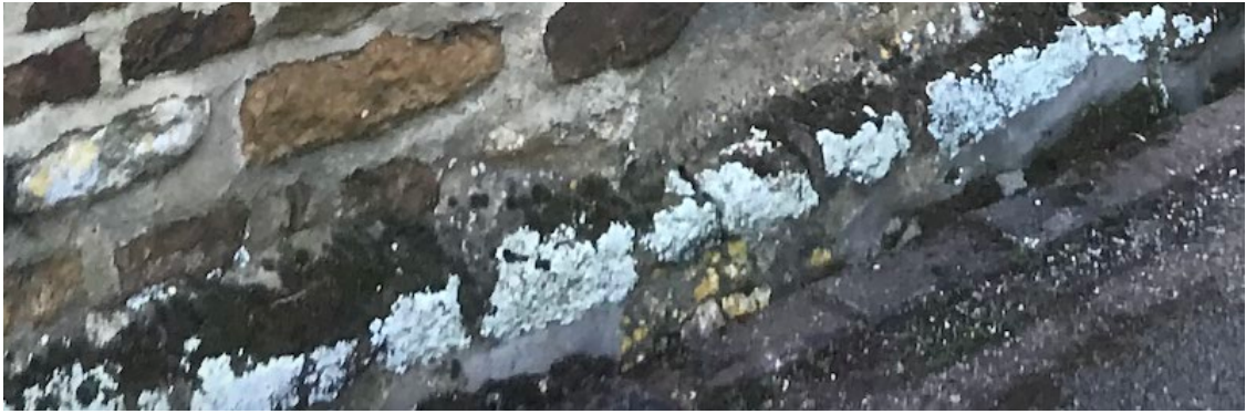
Fig. 12: Algae growing as a result of damp on the east elevation.
