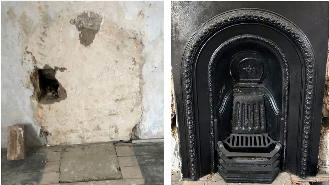
Fig.22: Existing blocked up fireplace in master bedroom showing small concrete slab within modern floorboards. Proposed replacement fireplace on the right.
