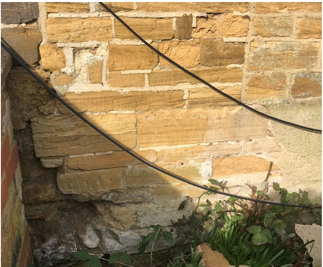
Fig. 13: Example of spalling stonework, failed pointing and deterioration of wall to south elevation. Note concrete skirt to right of photograph.
