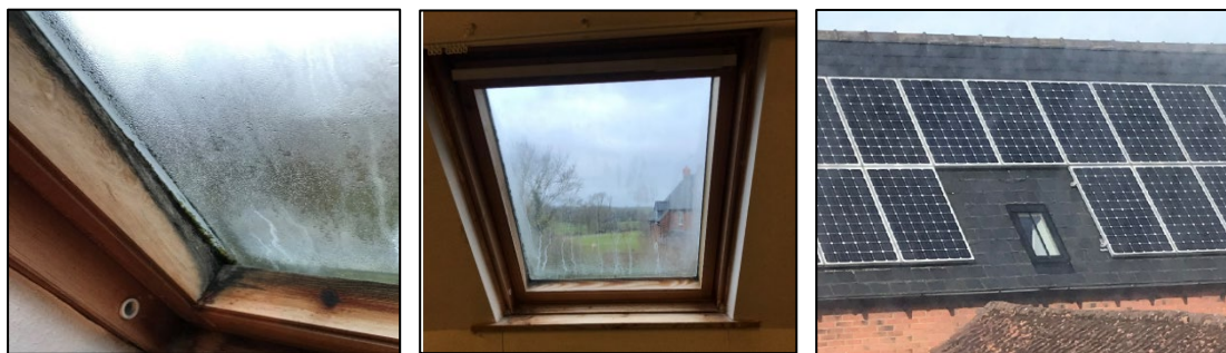
Fig. 15: Rooflights in attic showing signs of wear and degradation. Example of proposed rooflight on building opposite shown on the right.
