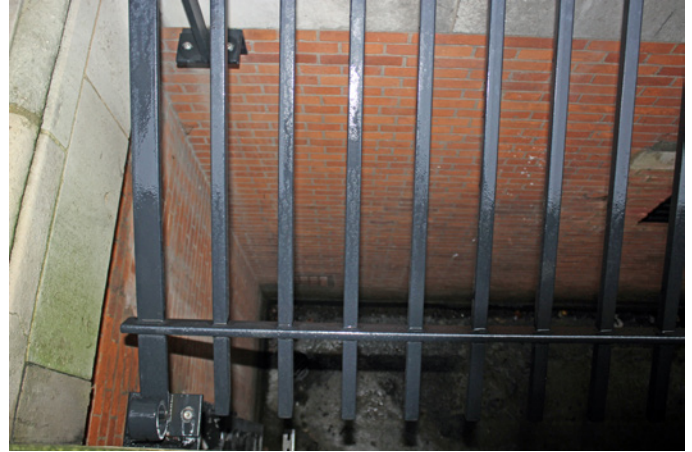
View looking into the lightwell (BM 34083-A) from street level on Great College Street
