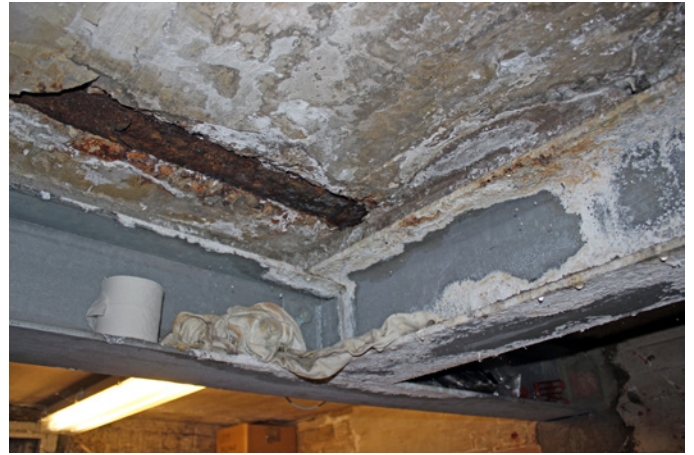
Corrosion of steel beams (expansion, lamination) in BM 63117 owing to water ingress
