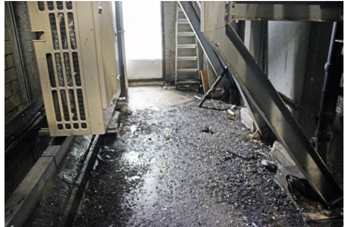
Floor showing surface water, dirt and pigeon guano
