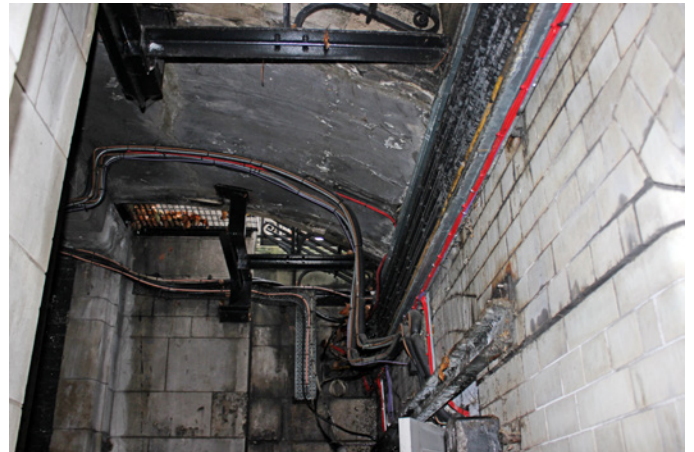
Cable trays with service wiring in the lightwell (BM 22850)
