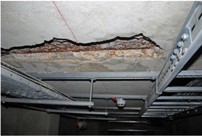
Corrosion of steel beams (expansion, lamination) owing to water ingress in BM 43077
