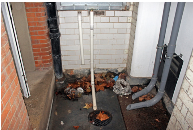
Concrete flooring at the south end of lightwell (B-29) and infilled opening between B-29 and B-34a
