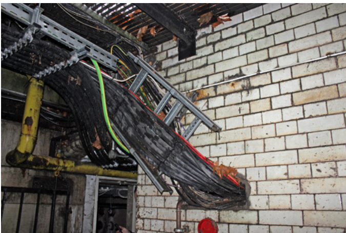
Cable trays and services interrupting wall fabric in BM 33113
