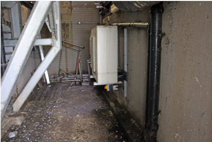
View looking west across BM 63108 showing a concrete floor, metal supports, pipework and service boxes
