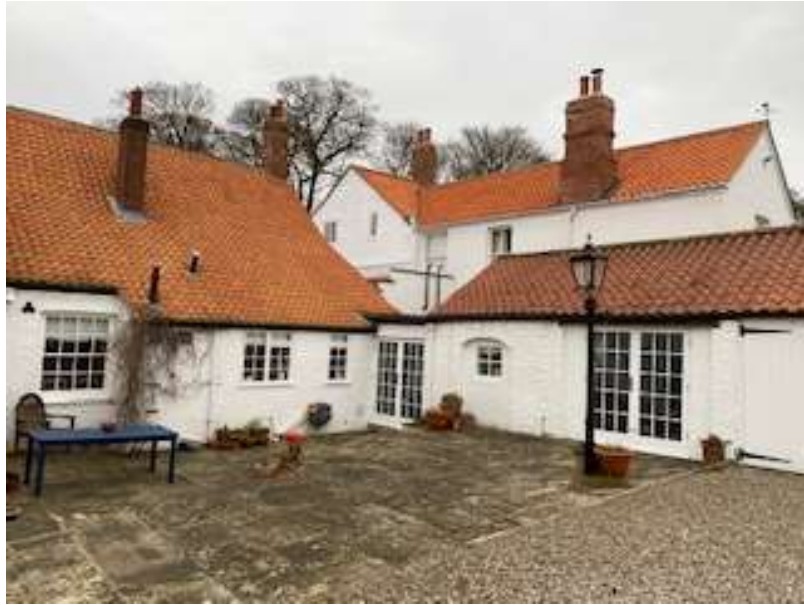
Photo 9 – rear elevation (to left) and single storey eastern wing (to right); neither set of existing French doors to be replaced
