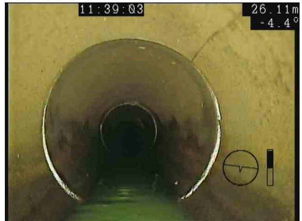
S18X_ec2350b0-acb3-445d-ae7-ac500e4601d8_20201106_154709_501.jpg, 00:02:08, 26.10 m Crack, longitudinal at 1 o'clock
