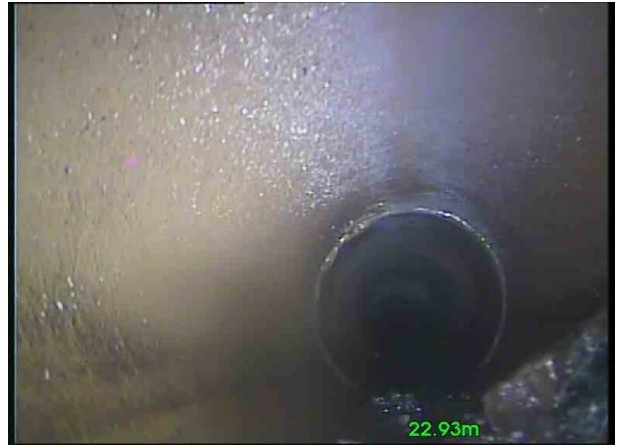
C16X_4a0ca8ad-960e-49ee-9f73-2d3afb1d0411_20201106_143019_940.jpg, 00:01:45, 22.98 m Settled deposits, coarse, 15% cross-sectional area loss
