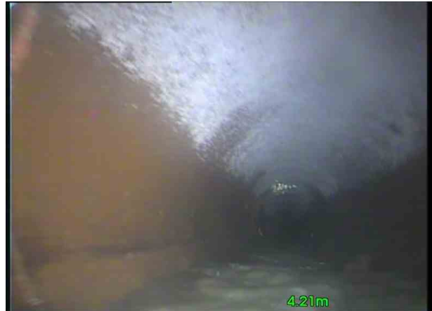
C16X_b5c9fa4-a52f-4b42-afac-de1a3b28e62c_20201106_130819_774.jpg, 00:00:33, 4.43 m Attached deposits, grease from 10 o'clock to 2 o'clock, 5% cross-sectional area loss, start
