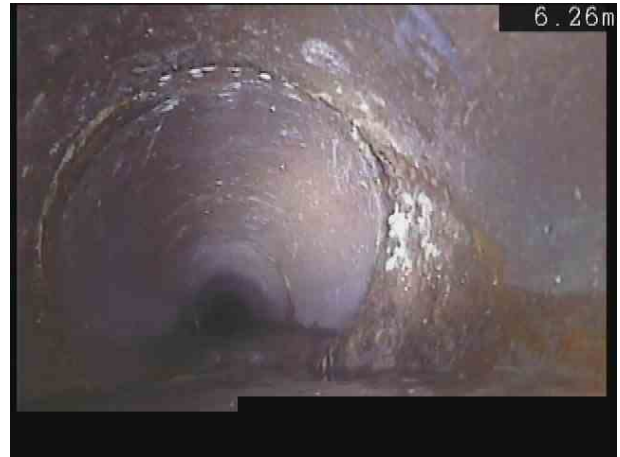
F1X_6a6c9ba3-5217-4132-a09d-0052345f46ce_20201110_105858_308.jpg, 00:00:45, 6.26 m Attached deposits, encrustation at joint from 2 o'clock to 6 o'clock, 15% cross-sectional area loss
