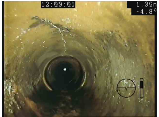
S19X_a582841d-2717-4ddd-89bc-d7c19de28dfe_20201110_111119_456.jpg, 00:00:23, 1.46 m Crack, longitudinal at 12 o'clock
