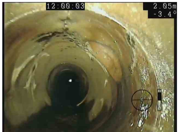
S19X_50f21c81-9d70-4eae-a7b6-a64339ea3148_20201110_111243_796.jpg, 00:00:26, 2.13 m Crack, circumferential from 9 o'clock to 12 o'clock
