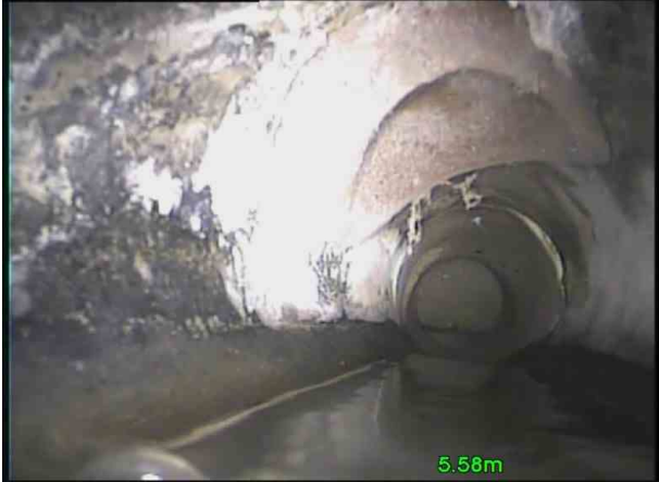
S17X_30903c72-e751-4bb4-97b8-41e7abac8dc8_20201106_125030_183.jpg, 00:00:38, 5.58 m Connection other than junction at 11 o'clock, diameter: 100mm
