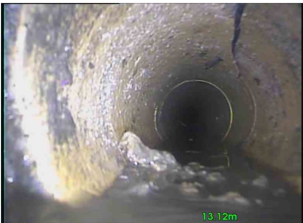
Branch X_47092d3a-271a-4efd-9c9e-2d220a38e735_20201109_1622 57_426.jpg, 00:01:38, 13.12 m Fracture, longitudinal at 1 o'clock
