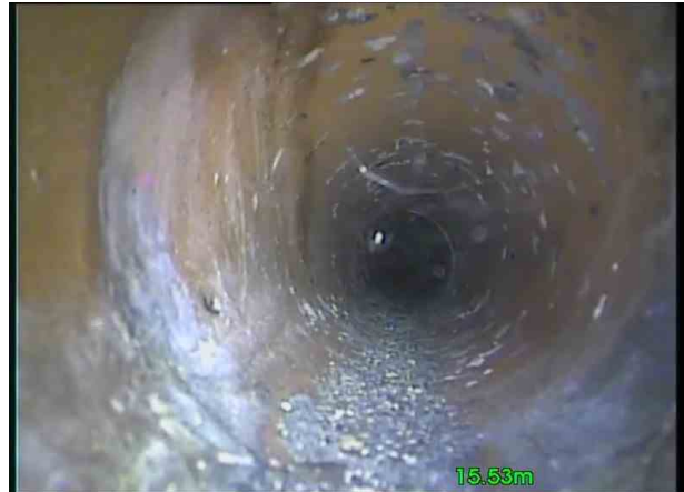
Branch 2X_365ecbab-3c0e-4c92-ba62-939207b87316_20201106_12 3955_239.jpg, 00:02:09, 15.53 m Settled deposits, coarse, 5% cross-sectional area loss
