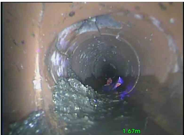
End O LineX_45453a69-058b-4e53-a29f-543728085864_20201105_162333_542.jpg, 00:00:14, 1.70 m Hole in drain or sewer at a joint from 11 o'clock to 12 o'clock
