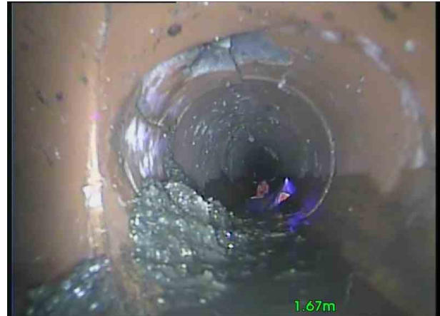
End O LineX_508b5ea3-3028-4401-aad6-392cc23e8313_20201105_162319_998.jpg, 00:00:14, 1.70 m Broken pipe at joint from 7 o'clock to 1 o'clock ,
