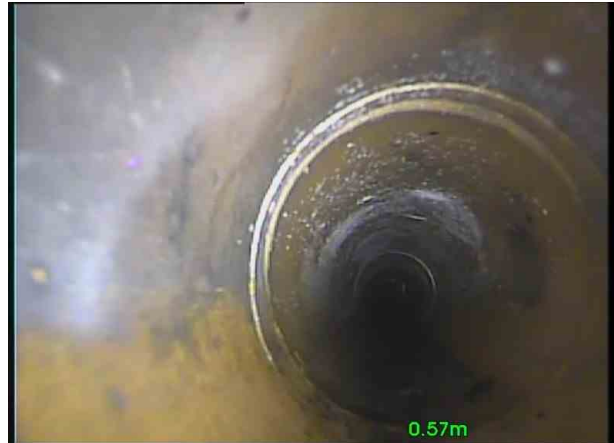
Branch 2X_f1a0522c-ab74-4fc0-ad5e-59ed6b5eab52_20201106_123 046_728.jpg, 00:00:12, 0.57 m Crack, circumferential at joint from 8 o'clock to 2 o'clock
