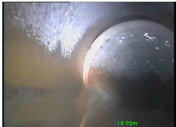
C16X_a0bf3a70-5b99-4b94-89e4-4b00dc26ef9f_20201106_142553_779.jpg, 00:01:22, 18.90 m Joint displaced, medium
