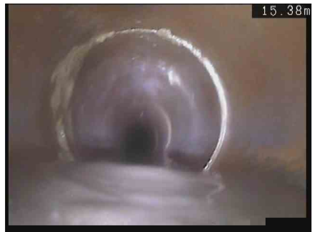
F1X_806fd6a6-3e72-43f3-bf46-e7725bc9fd1a_20201110_110438_127.jpg, 00:01:47, 15.40 m Attached deposits, encrustation at joint from 7 o'clock to 11 o'clock, 5% cross-sectional area loss
