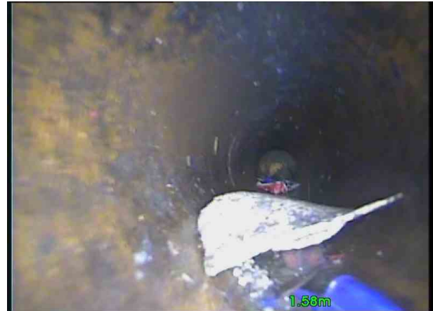
Branch 2X_36cd05c7-09a3-4c61-8e7a-1168bfbe9d40_20201105_163 513_104.jpg, 00:00:19, 1.58 m Settled deposits, other, 10% cross-sectional area loss, Debris
