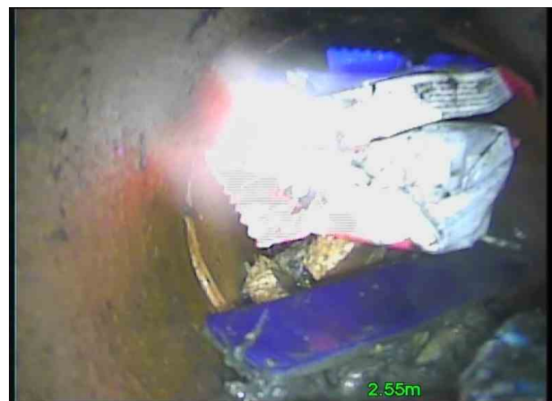
Branch 2X_88eebec7-9bc3-4ced-9545-07b14c0d7634_20201105_16 3556_805.jpg, 00:00:27, 2.55 m Settled deposits, other, 70% cross-sectional area loss, debris
