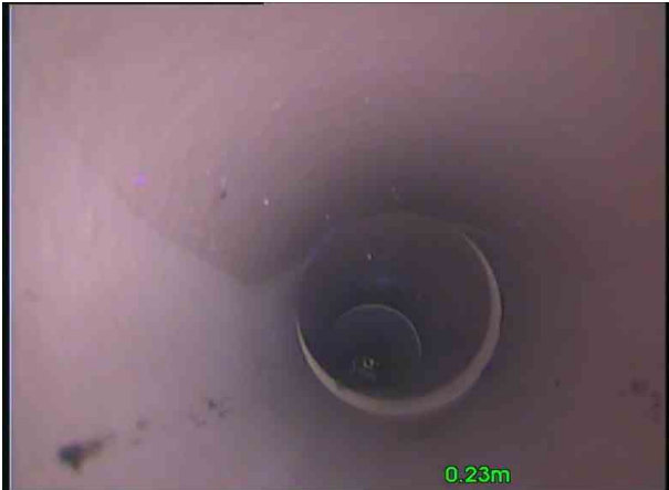
End O LineX_8bf572d9-1073-4fd8-8079-dd29252b1eb8_20201109_1 01306_920.jpg, 00:00:15, 0.23 m Crack, longitudinal at 2 o'clock
