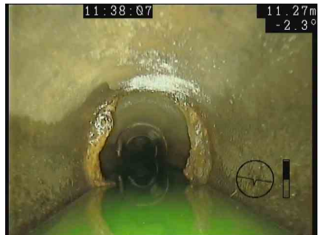
S18X_f6316c98-aa94-48ba-afd9-23bb97cd5314_20201106_153940_750.jpg, 00:01:12, 11.36 m Attached deposits, encrustation at joint from 8 o'clock to 4 o'clock, 20% cross-sectional area loss
