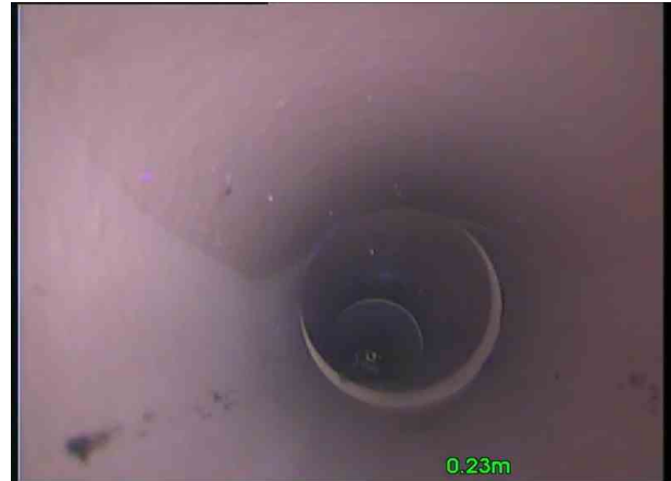
End O LineX_21e96b31-7273-4a78-96a6-e1f5af0f99a1_20201109_1 01245_296.jpg, 00:00:15, 0.23 m Crack, longitudinal at 10 o'clock
