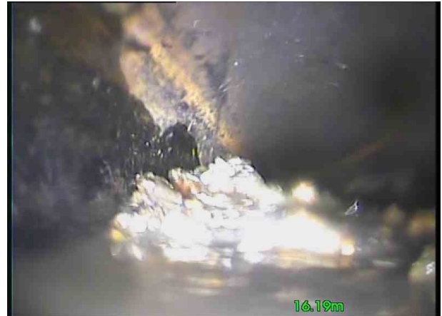
USX_5f3638b9-4dc3-41dc-b97a-df562f0a5bc9_20201106_120715_594.jpg, 00:01:50, 16.19 m Settled deposits, coarse, 30% cross-sectional area loss
