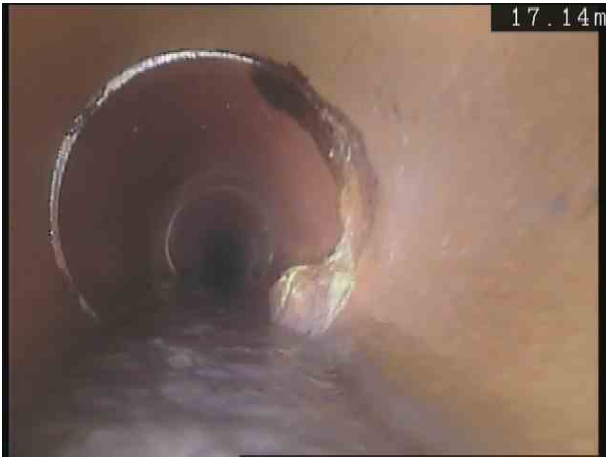
F1X_05b06084-92c3-4860-9708-6e39ca92a0bd_20201110_1 10503_382.jpg, 00:01:54, 17.25 m Attached deposits, encrustation at joint from 1 o'clock to 5 o'clock, 10% cross-sectional area loss
