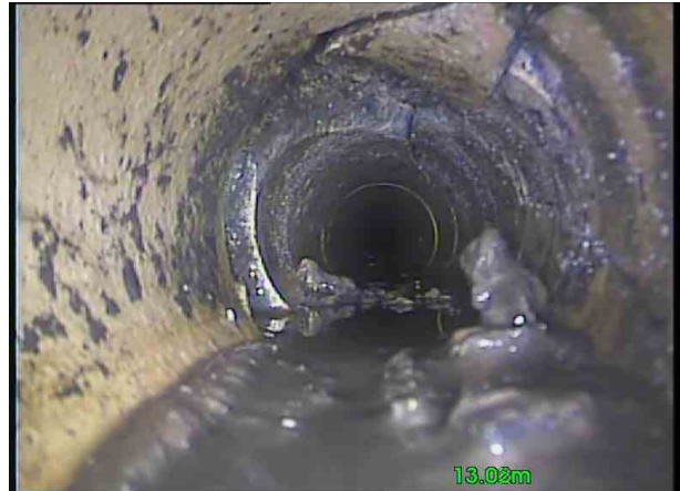
Branch X_327269f3-6905-4e12-9e0b-4040eaa99063_20201109_162 153_785.jpg, 00:01:32, 13.06 m Broken pipe from 11 o'clock to 4 o'clock
