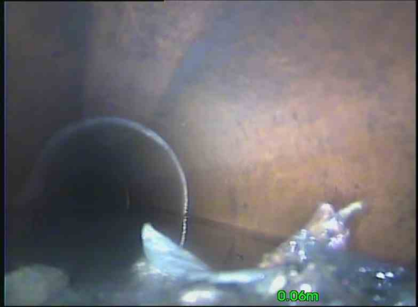
USX_eddd4ecc-7660-4389-938d-367d4dfd7d1e_20201105_1 55626_975.jpg, 00:00:08, 0.01 m Settled deposits, coarse, 15% cross-sectional area loss
