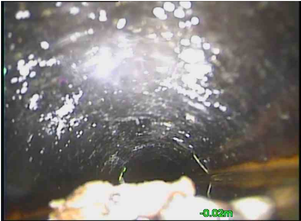
USX_6685c647-a3d7-4118-89c1-d5b9e974c8bc_20201105_1 64424_906.jpg, 00:00:08, 0.01 m Settled deposits, coarse, 15% cross-sectional area loss
