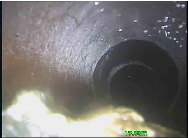
C16X_09b27c50-9367-4d7f-a19f-a535eadf9aae_20201106_142741_812.jpg, 00:01:27, 19.88 m Settled deposits, other, 15% cross-sectional area loss, Debris
