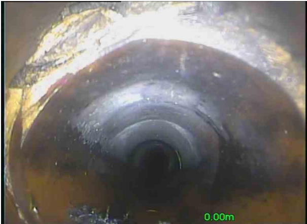
Branch 2X_73174870-0115-4315-bdd9-0c8b92c96928_20201106_12 2937_973.jpg, 00:00:07, 0.01 m Broken pipe at joint from 9 o'clock to 2 o'clock ,
