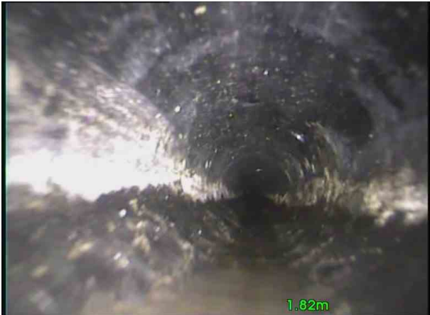
F41X_38ed019c-606b-45ac-8ff2-08375c96b1cd_20201110_093505_136.jpg, 00:00:14, 1.82 m Attached deposits, grease from 3 o'clock to 4 o'clock, 5% cross-sectional area loss, start
