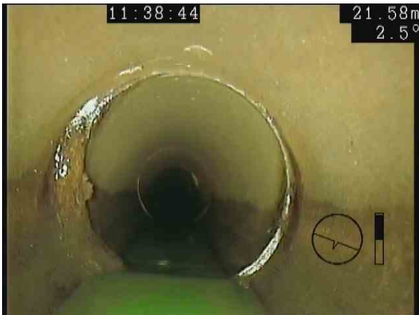
S18X_b4cb2a48-c6e3-4e24-b5f5-6e3029eb44ee_20201106_154627_087.jpg, 00:01:50, 21.67 m Attached deposits, encrustation at joint from 7 o'clock to 10 o'clock, 10% cross-sectional area loss
