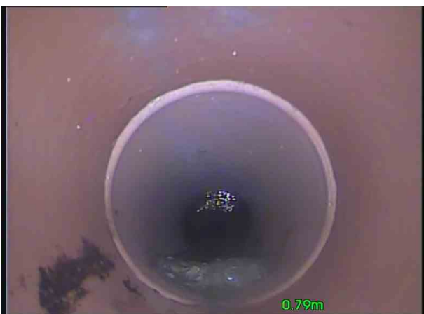
End O LineX_ccacb8fa-e7d4-4bdc-9e3b-3f455fe38f59_20201109_10 1405_971.jpg, 00:00:18, 0.80 m Settled deposits, fine, 10% cross-sectional area loss
