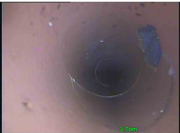
F28X_4930d5ab-3d21-47b6-8a81-1e0fb8b79434_20201106_161234_367.jpg, 00:00:33, 3.76 m Crack, circumferential from 3 o'clock to 8 o'clock
