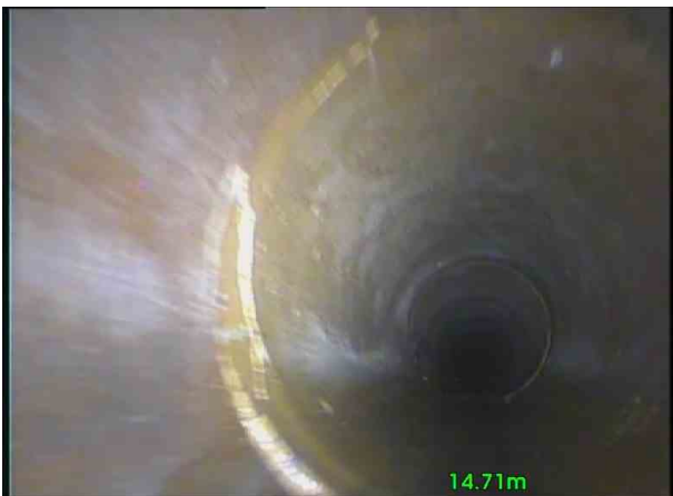
C9X_69511520-c31d-45ca-8d9e-f23c6cc42670_20201110_105248_896.jpg, 00:01:29, 14.70 m Crack, circumferential at joint from 8 o'clock to 11 o'clock
