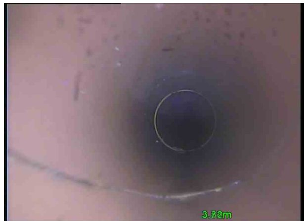
F28X_afa23ae4-bfbc-4ce7-974f-cb345fcd6a97_20201106_161301_053.jpg, 00:00:36, 3.82 m Fracture, circumferential from 3 o'clock to 8 o'clock
