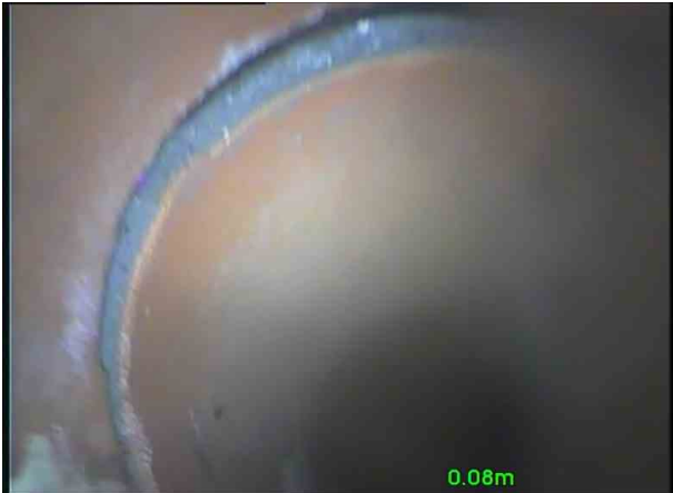
Branch 1X_3a75bf34-27d8-4ee7-93c5-f93aee379d16_20201106_162 422_024.jpg, 00:00:11, 0.10 m Open joint, medium
