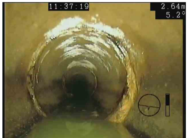
S18X_ef0b9b6f-b33f-4e0c-8aac-f53774f2120b_20201106_153552_219.jpg, 00:00:32, 2.72 m Attached deposits, encrustation at joint from 1 o'clock to 5 o'clock, 10% cross-sectional area loss
