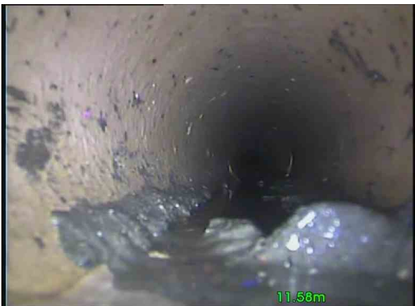
Branch X_34783183-e1db-459b-9ac4-04b6f3f610e5_20201109_1621 17_969.jpg, 00:01:23, 11.60 m Settled deposits, fine, 10% cross-sectional area loss
