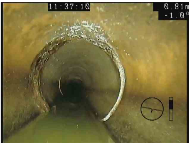
S18X_de190b00-621f-47ca-956d-04f5f0933d43_20201106_153522_380.jpg, 00:00:23, 0.88 m Attached deposits, encrustation at joint from 7 o'clock to 11 o'clock, 5% cross-sectional area loss
