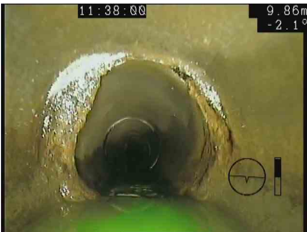
S18X_7d9cedae-6969-4f7c-9fb5-eeb3deca9ce9_20201106_153857_968.jpg, 00:01:05, 9.86 m Attached deposits, encrustation at joint from 7 o'clock to 4 o'clock, 20% cross-sectional area loss
