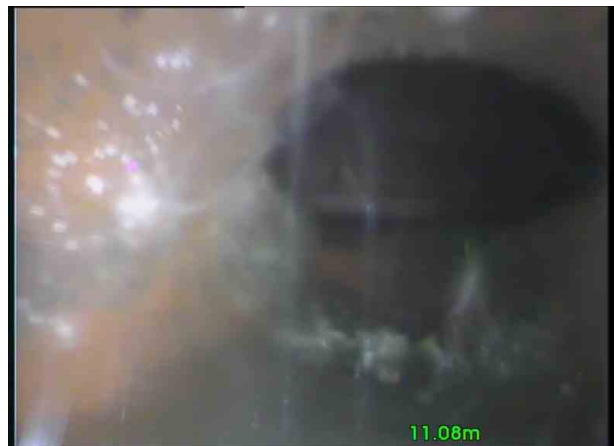
F40X_bee0ab22-7751-4006-976e-e8d67fdf2340_20201110_092432_044.jpg, 00:01:43, 11.08 m Settled deposits, fine, 5% cross-sectional area loss
