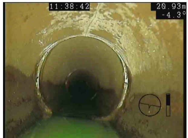
S18X_c6fce1ed-d7d8-4ed7-b6b7-ec7182af3358_20201106_154608_712.jpg, 00:01:47, 20.93 m Crack, longitudinal at 12 o'clock
