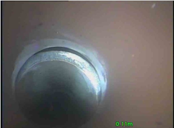
C22X_e022b4d2-b8ae-4c06-b650-ffd1859f2783_20201109_1 12516_904.jpg, 00:00:10, 0.10 m Joint displaced, large
