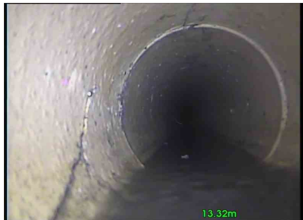
Branch X_48819294-8f4c-43f7-b0f2-0d3f8680d79c_20201109_16231 9_761.jpg, 00:01:40, 13.32 m Crack, circumferential from 7 o'clock to 9 o'clock
