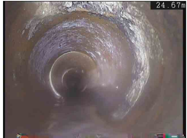
F4X_6191a1bc-4c17-4ad2-8297-9aab1560f653_20201109_165602_771.jpg, 00:02:18, 24.78 m Attached deposits, grease from 1 o'clock to 5 o'clock, 5% cross-sectional area loss
