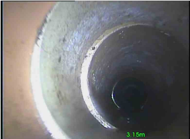
C9X_202de8bf-c946-4cd9-8a53-768cba2822e4_20201110_104335_375.jpg, 00:00:37, 3.15 m Joint displaced, medium
