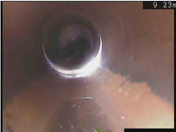
USX_548e278a-9421-410b-8288-2751742eba9c_20201109_152809_858.jpg, 00:01:00, 9.34 m Joint displaced, medium
