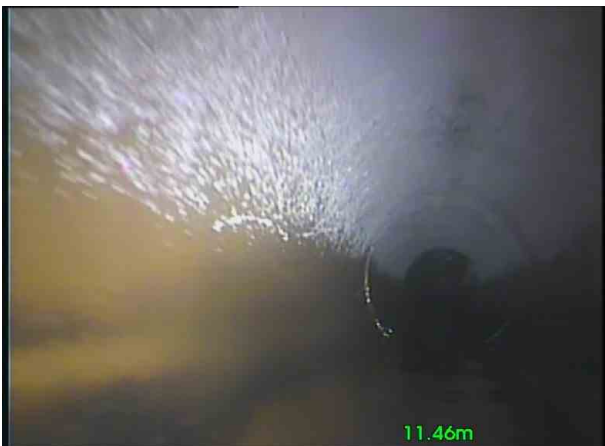
C16X_770be9cc-2366-4201-a38f-93e0c4affe35_20201106_131026_871.jpg, 00:00:58, 11.46 m Attached deposits, grease from 10 o'clock to 2 o'clock, 5% cross-sectional area loss
