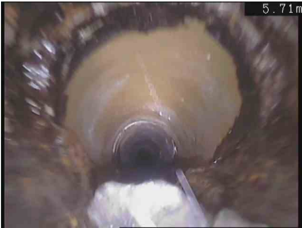
F1X_3e609a3d-5da2-461c-b477-8145ea55b999_20201110_105709_081.jpg, 00:00:37, 5.70 m Attached deposits, encrustation at joint from 12 o'clock to 12 o'clock, 25% cross-sectional area loss
