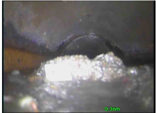
S42X_880e25ce-ba96-456c-ba13-4a50570136b5_20201105_163947_665.jpg, 00:00:08, 0.05 m Settled deposits, fine, 15% cross-sectional area loss
