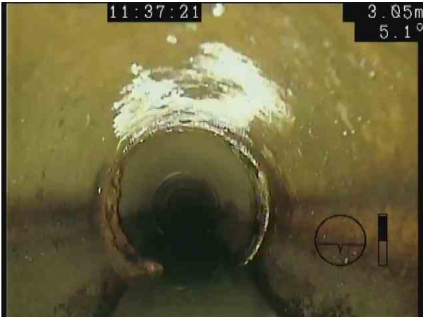
S18X_a922fc15-c22a-4cfa-a59b-7f10750e23f9_20201106_153613_417.jpg, 00:00:35, 3.20 m Attached deposits, encrustation at joint from 7 o'clock to 10 o'clock, 10% cross-sectional area loss
