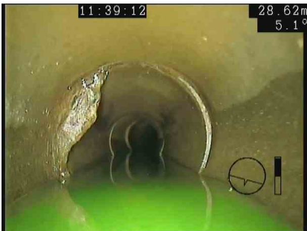
S18X_8242c4da-7854-46b3-a97c-adc9b7c6de9e_20201106_154743_651.jpg, 00:02:17, 28.62 m Attached deposits, encrustation at joint from 8 o'clock to 12 o'clock, 15% cross-sectional area loss
