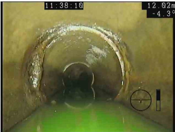
S18X_cd62f348-0ced-41b3-8e51-f44f8b37d90b_20201106_154120_416.jpg, 00:01:15, 12.02 m Attached deposits, encrustation at joint from 8 o'clock to 11 o'clock, 10% cross-sectional area loss
