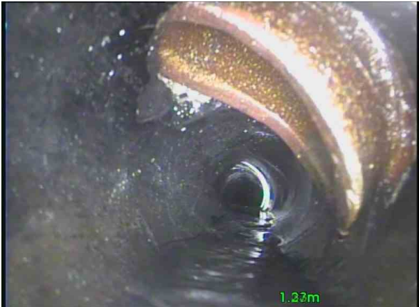
USX_c5e9e691-8fc6-474e-86e1-88aa62dba8e6_20201106_1 24640_341.jpg, 00:00:16, 1.33 m Connection defective, position incorrect at 2 o'clock, diameter: 100mm
