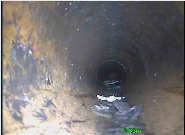
Branch 2X_a6bca09d-0fae-4926-938a-ae7fc9b9cde3_20201105_163 446_274.jpg, 00:00:15, 0.80 m Settled deposits, coarse, 5% cross-sectional area loss
