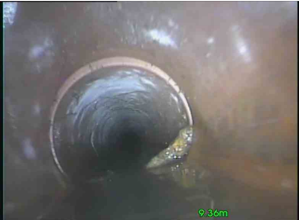
F40X_88b48801-c946-4518-9ade-fa31307cdf2a_20201110_092028_462.jpg, 00:00:44, 9.36 m Attached deposits, encrustation at joint from 3 o'clock to 7 o'clock, 20% cross-sectional area loss
