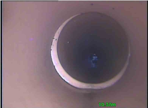
F28X_fb5ef1a3-a45c-44d0-8bd2-b5880a3a00ba_20201106_1 61347_387.jpg, 00:01:00, 10.55 m Joint displaced, medium
