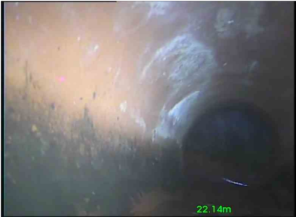
F20X_93474d2a-d8f9-4b89-9b81-7183b8db47b1_20201109_111728_977.jpg, 00:01:14, 22.15 m Settled deposits, hard or compacted, 10% cross-sectional area loss
