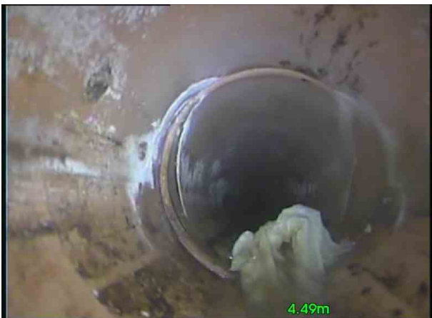
End O LineX_cbb0c64e-17da-49d4-bf4e-dc356e92833c_20201106_160214_546.jpg, 00:00:35, 4.50 m Settled deposits, other, 10% cross-sectional area loss, Wipes
