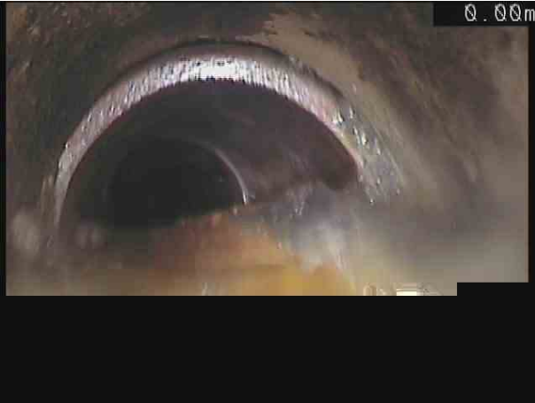
F6X_36db4c7e-f239-4a9e-ba2a-911e01c3538a_20201109_16 2818_233.jpg, 00:00:18, 0.05 m Joint displaced, medium
