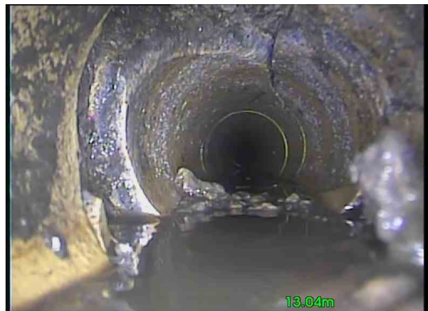
Branch X_6f930d41-94af-4faa-8532-c03527b4e997_20201109_16223 9_091.jpg, 00:01:37, 13.05 m Hole in drain or sewer from 7 o'clock to 12 o'clock
