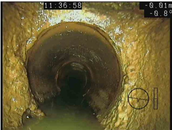
S18X_4f4e42f7-d649-41b4-afad-11ae3afd3798_20201106_153415_880.jpg, 00:00:12, 0.01 m Attached deposits, encrustation from 7 o'clock to 5 o'clock, 15% cross-sectional area loss
