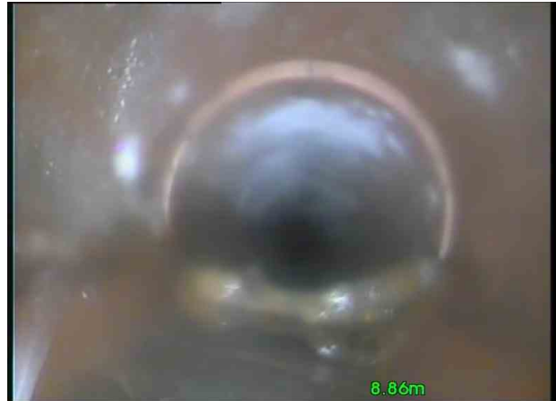
F40X_3bd4db38-9d64-4bea-a178-5b7277d45a9d_20201110_092204_494.jpg, 00:00:44, 9.36 m Attached deposits, encrustation at joint from 3 o'clock to 7 o'clock, 20% cross-sectional area loss
