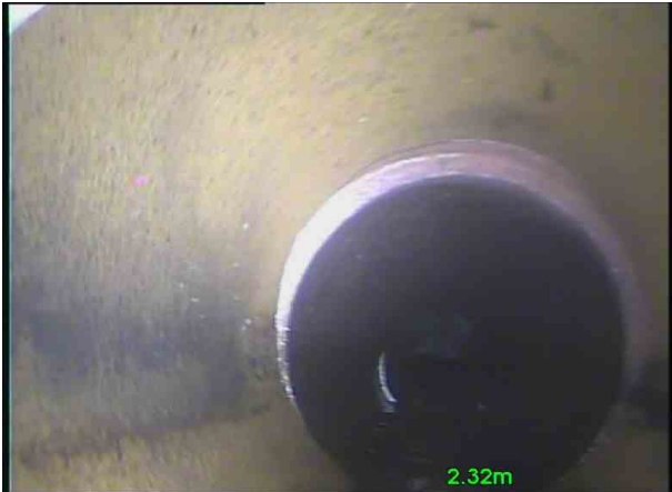
C18X_2b4e6725-5ec7-4fe6-b17b-e7f27026f290_20201106_130629_316.jpg, 00:00:18, 2.30 m Joint displaced, medium
