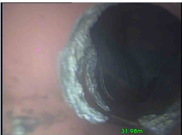
C22X_f3fcc9f7-461d-4e92-92ea-bebe98ced525_20201109_1 12953_401.jpg, 00:01:56, 31.98 m Attached deposits, grease at joint from 7 o'clock to 5 o'clock, 10% cross-sectional area loss
