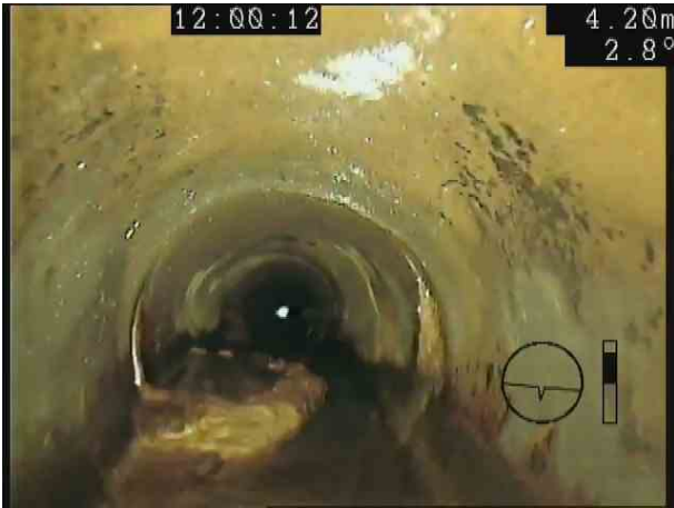
S19X_4a93d849-7f6e-4131-852a-cdd98a75d6d2_20201110_111358_217.jpg, 00:00:35, 4.33 m Settled deposits, hard or compacted, 25% cross-sectional area loss
