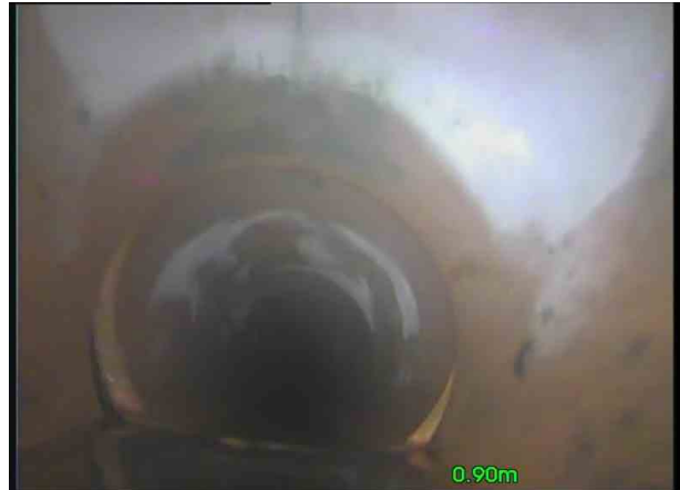
C22X_2cfd079-b21c-420a-b1b0-7a9959477650_20201109_1 12618_757.jpg, 00:00:13, 0.90 m Joint displaced, medium
