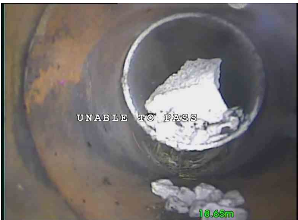
Branch 2X_7eabd447-ee63-4cae-99c3-d46371f48a00_20201106_124 208_870.jpg, 00:02:39, 18.65 m Obstacles, external pipe or cable from 12 o'clock to 12 o'clock, 50% cross-sectional area loss, Smaller pipe in drain, Debris at the entrance
