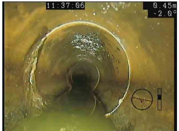
S18X_7cb84242-ac10-4d80-a729-1f478ad9e85a_20201106_153445_446.jpg, 00:00:20, 0.50 m Attached deposits, encrustation at joint from 7 o'clock to 11 o'clock, 5% cross-sectional area loss
