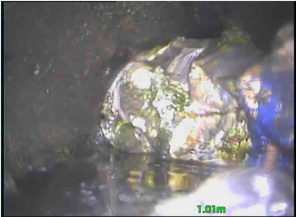
S36X_e1b14cac-e86d-4bc9-b260-0c5c9f46dc73_20201106_1 22359_538.jpg, 00:00:15, 1.00 m Settled deposits, other, 85% cross-sectional area loss, Debris
