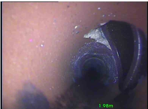
Branch 2X_dce7c60e-3e78-4d2a-ad8a-b66cf6cfe55f_20201106_1231 30_117.jpg, 00:00:21, 2.00 m Connection defective, position incorrect at 2 o'clock, diameter: 100mm
