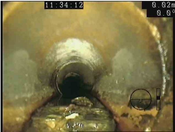
USX_d8e434eb-1a70-44c0-8233-0b88441ca576_20201106_152412_326.jpg, 00:00:18, 0.05 m Settled deposits, hard or compacted, 15% cross-sectional area loss
