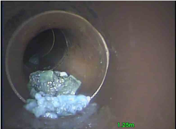
USX_348c6604-30e1-48ee-bb8d-109f76e78d33_20201110_095931_892.jpg, 00:00:53, 1.25 m Settled deposits, other, 25% cross-sectional area loss, Rock
