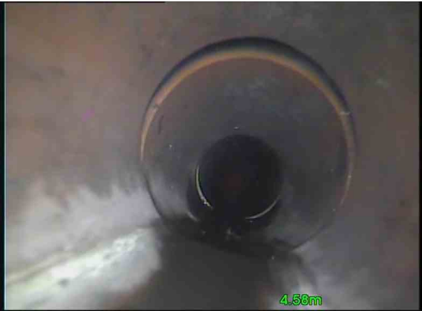
F39X_fca828d8-2945-469c-b869-a62eabfb5a2e_20201110_092727_827.jpg, 00:00:24, 4.60 m Joint displaced, medium
