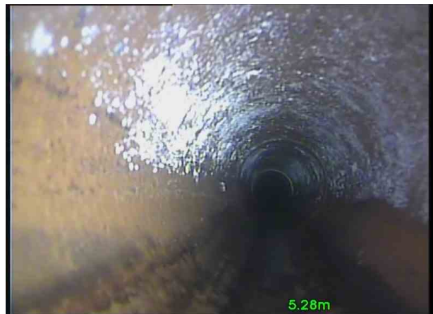
Branch 2X_2ac7df6a-352c-4816-a123-468eeb04a987_20201106_123 520_568.jpg, 00:00:49, 5.28 m Attached deposits, grease from 9 o'clock to 3 o'clock, 5% cross-sectional area loss
