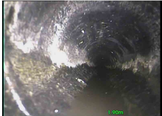
F41X_7d235afc-c23d-4967-929f-0e520c81505b_20201110_093437_363.jpg, 00:00:14, 1.90 m Attached deposits, grease from 9 o'clock to 10 o'clock, 5% cross-sectional area loss, start
