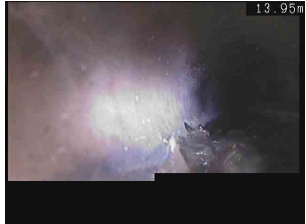
USX_1d8947bd-7930-483c-883d-98f08637c592_20201109_152843_028.jpg, 00:01:19, 14.06 m Settled deposits, coarse, 15% cross-sectional area loss
