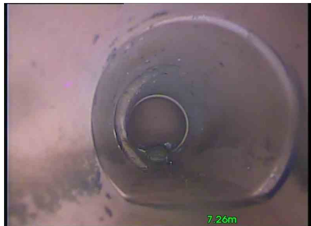
End O LineX_7f7e4528-b4be-4f11-8280-db7c87e05b26_20201106_160351_269.jpg, 00:00:53, 7.30 m Open joint, medium
