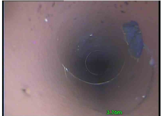
F28X_6381d4ca-e373-4aa9-98b2-bce59e1edac9_20201106_161212_176.jpg, 00:00:33, 3.76 m Hole in drain or sewer from 1 o'clock to 3 o'clock
