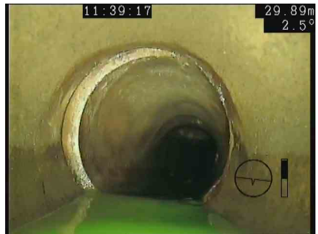
S18X_818ec3eb-e12a-4c5d-a018-6fb7a24fb8a0_20201106_154759_826.jpg, 00:02:22, 29.97 m Joint displaced, medium
