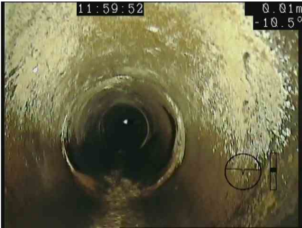
S19X_a7df55b7-a0bf-4cd2-98cc-bbabe69b83d3_20201110_11208_279.jpg, 00:00:14, 0.30 m Attached deposits, encrustation at joint from 3 o'clock to 7 o'clock, 5% cross-sectional area loss
