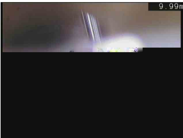
F1X_c3d74d90-15dd-4643-8721-da30fc64ea32_20201110_110247_838.jpg, 00:01:18, 10.10 m Attached deposits, encrustation at joint from 1 o'clock to 5 o'clock, 10% cross-sectional area loss
