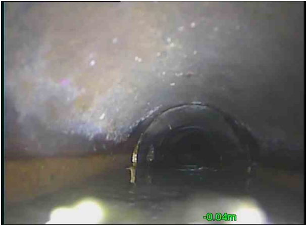
S42X_27c6418a-1244-4c36-829a-6bba5c22d076_20201105_163758_758.jpg, 00:00:08, 0.05 m Settled deposits, fine, 15% cross-sectional area loss
