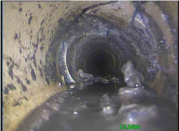
Branch X_2e8ff3b5-9aed-4fae-8d18-226792160f50_20201109_16221 5_021.jpg, 00:01:32, 13.06 m Deformed drain or sewer, 5%
