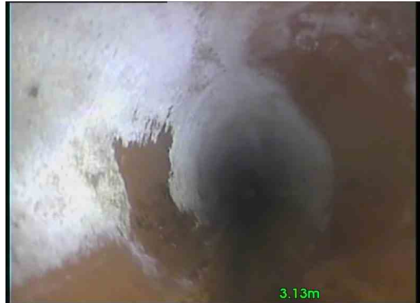
End O LineX_128482e2-076d-411b-9ac6-ab903f453058_20201106_160149_706.jpg, 00:00:30, 3.13 m Attached deposits, grease from 8 o'clock to 4 o'clock, 5% cross-sectional area loss
