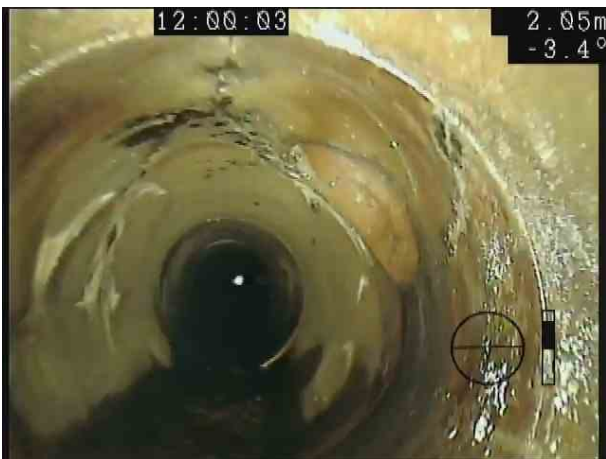
S19X_e79285c3-b780-4a96-bc4c-98708fa75e17_20201110_11301_659.jpg, 00:00:26, 2.13 m Crack, circumferential from 12 o'clock to 1 o'clock
