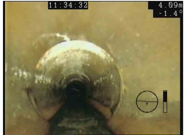
USX_1ae78ce8-9547-41b5-9e37-a0fb2de6d519_20201106_152845_412.jpg, 00:00:37, 4.10 m Crack, circumferential at joint from 11 o'clock to 12 o'clock
