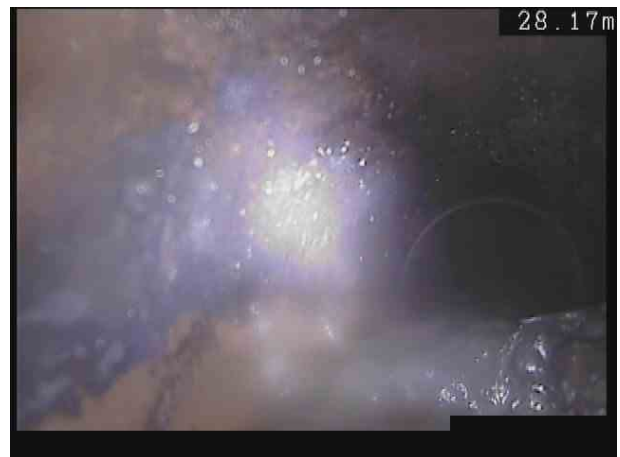
USX_4a6420a9-d279-4231-94e9-a1013f10efc7_20201109_153457_870.jpg, 00:03:38, 28.17 m Settled deposits, other, 30% cross-sectional area loss, unknown
