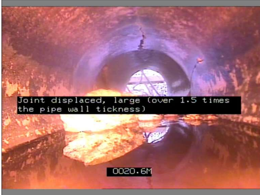
Photo: 11_5A, MPEG #: 220321_1, 00:02:41 20.6m, Joint displaced, large (over 1.5 times the pipe wall tickness)
