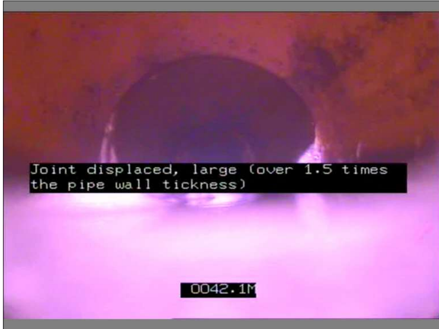
Photo: 10_2A, MPEG #: 220321_1, 00:05:22 42.1m, Joint displaced, large (over 1.5 times the pipe wall tickness)
