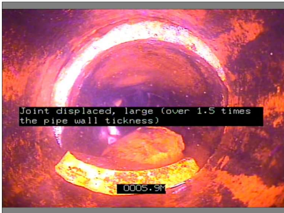
Photo: 2_4A, MPEG #: 220321_1, 00:01:06 5.9m, Joint displaced, large (over 1.5 times the pipe wall thickness)
