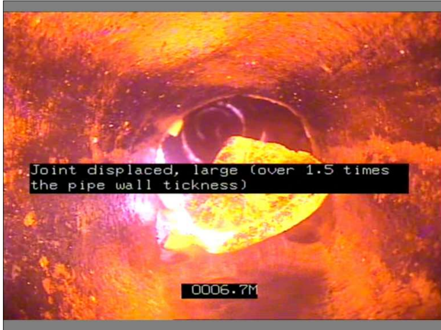
Photo: 2_6A, MPEG #: 220321_1, 00:01:22 6.7m, Joint displaced, large (over 1.5 times the pipe wall tickness)
