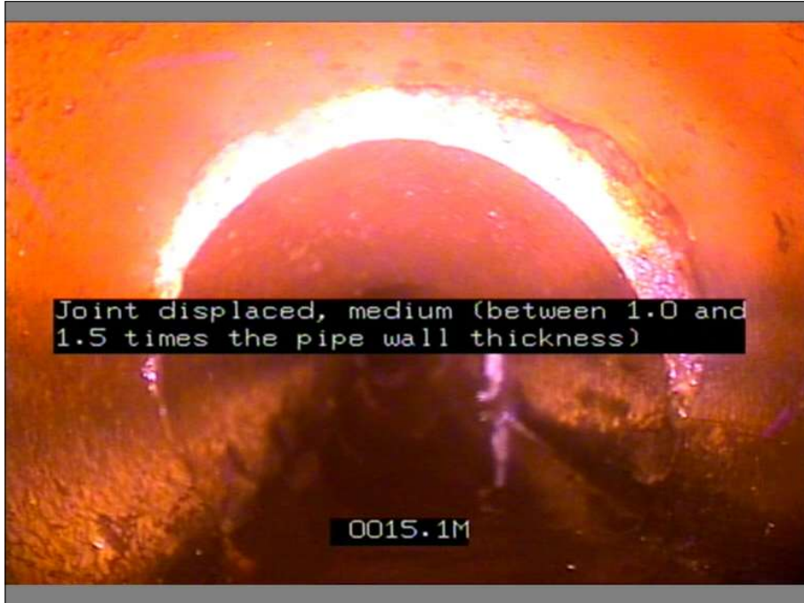
Photo: 3_4A, MPEG #: 220321_1, 00:02:04 15.1m, Joint displaced, medium (between 1.0 and 1.5 times the pipe wall thickness)
