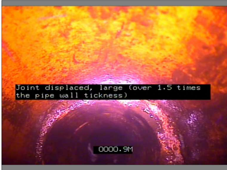
Photo: 1_2A, MPEG #: 220321_1, 00:00:50 0.9m, Joint displaced, large (over 1.5 times the pipe wall tickness)
