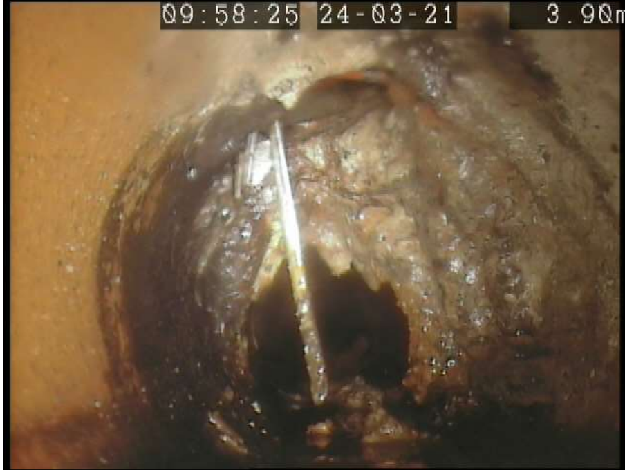
Photo: 21_2A, MPEG #: 220321_1, 00:00:28 3.9m, Encrustation, heavy, from 12 to 12 o'clock, 50% cross-sectional area loss
