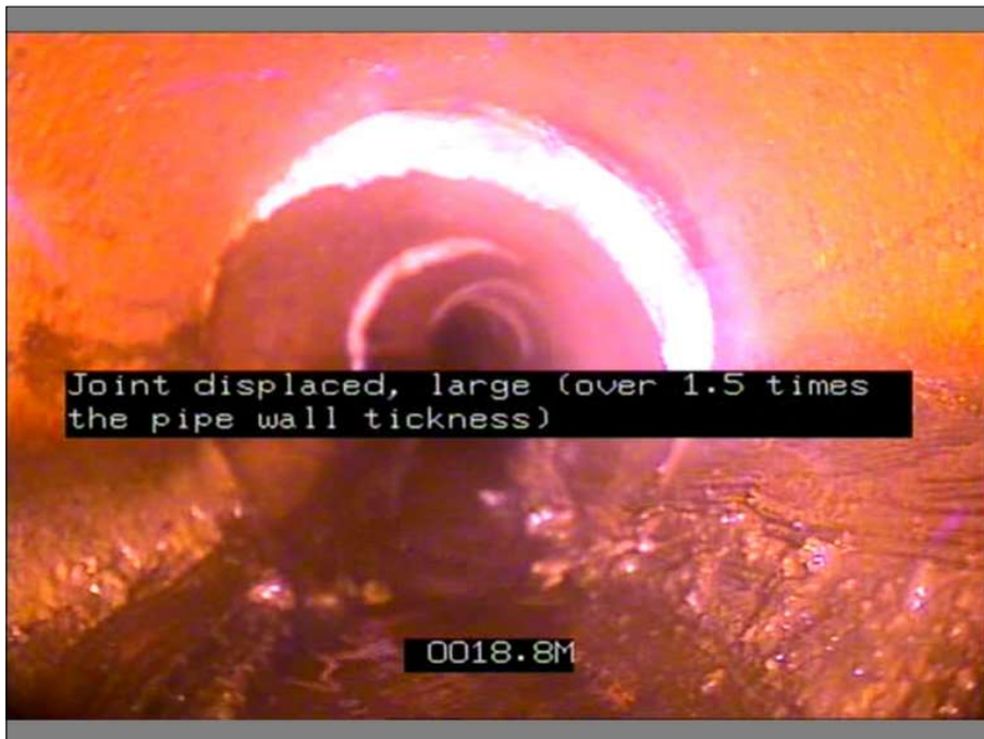
Photo: 3_5A, MPEG #: 220321_1, 00:02:27 18.8m, Joint displaced, large (over 1.5 times the pipe wall thickness)
