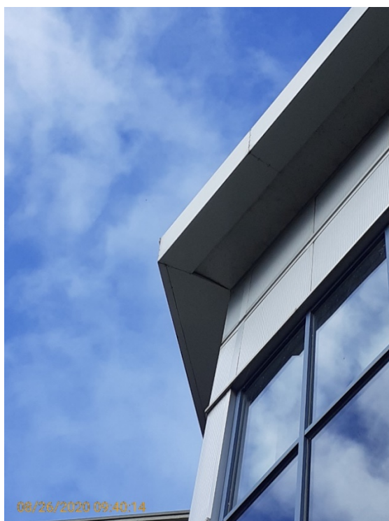
Figure 18: Small gap in the roof panels under the eaves of the overhang at the southern entrance to the building. Low to moderate potential (to be confirmed after further surveys).
