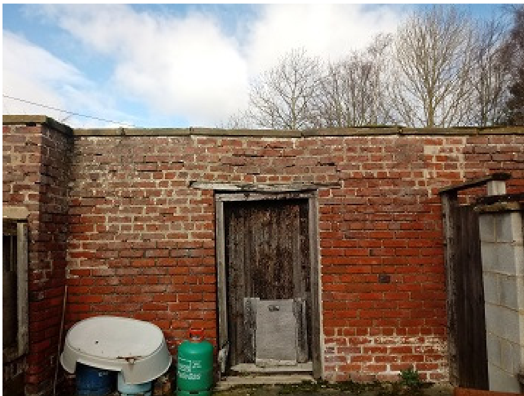
Plate11. Example of holes in the external wall and gaps surrounding door frame
