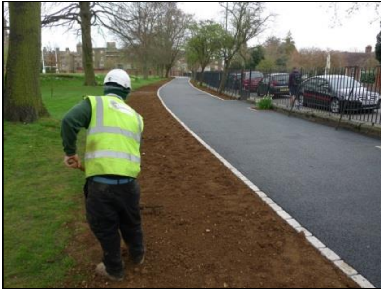
Fig 8 – All 'making good' topsoil will be BS3882 compliant and raked out by hand to no greater depth than 100mm
