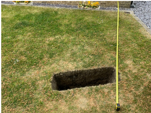
Figure 4; trench dug to investigate tree roots at point of proposed extension closest to street tree.
