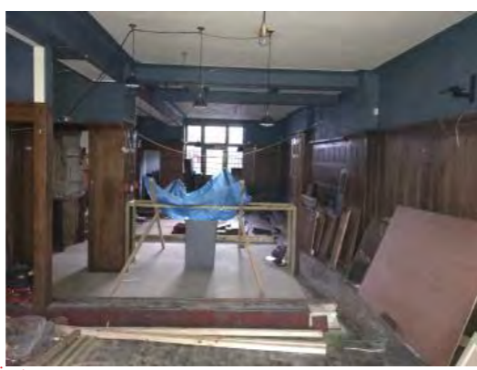
Intact; bar missing
