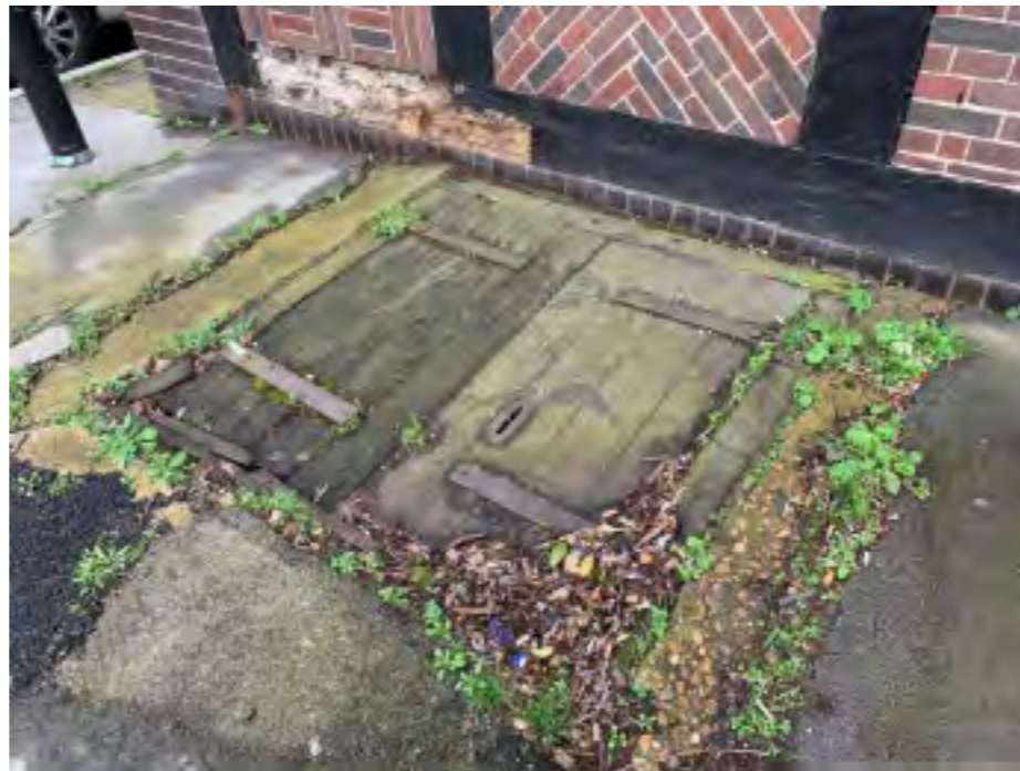
External trap doors to cellar requiring repair.
