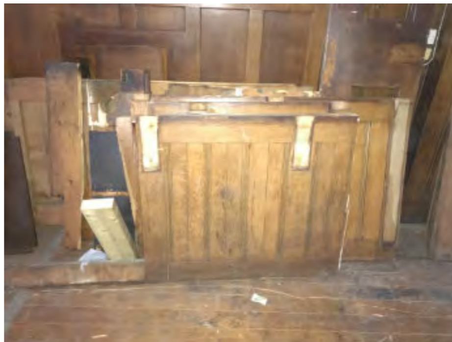
Surviving panels to bar servery front.
