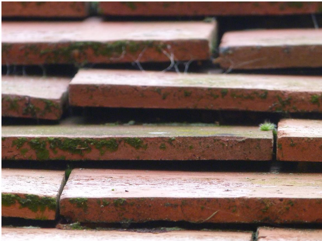
Photograph No: 2 - Gaps between tiles present potential roosting features for crevice dwelling bats
