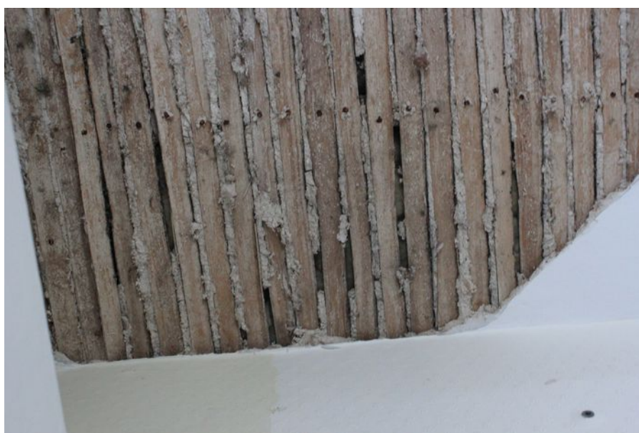
Plate 7: Earlier laths and plaster seen beneath the modern plaster board, hall ceiling first floor, facing west
