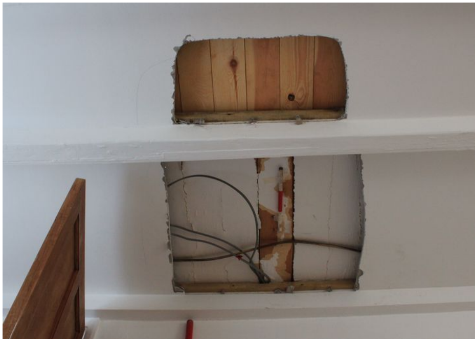
Plate 2: Area of ceiling to be impacted by the insertion of the spiral stair with plasterboard removed showing timber and floor boards to be modern, looking south
