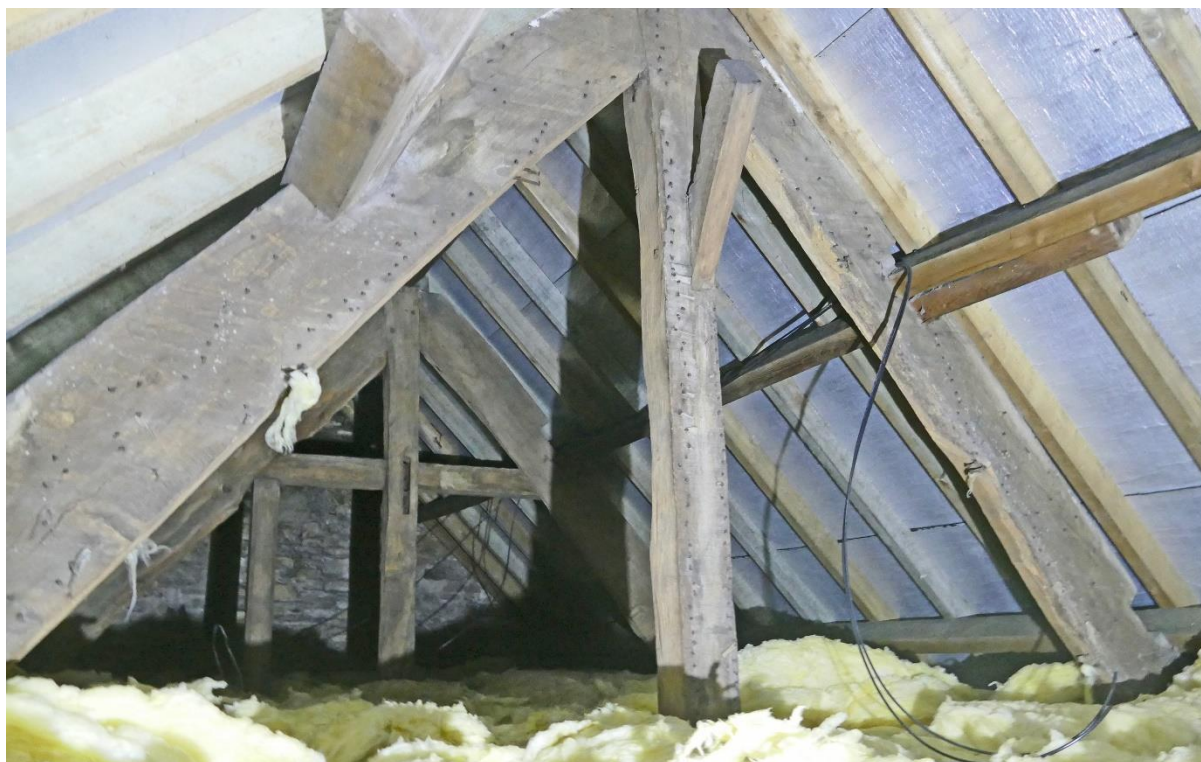
The roof looking south-west, showing the two king-post trusses; note nails in nearer truss, associated with lath infill.
