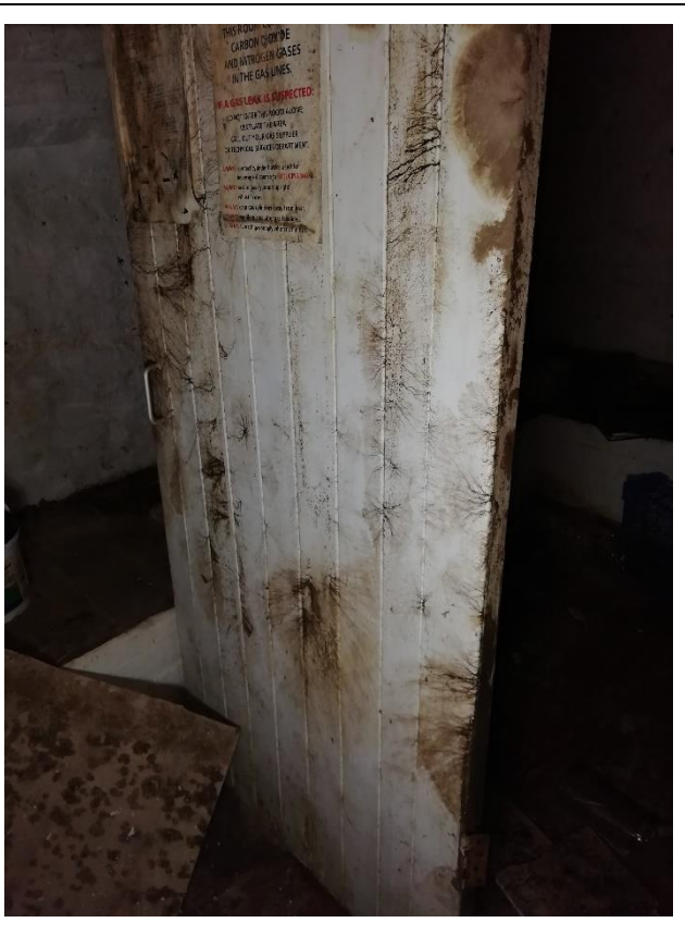
Evidence of dry rot fungus.
