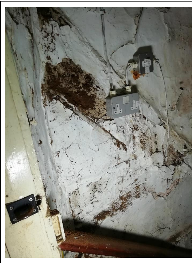
Timber frame to cellar stairs with rot.
