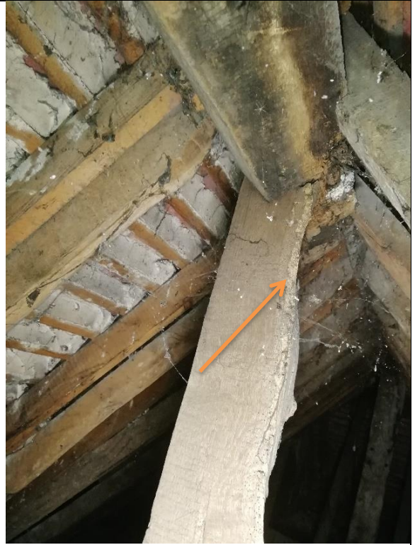
Evidence of beetle infestation and rot.
