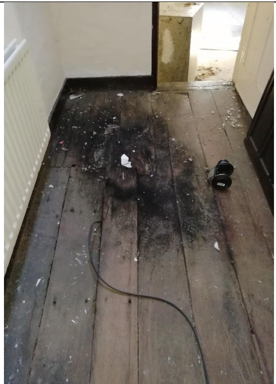
Damage to floor from open skylight.
