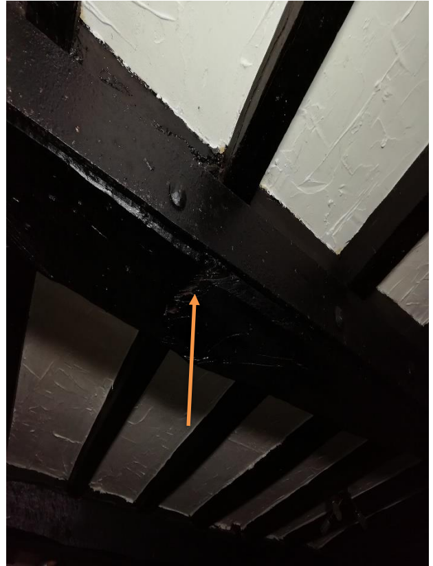
Fracture and steel plate repair to beam.
