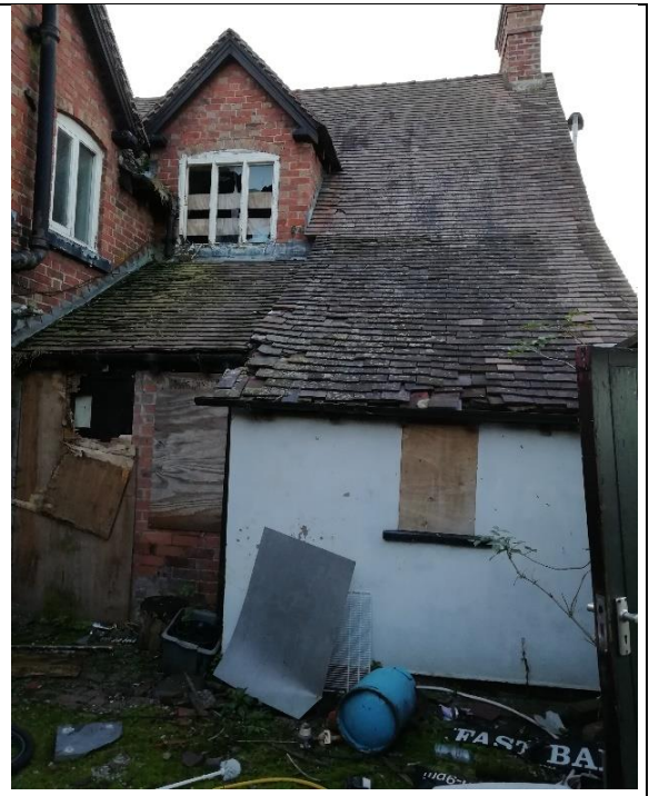
Repairs to roof and gutters required.
