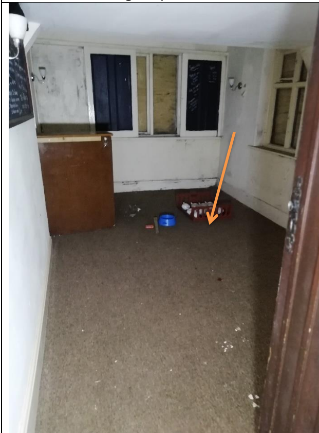
Area above cellar, starting to fail.
