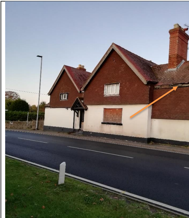
Gutter fascia damage requires attention.
