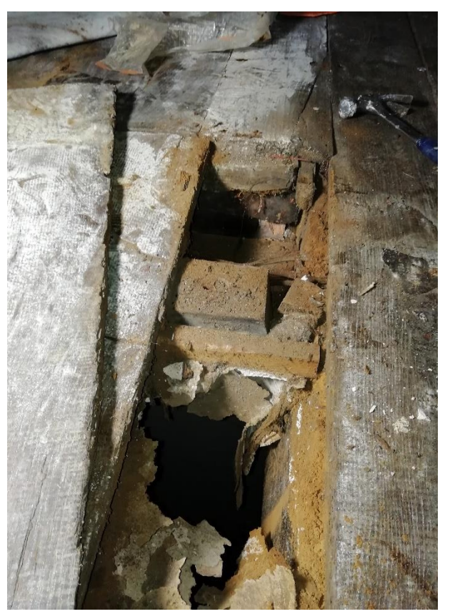
Oak floorboard lifted above deflected beam
