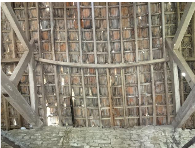
Barn Deflected Purlin
