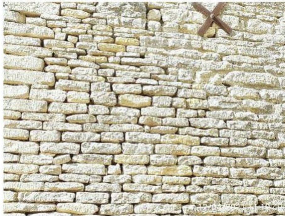
Figure 19: Further example of holes in wall of B2
