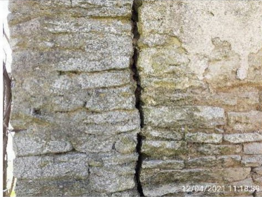
Figure 18: Example of large cracks/ crevices in stonework in B2
