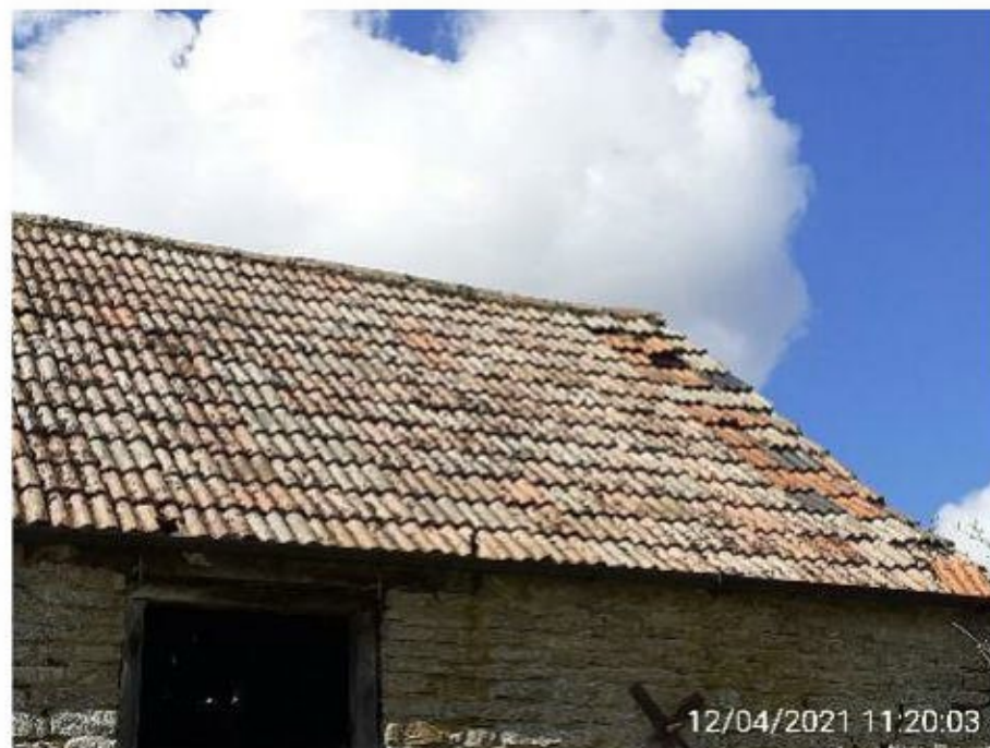
Figure 20: Example of loose/missing roof tiles on B2
