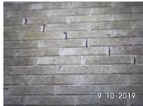
Right Side Gable Elevation – Stepped Cracks
