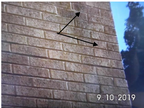
Side Elevation – Stepped Masonry Cracks
