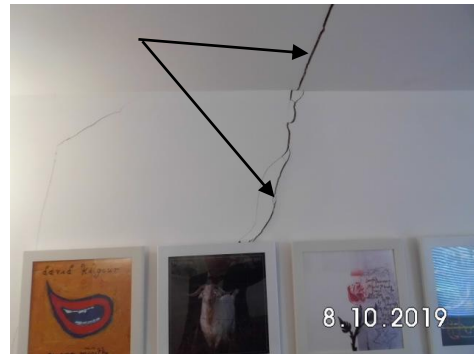
Flat 4 Lounge – Wall/Ceiling Crack
