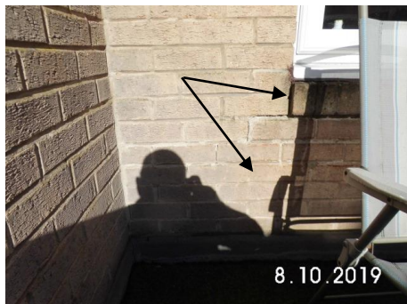
Flat 4 Side Wall – Stepped Cracks
