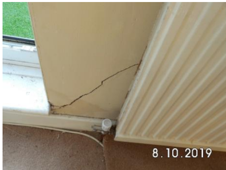
Flat 10 Lounge – Diagonal Crack at uPVC Door
