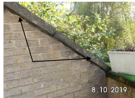
Flat 10 Balcony – Displaced Copings
