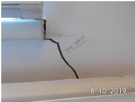
Flat 4 Lounge – Diagonal Crack to Sill
