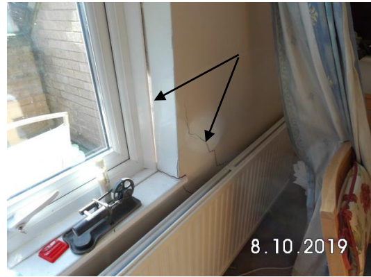
Flat 10 – Diagonal Crack to Lounge
