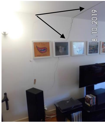
Flat 4 – Vertical Crack in Lounge
