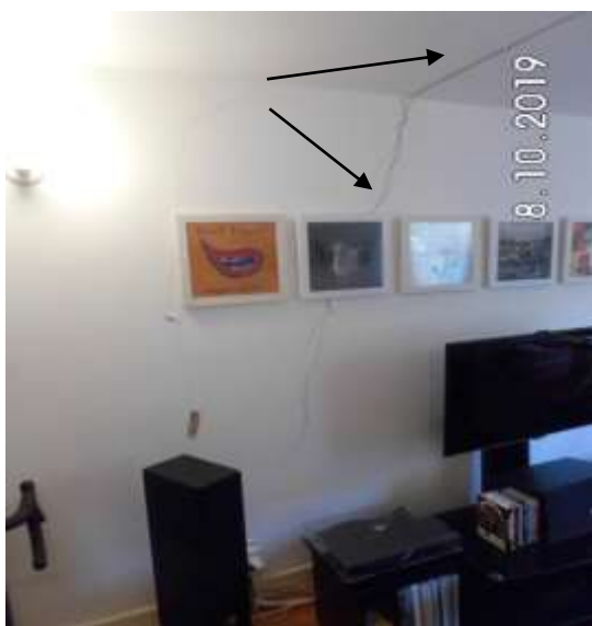
Flat 4 – Vertical Crack in Lounge
