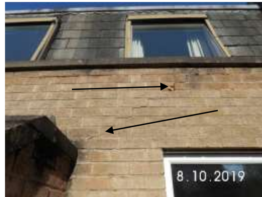
Flat 10 – Stepped Cracking
