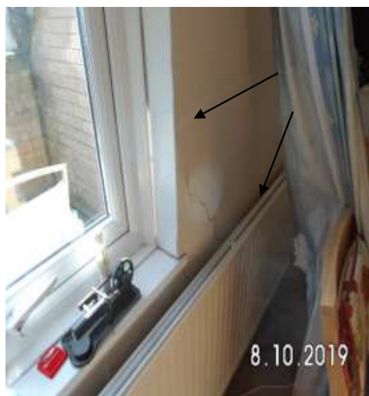
Flat 10 – Diagonal Crack to Lounge
