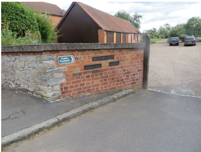
Figure 8 – Boundary wall at the entrance to be altered, with timber clad front elevation of the outbuilding
