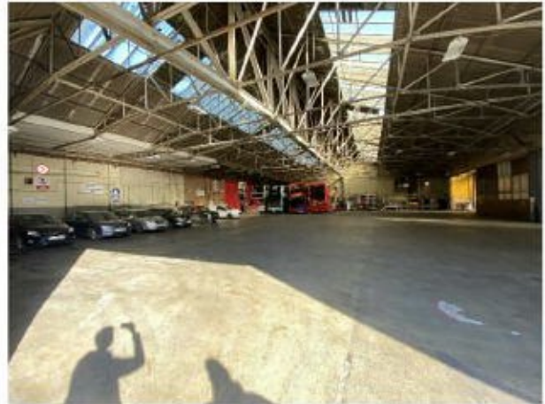
Inside the main workshop area
