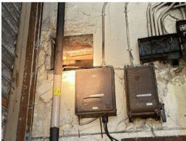
Hole into cavity wall inside workshop
