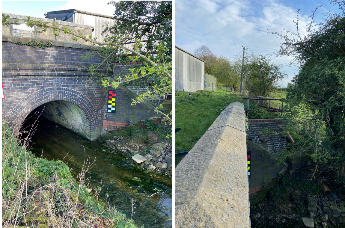
Photographs showing the substantial nature of the culvert and the significant levels difference between the Beck and the yard
