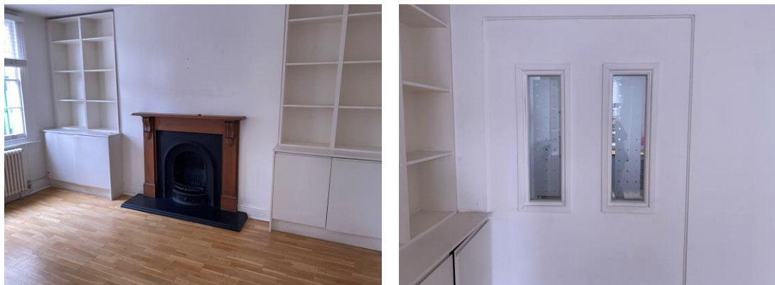
Figures 12 and 13: Views of the second floor showing the front room with chimney breast and fire surround (left) and infill panel within the spine wall (right)
