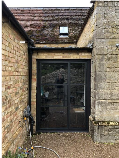
Existing flat roof above as viewed from rear courtyard. Note the new Roof Window will barely be visible when standing in the courtyard
