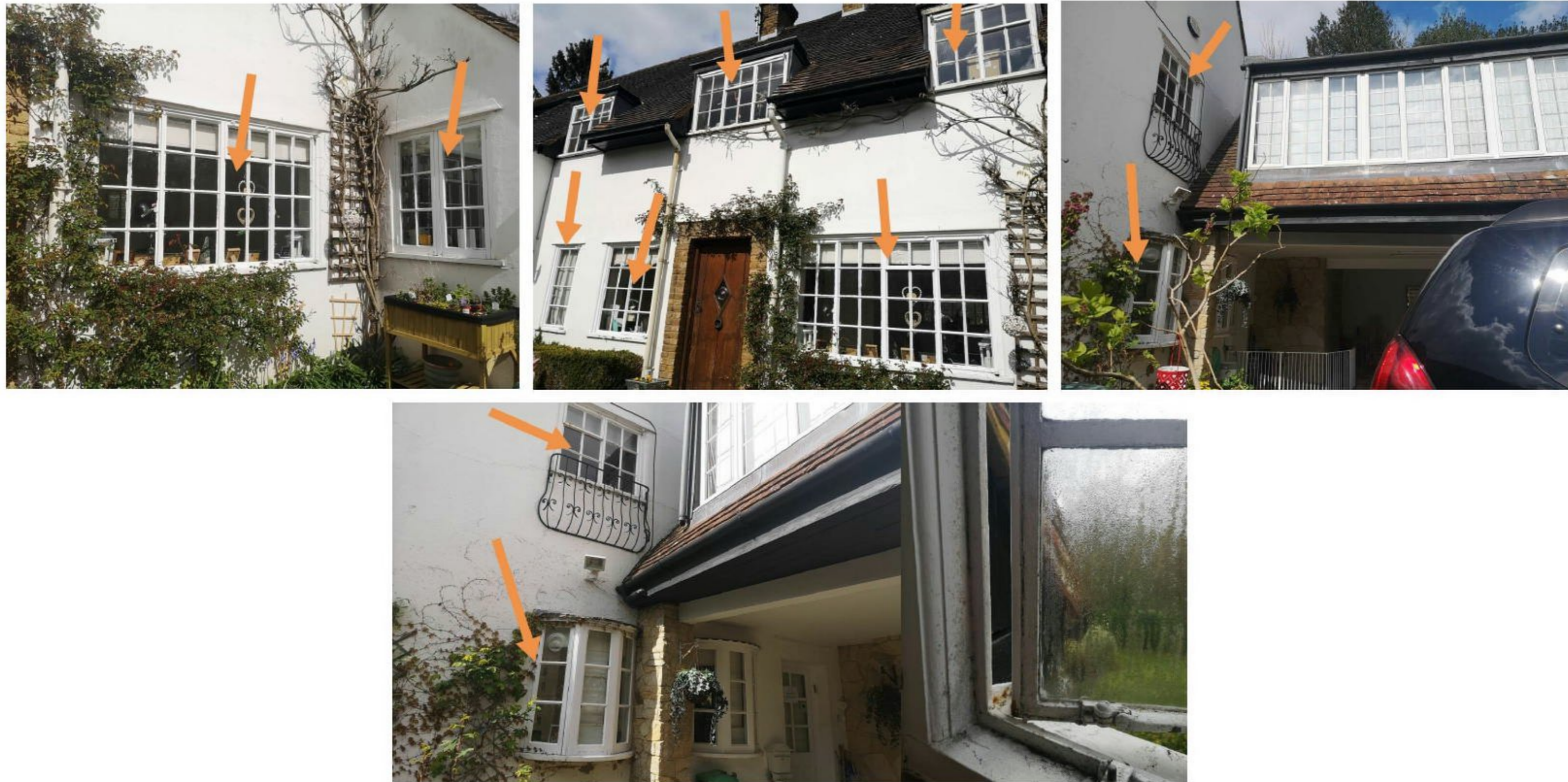
Figure 2 Photographs showing existing dilapidated windows to be replaced
