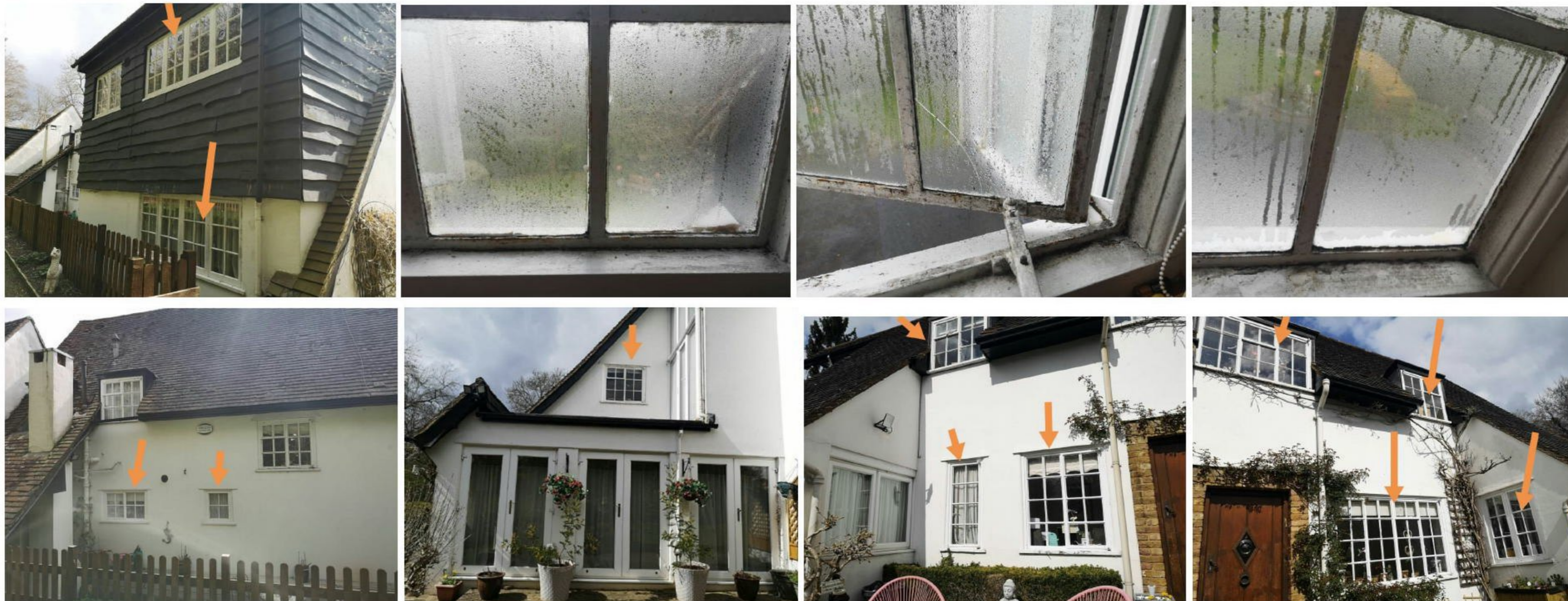
Figure 1 Photographs showing existing dilapidated windows to be replaced
