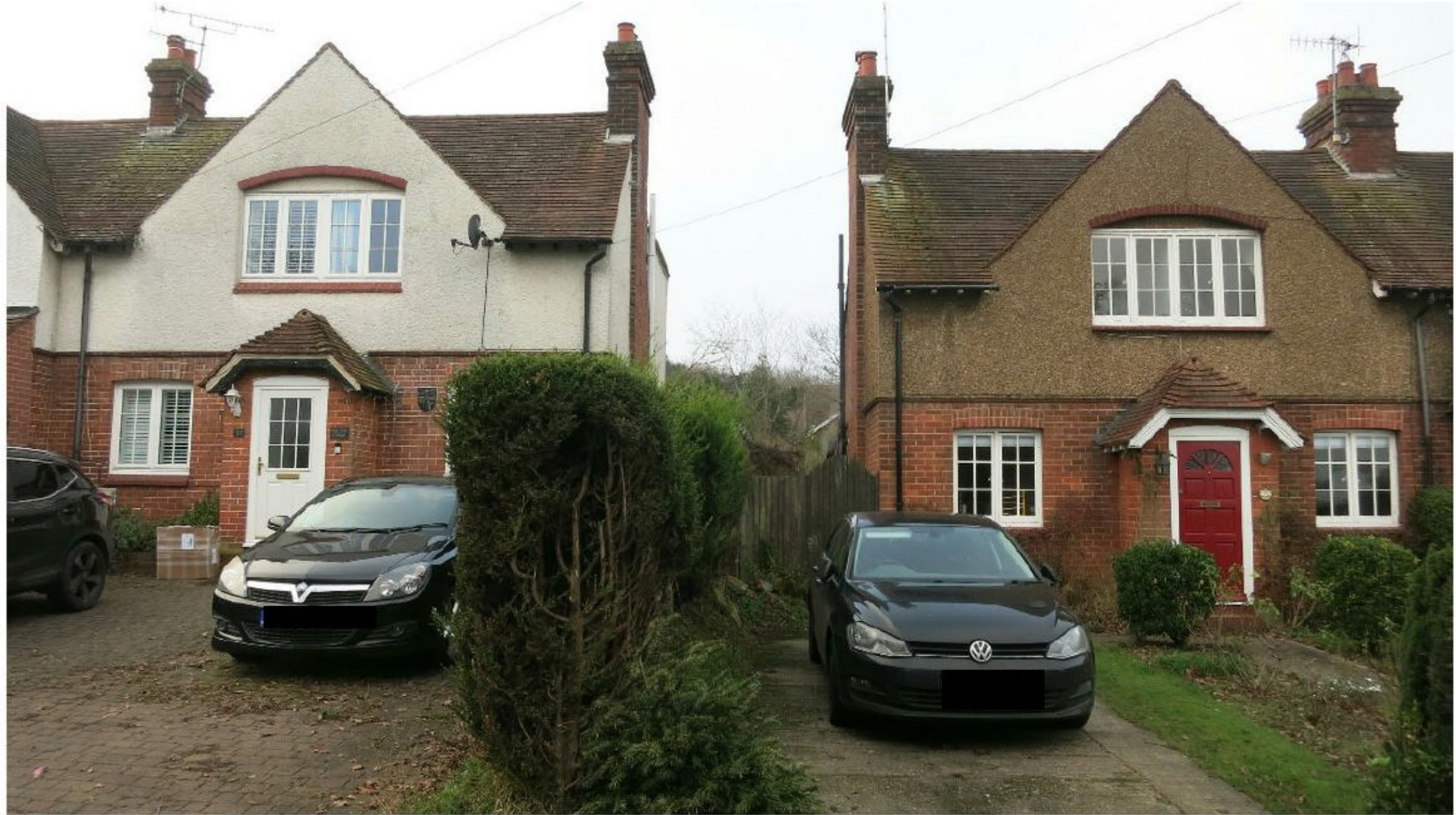
The existing gap between the 17 Powder Mills and the neighbouring property
