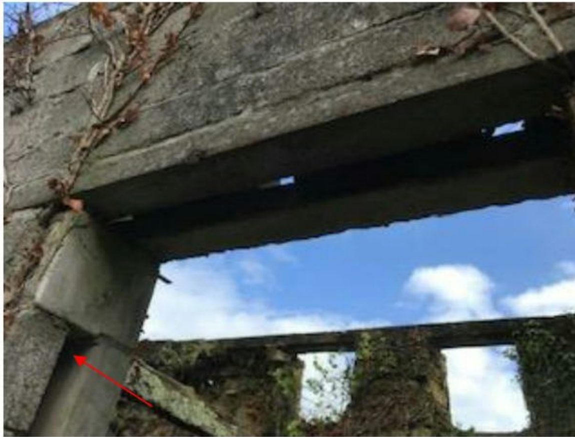
Photo 3: Cavity between the concrete blocks
