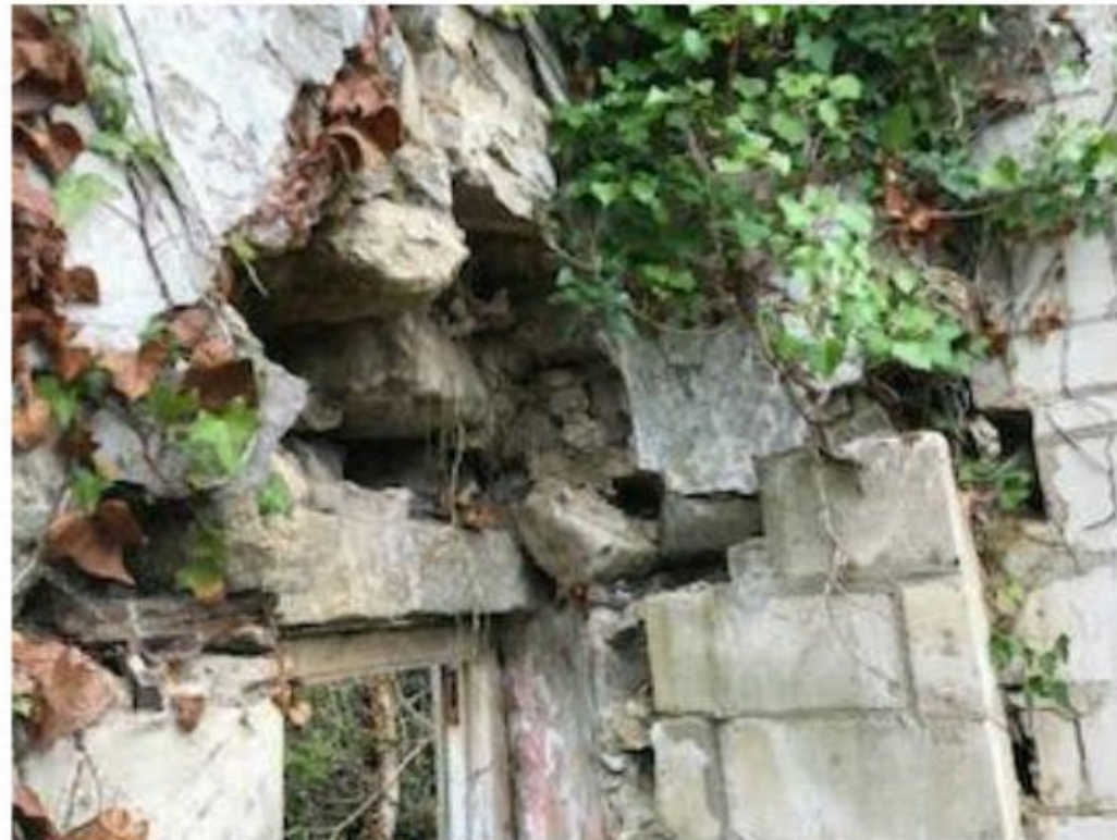
Photo 5: Crevices in the western elevation wall
