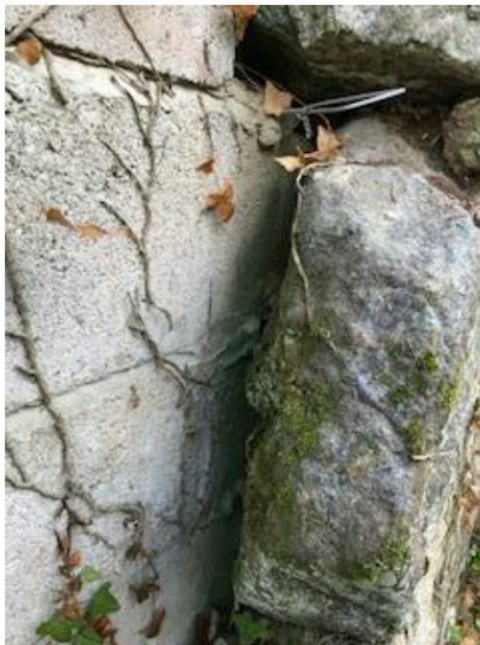
Photo 2: Crevices between the concrete block wall and stone wall
