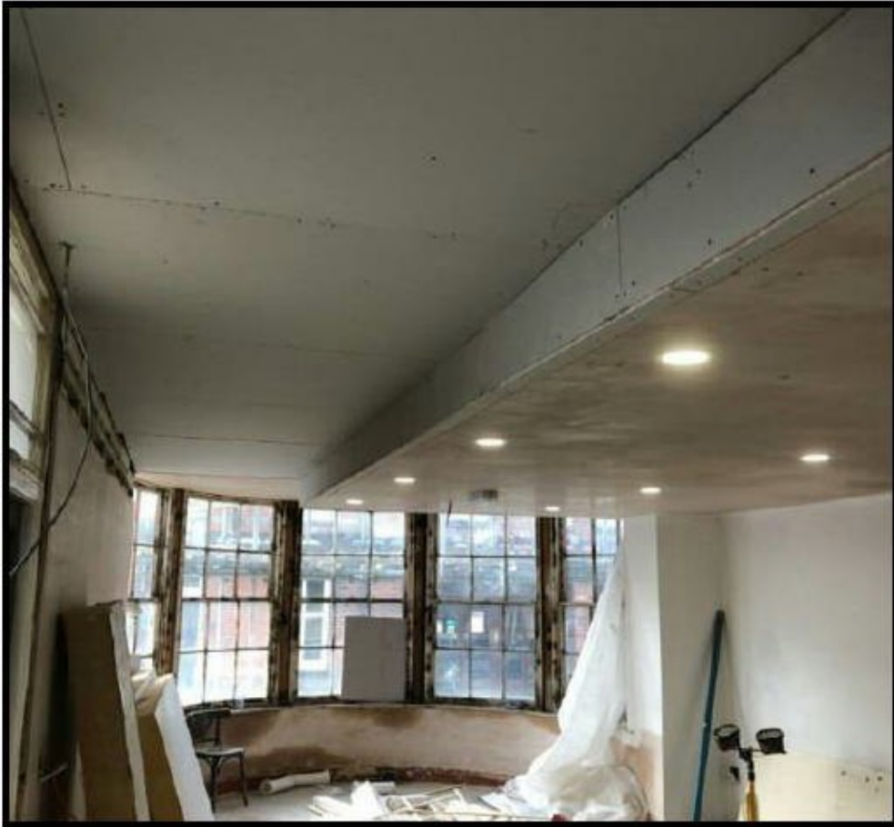
The raised ceiling height matches the full height of the bow window. See drawing number P&P/20/160/01
