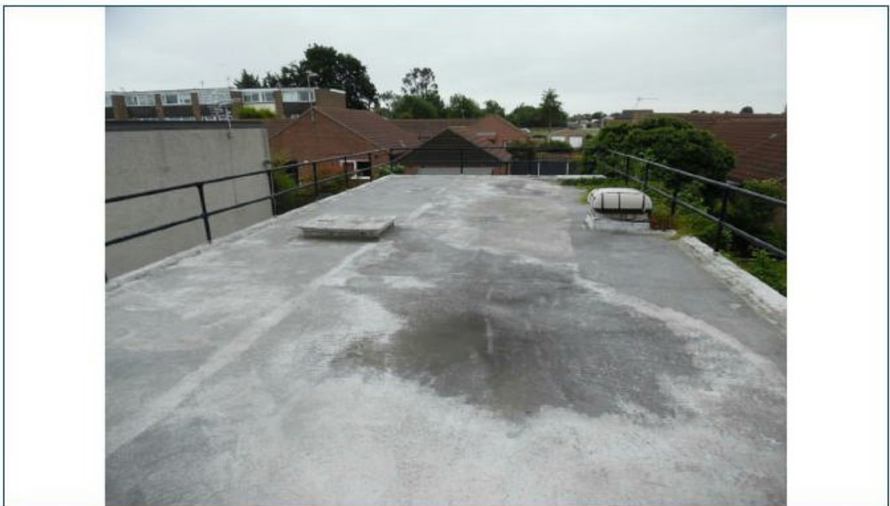
Photo 02 Flat roof and section for proposed pitched roof. Adjacent bungalows seen in background.
