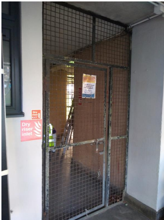
Access gate with side panel
