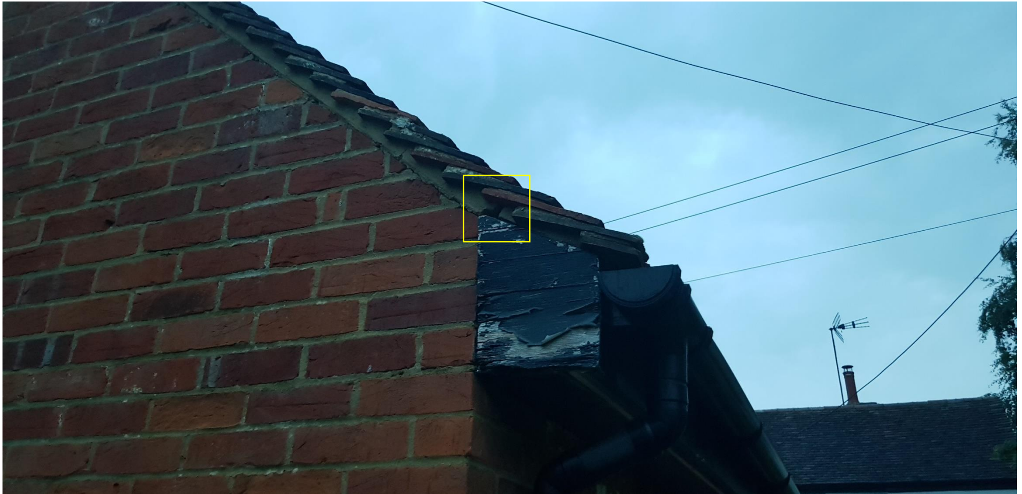
Photo 2: Close up of the roosting crevice under missing mortar.
