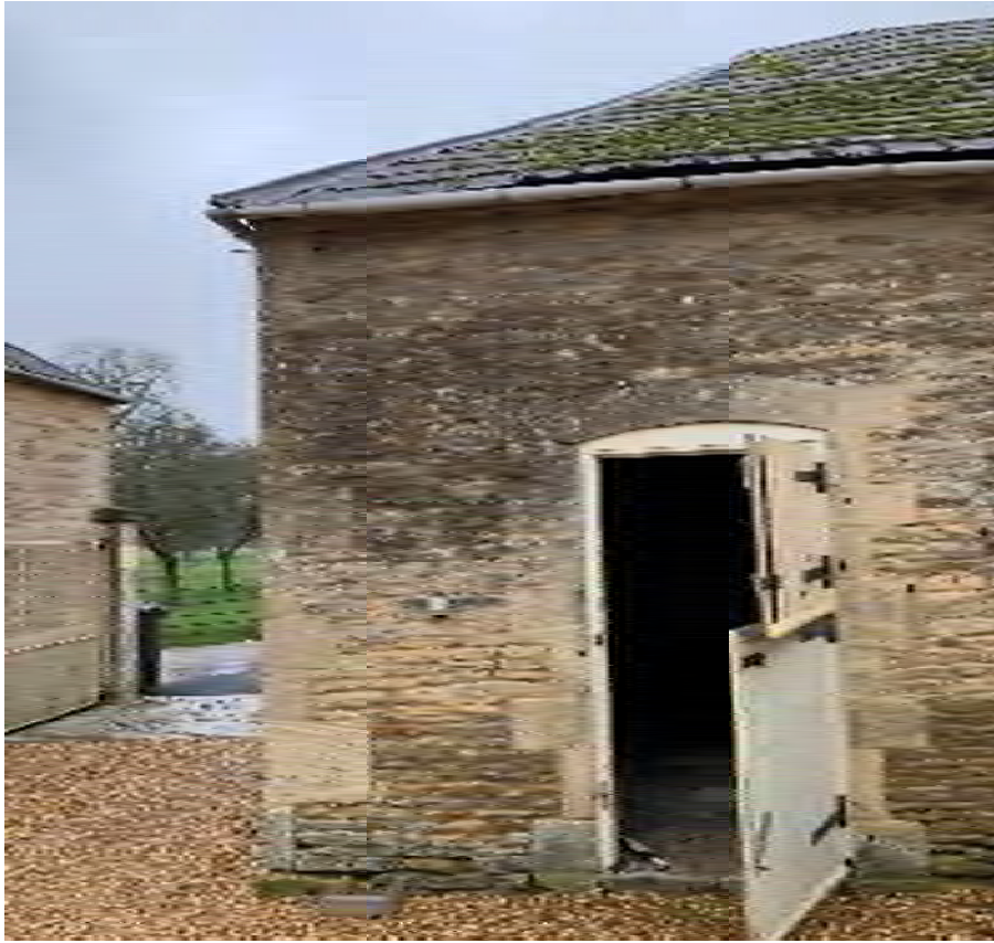
Heavily modified door to be replaced with semi-glazed door.
