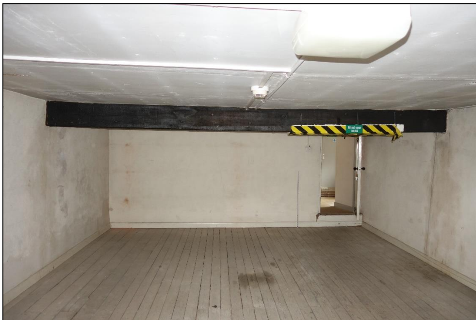
Plate 5: Internal view looking south showing exposed ceiling beam in first floor room within No. 131 (Border 2019)
