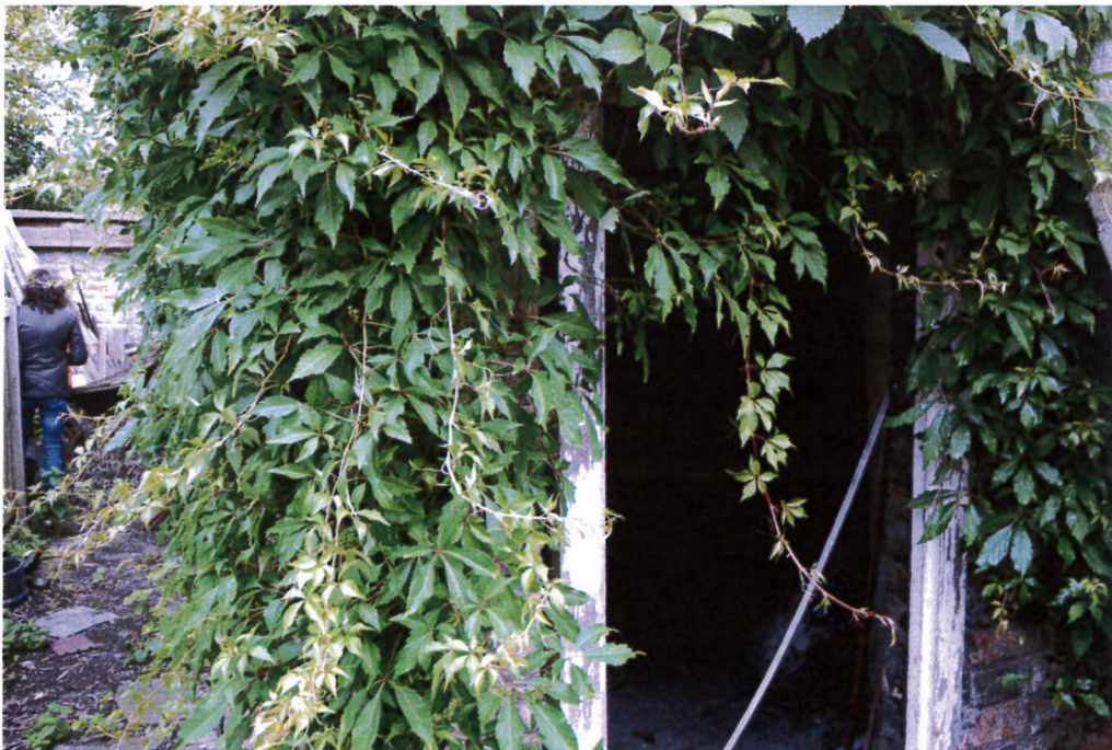
Movement to doorway in Right Hand Wall
