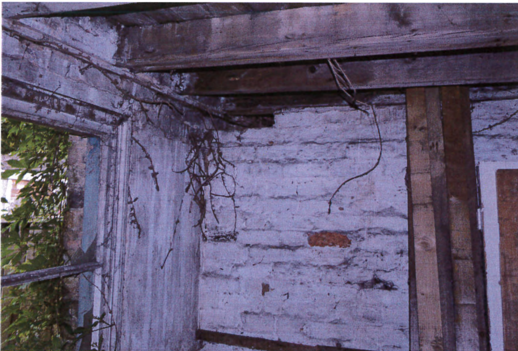
Minor timber damage in right hand room
