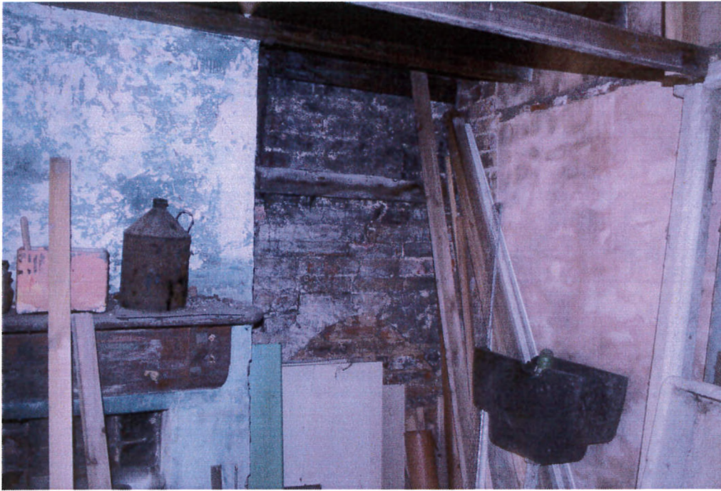
Cracking to left wall, left hand room
