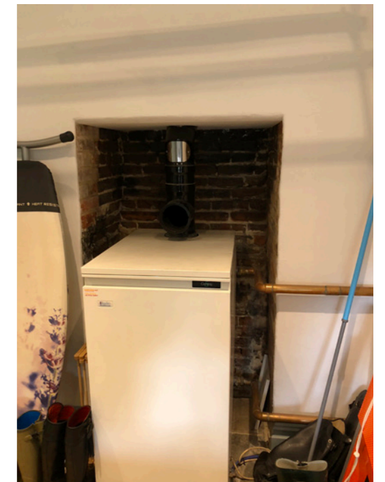
Existing boiler requiring replacement. Existing flue no longer to spec and replacing boiler in this location would increase risk of damage to the historic fabric of Hall Place
