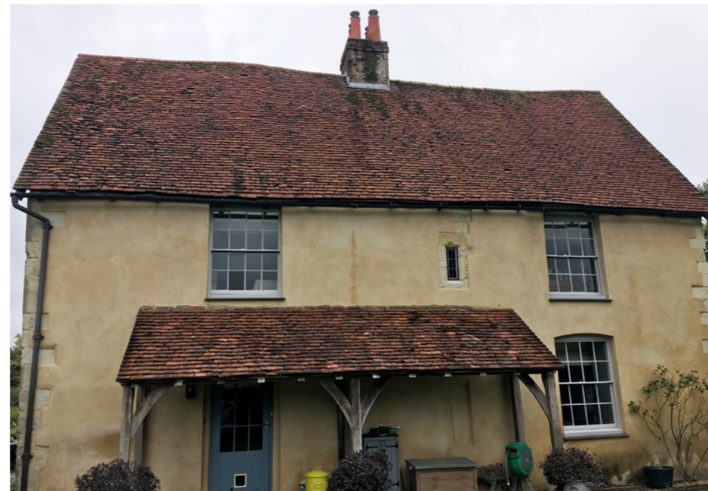
East elevation of Hall Place main house showing Boot Room entrance (Existing boiler currently located in Boot Room). Pipework to penetrate through wall where existing oil pipe is located
