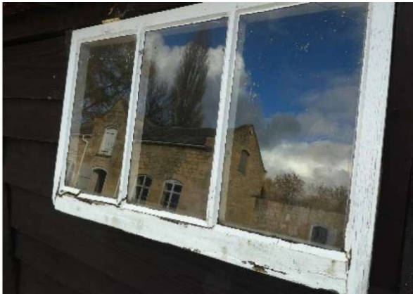
Modern window in a state of disrepair to be replaced.
