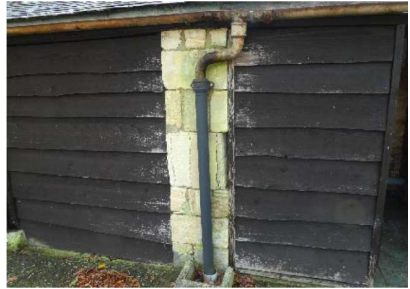
Modern materials – Painted softwood cladding to be removed.
