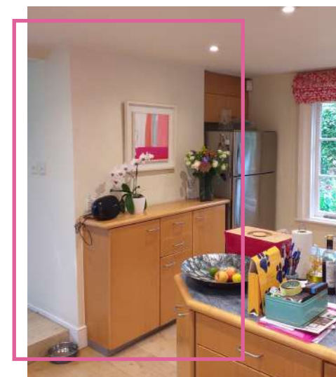
02 Existing chimney-breast not functional. Original planform disrupted by modern extension
