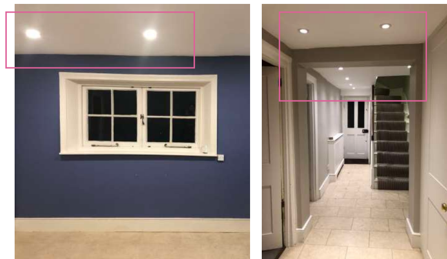
16 Photos of Lower Ground Floor; modern ceilings and inset downlights. Note: no cornicing present
