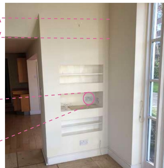
01 Existing wall not original; instead a stud partition rebuilt during extension. New beam installed over to support existing structure above.
