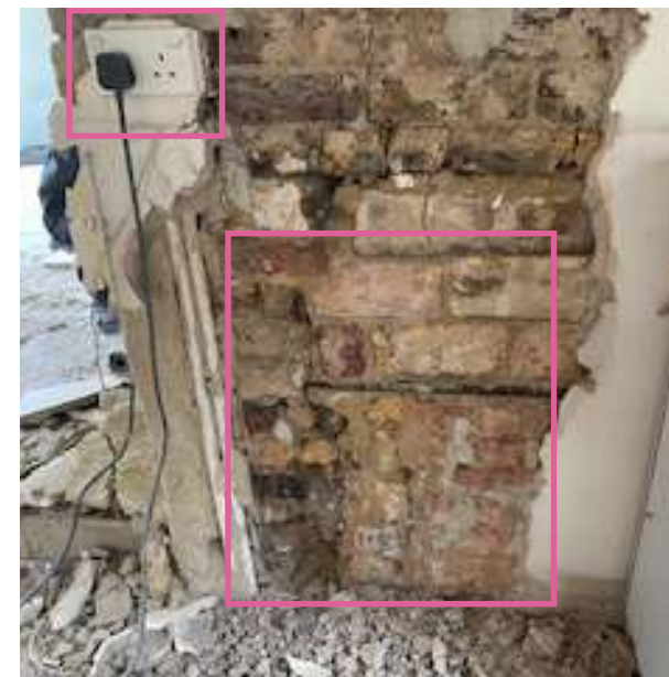
09 More areas of modern brickwork to chimney-breast. Modern services installed onto original fabric.
