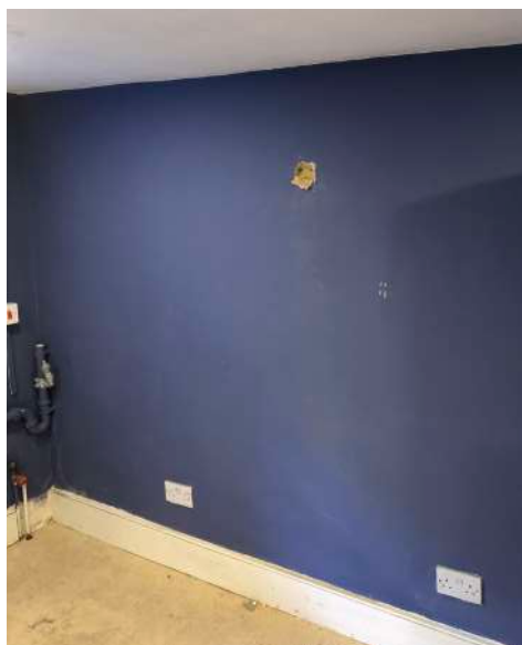
13 Photos of existing WC located at Lower Ground Floor, under the front entrance steps.
