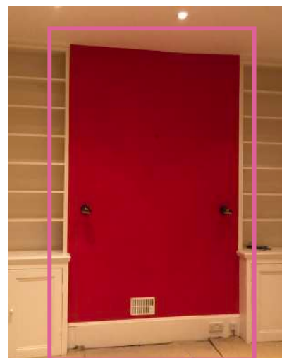
01 Photo taken internally showing existing chimney-breast blocked-up / plastered over.
