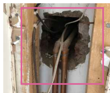
08 Crude service penetrations cut through existing building fabric
