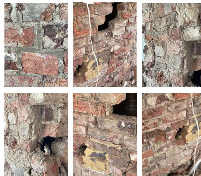
11 Close-up photos of modern brickwork following strip-out. Clear modern interventions and infill; little remaining historic fabric
