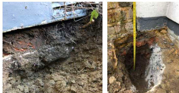
15 Photos of trial pits dug externally to expose foundation footing and non-original floor structure (concrete slab)
