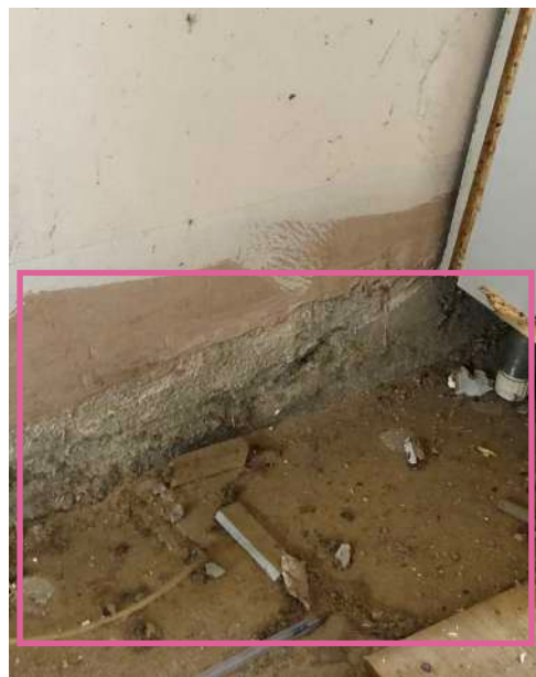
07 Strip-out at floor-level reveals no original hearth and modern concrete & plastered wall finish
