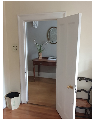
GF Living-Room door to be fixed shut
