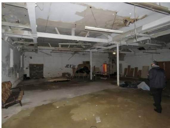
Figure 37 – The c1880s “ring room” showing the open pitched roof structure now boarded over.
