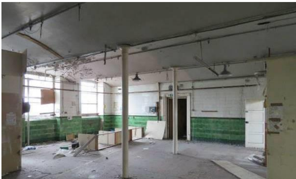
Figure 21 –Looking south-east across the former canteen in 2016, showing the Edwardian glazed tilework. (Heritage Architecture)
