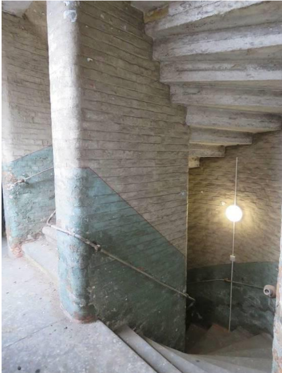
Figure 48 – An example of an upper floor of the east block, showing the full form and articulation of the original staircase.
