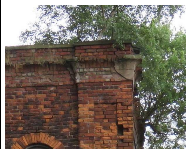
Figure 9 – 2016 – A view of the last remaining part of the original cornice, seen here around the perimeter of the former engine house. When first built, this cornice extended around the whole of the building, using curved bricks which were then coated with stucco to form the appearance of stonework.
