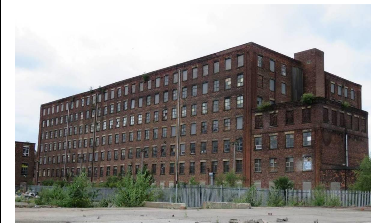
Figure 29 – The long rear elevation fronting onto the Ashton Canal. To the right is the 1844 waste house, the top storey of which was added in the 1920s.
