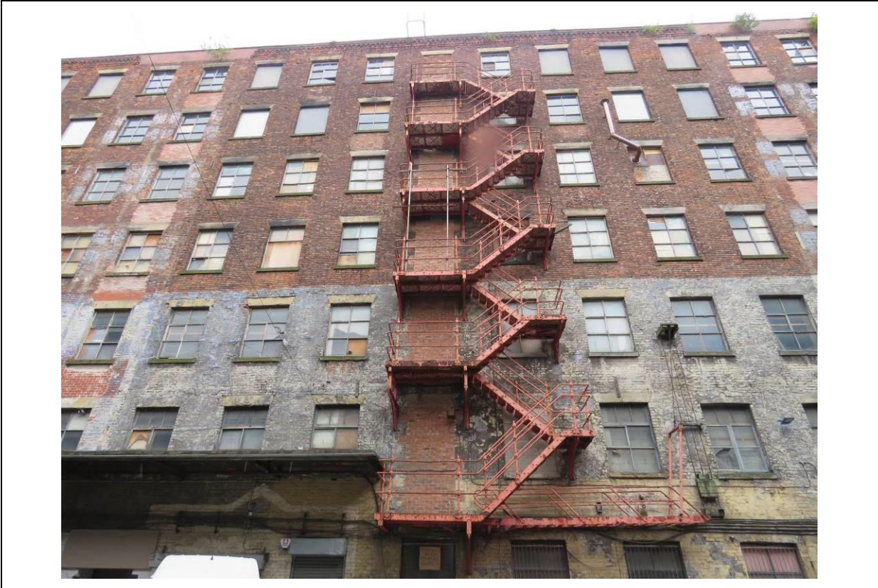
Figure 52a – The south courtyard elevation, showing the late-19 th /early-20 th century cast iron fire escape stairs.
