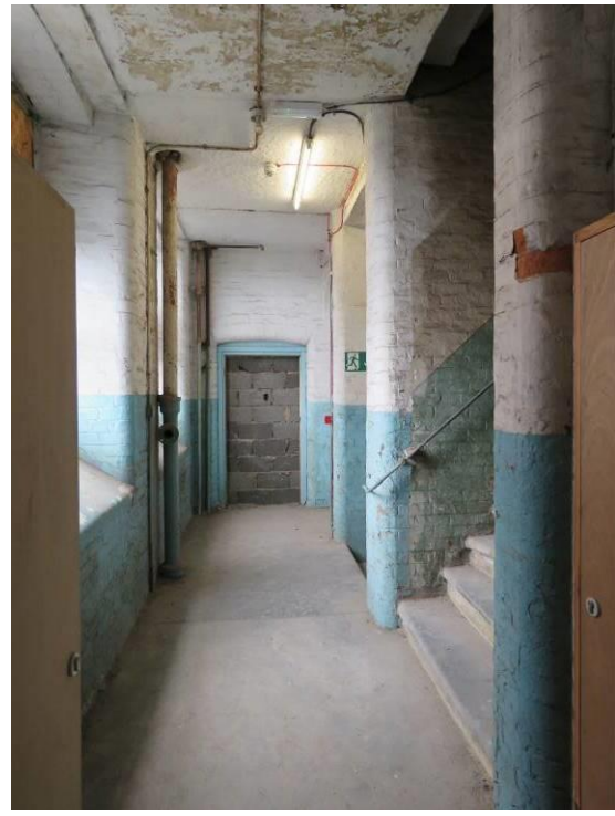
Figure 47 – An example of one of the upper floors of the east block, showing the link corridor between the main mill and the eastern wing.
