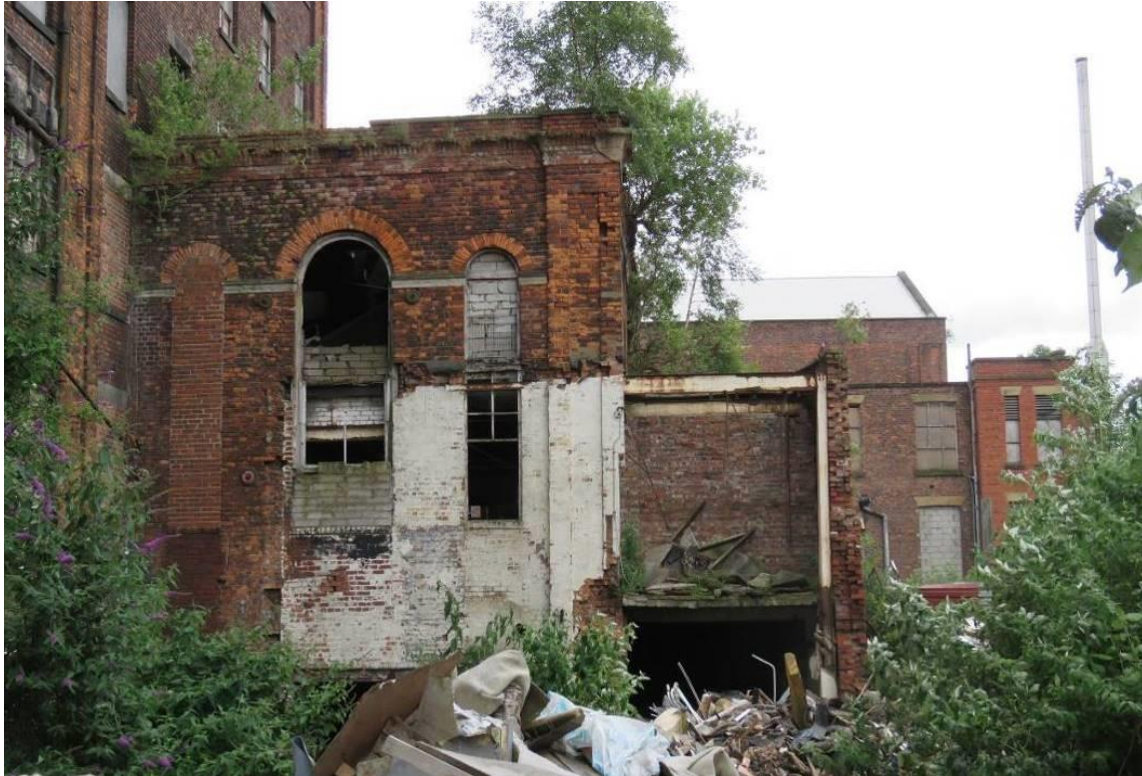
Figure 33 – A view of the former engine house, used to power the mill between 1839 and 1908. The building was inaccessible at the time of survey.
