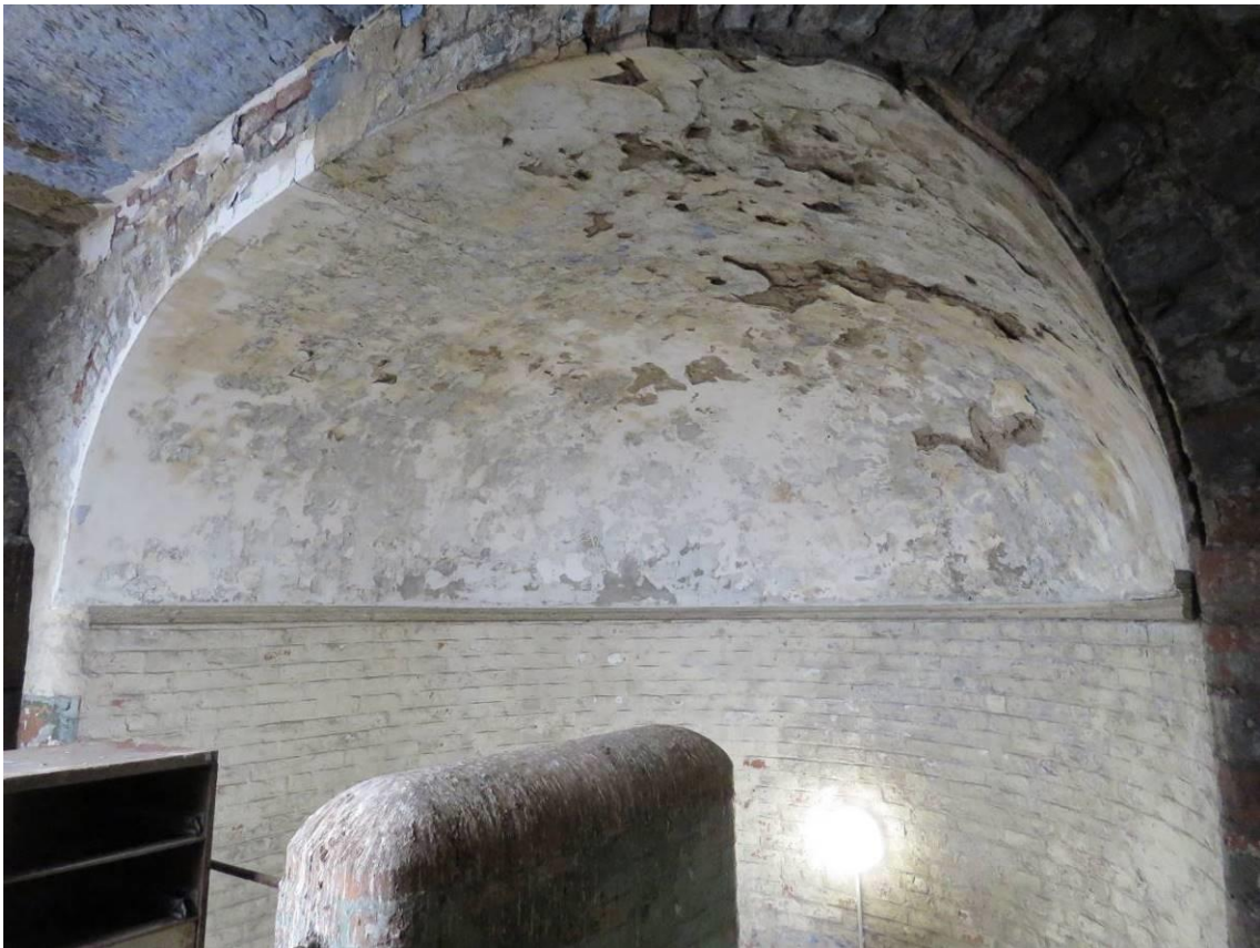
Figure 50 – A closer view of the termination of the staircase with its half-domed ceiling.
