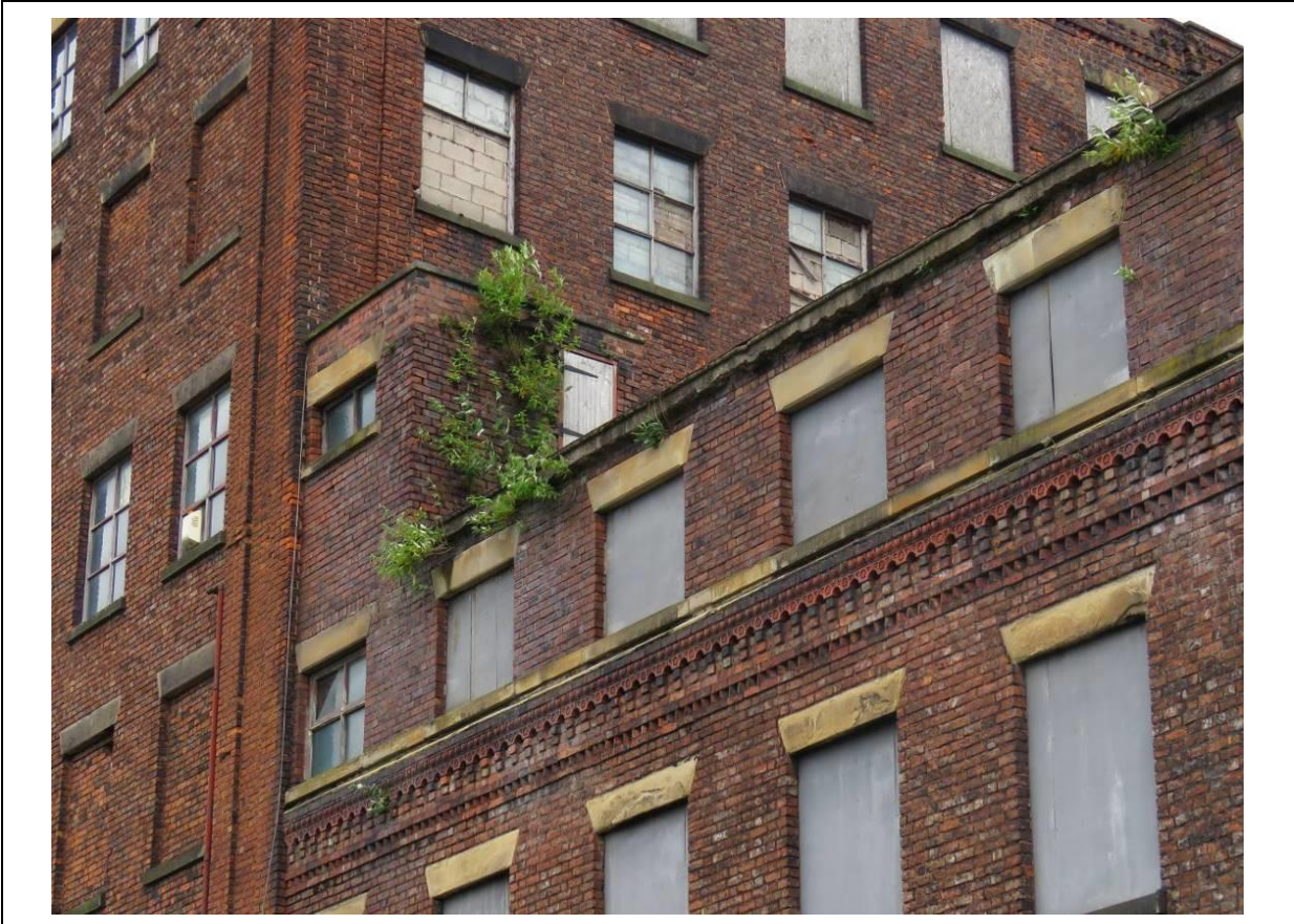
Figure 28 – Looking up to the inside, courtyard face of the eastern wing, showing the 1920s extension forming the third floor level above the north block. The blocked windows to the far left of the east block denote the former glazed tile dining room.
