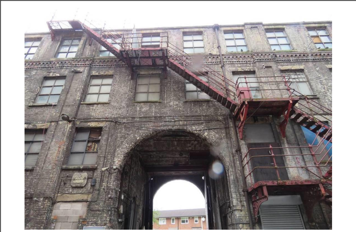
Figure 52b – The north courtyard elevation, showing the late-19 th /early-20 th century cast iron fire escape stairs and originally central covered entrance.
