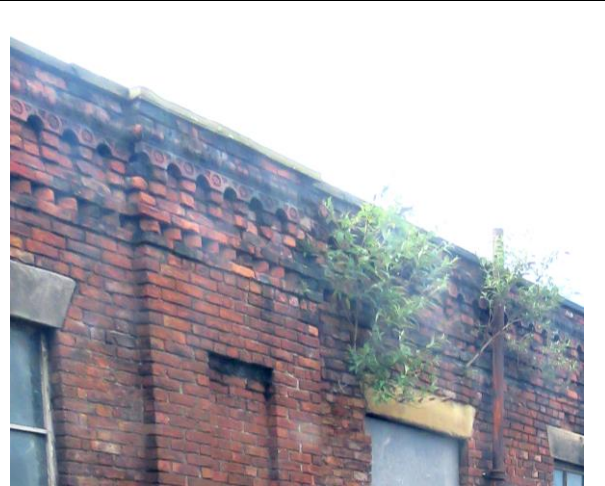
Figure 10 –2016 – A example of the current cornice that now surrounds the entire building (except former engine house). The original stuccoed cornice was removed during the c1890s and replaced with decorative red brick. This redesign was probably undertaken due to the deterioration of the stuccowork.
