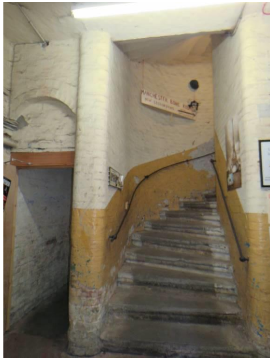
Figure 46 – The staircase hall of the original stairs in the east block. Note the original iron handrails and stone treads. The narrow door to the left leads into the rear staircase hall, which originally houses the toilets and a link into the northern end of the east block.
