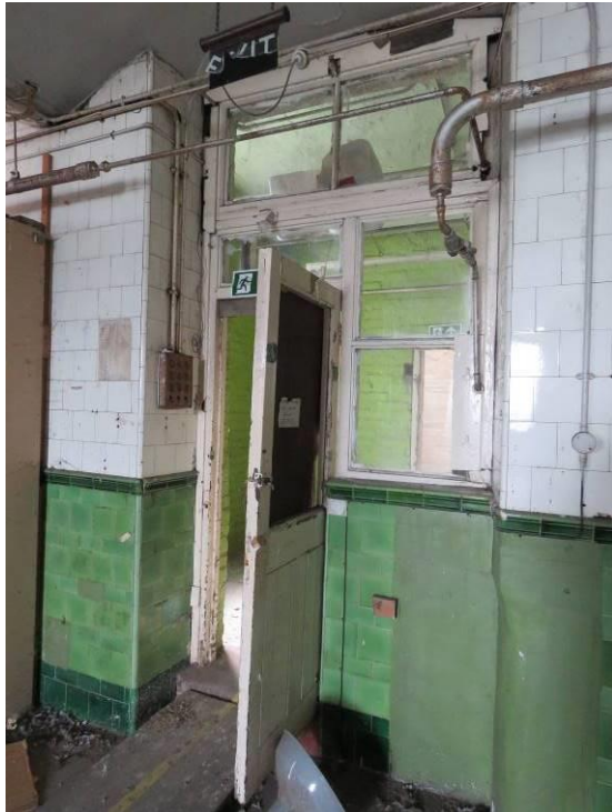
Figure 42 – The doorway between the canteen and the kitchen, on the third floor of the east block, showing the green and white Edwardian glazed tiling.
