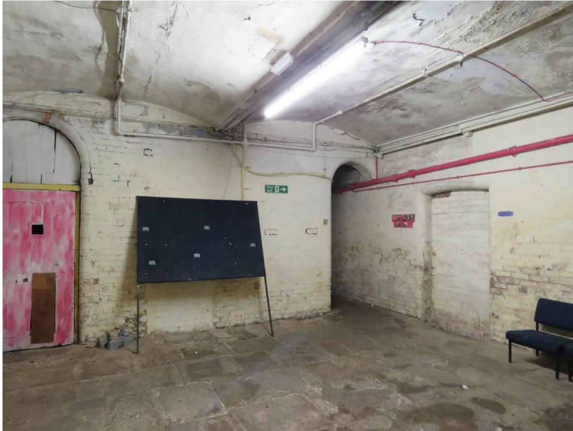
Figure 36 – The wide corridor to the rear of the staircase in the east wing, showing the narrow passage into the staircase hall to the right, and a now blocked hoist/chute to the left. Note the original stone flags to the floor.
