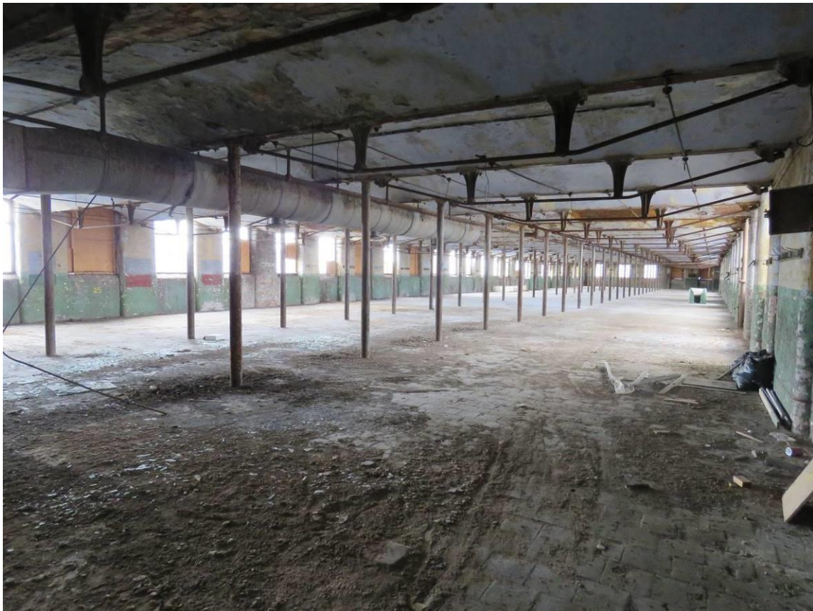
Figure 43 – A view looking west across the sixth (top) floor level of the main mill building
