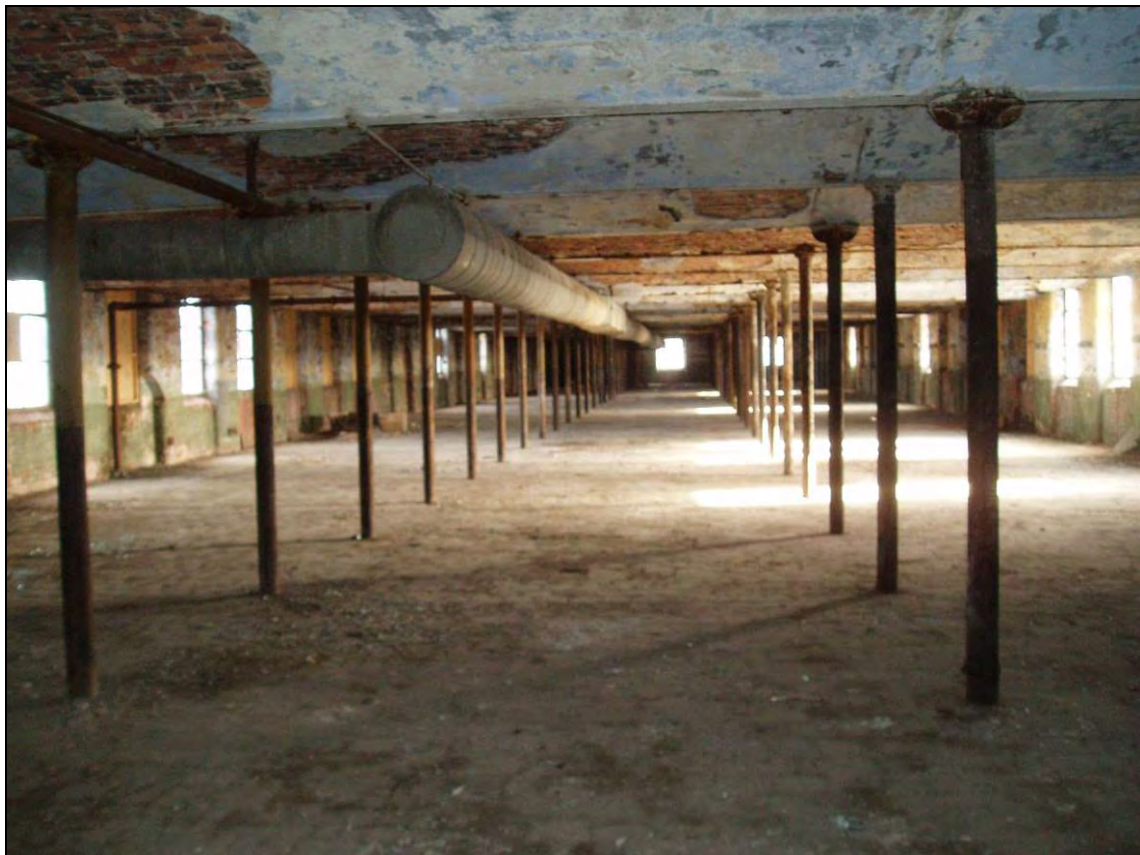
Plate 4: The top floor of the main spinning block, showing the fireproof construction
