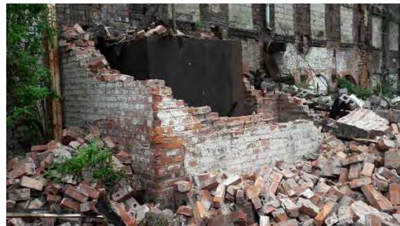
Photograph 4 (P4) Relic oil tank located in the south west of the mill building.
