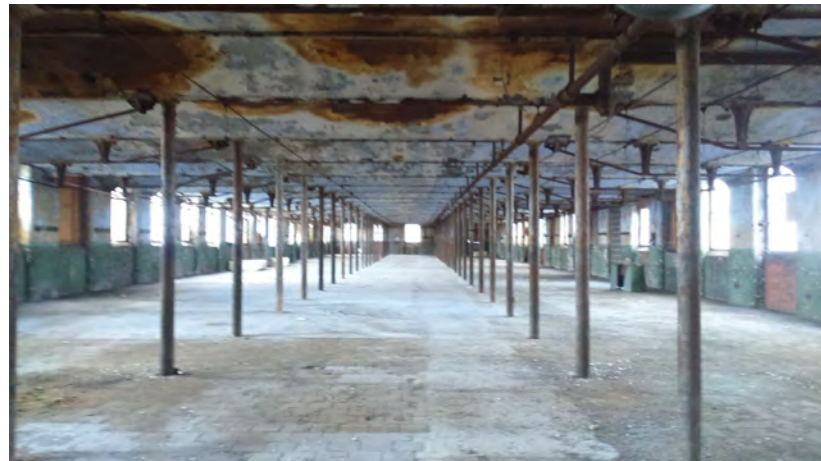
Existing mill structure indicating trussed ties introduced in 1920's to reinforce the floors
