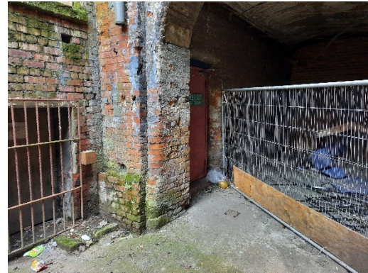
Photograph 2: Loose and missing bricks within the Brunswick Mill courtyard.
