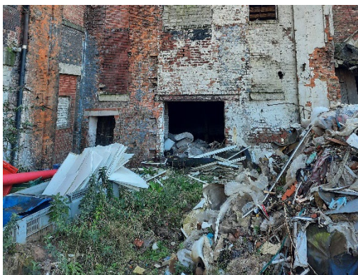
Photograph 5: Debris piles and broken/boarded windows within the southwest section of the Site.
