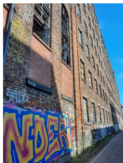
Photograph 20: Boarded windows and graffiti along the external walls of the mill buildings.
