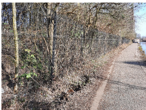
Photograph 19: External fencing and dense vegetation along the boundary of the site and canal towpath.
