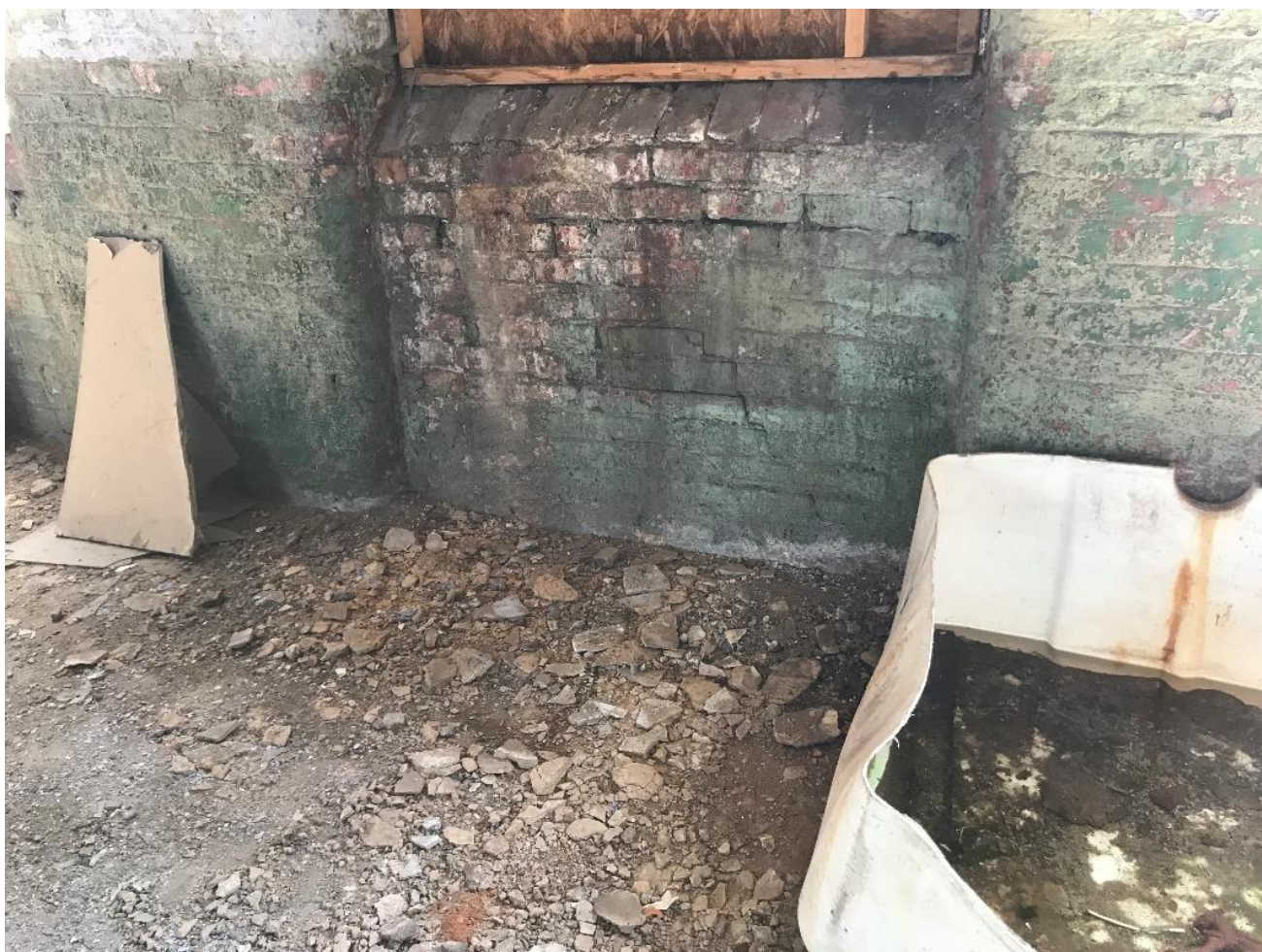
Figure 21: Drop in Cill Level and Associated Cracking to Masonry
