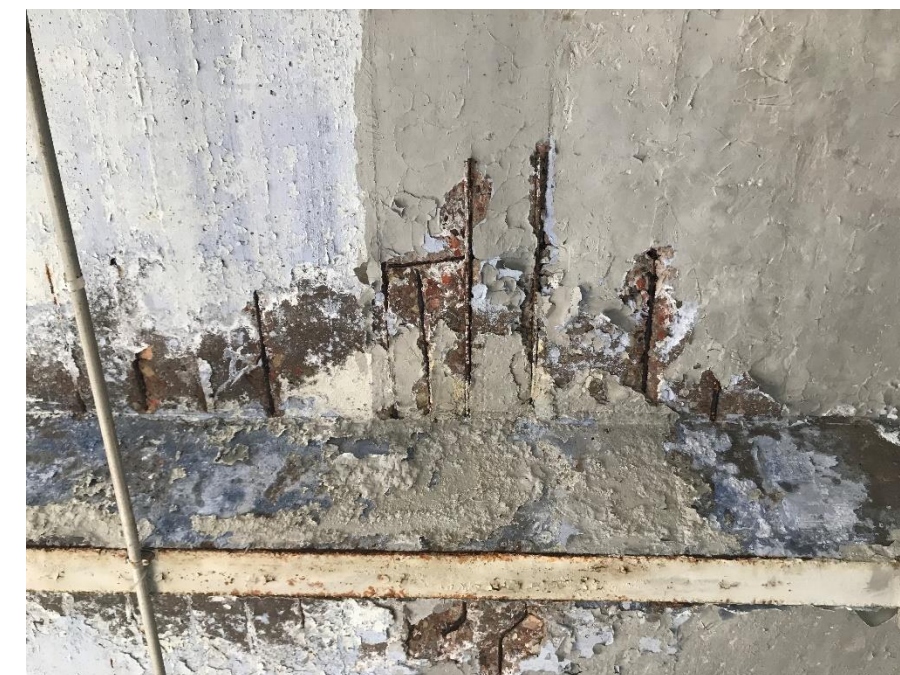
Figure 33: Stained Slab Soffits and Corroded Reinforcement
