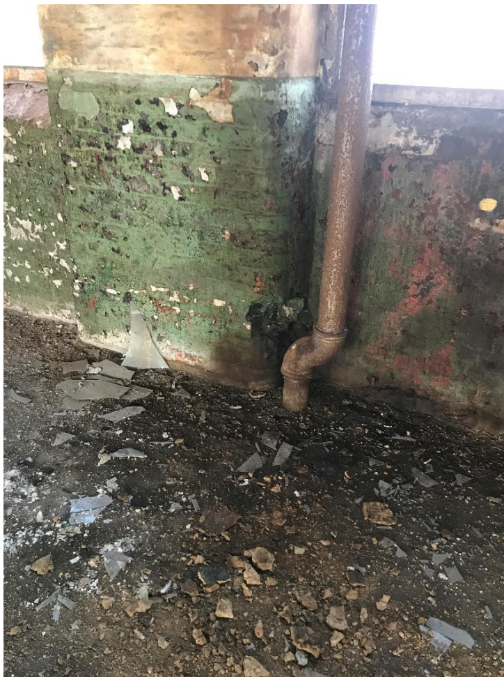
Figure 23: Small Areas of Masonry Loss in Pier
