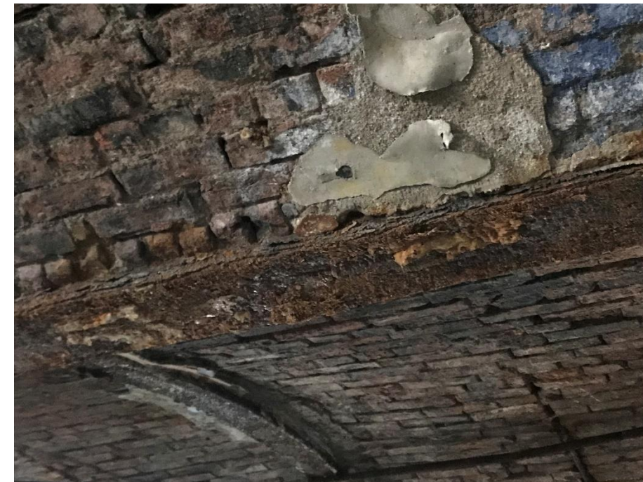
Figure 19: Lamination of Cast Iron Structure Resulting from Water Ingress
