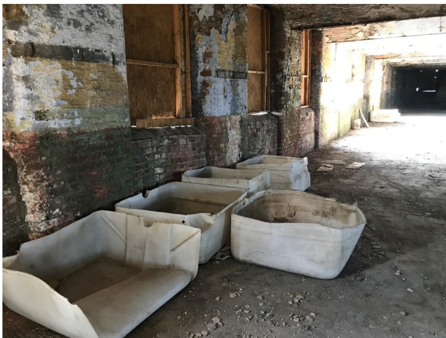
Figure 18: Plastic Buckets to Catch Water from Leaking Roof.
