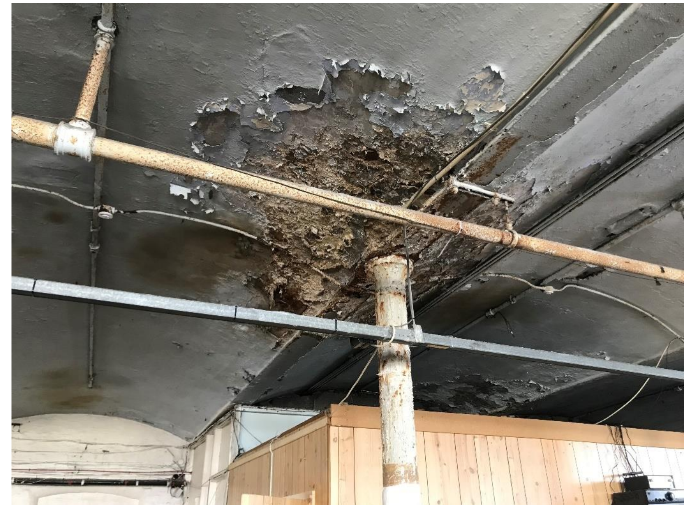
Figure 27: Damage to Masonry Jack Arch and Cast Iron Structure
