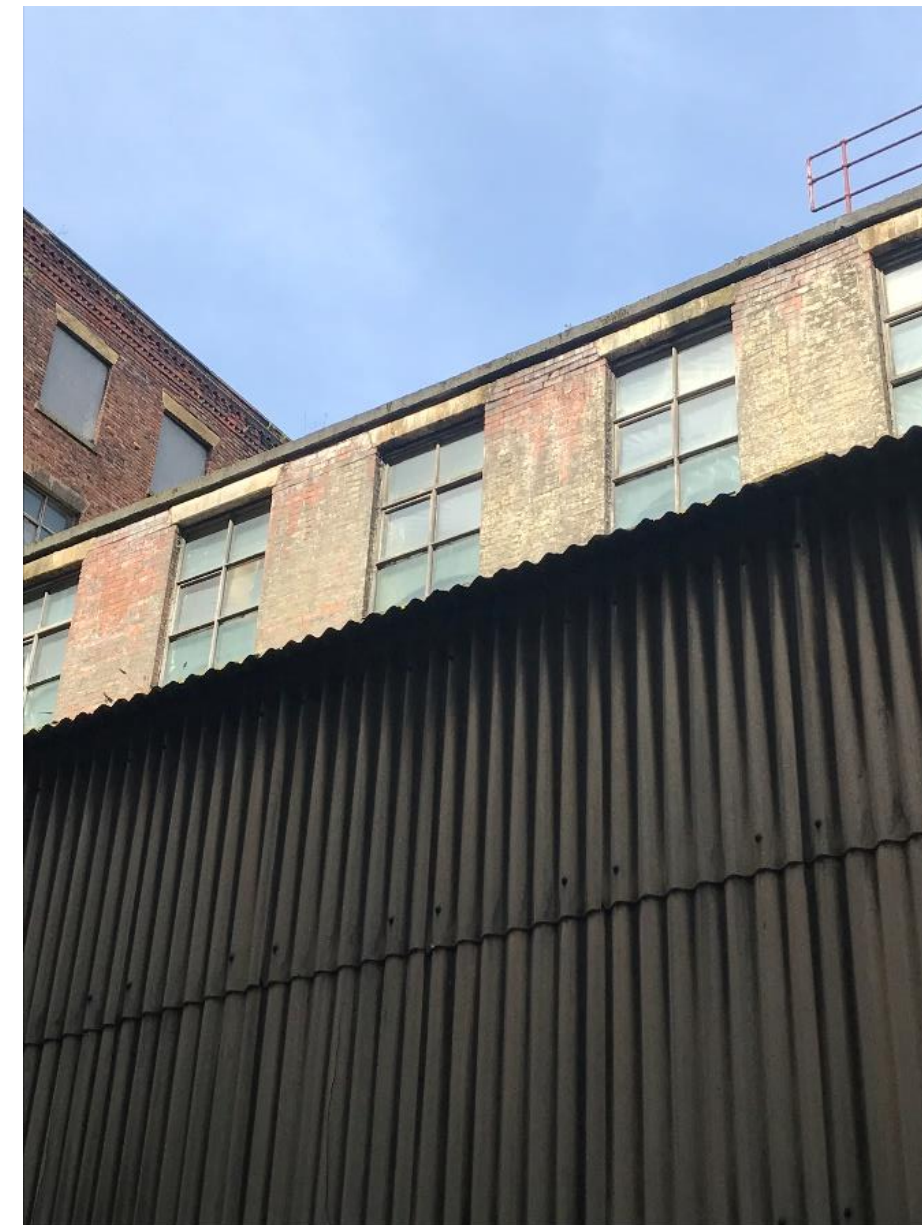
Figure 77: Open Joints and Loos Brickwork
