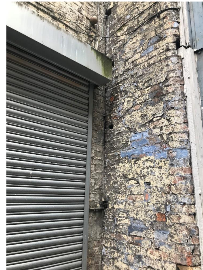
Figure 83: Differential Movement Causing Peeling Away of Two Storey Structure
