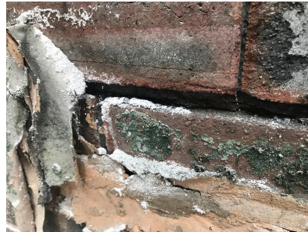
Figure 35: Corroded and Expanded Bed Joint Reinforcement
