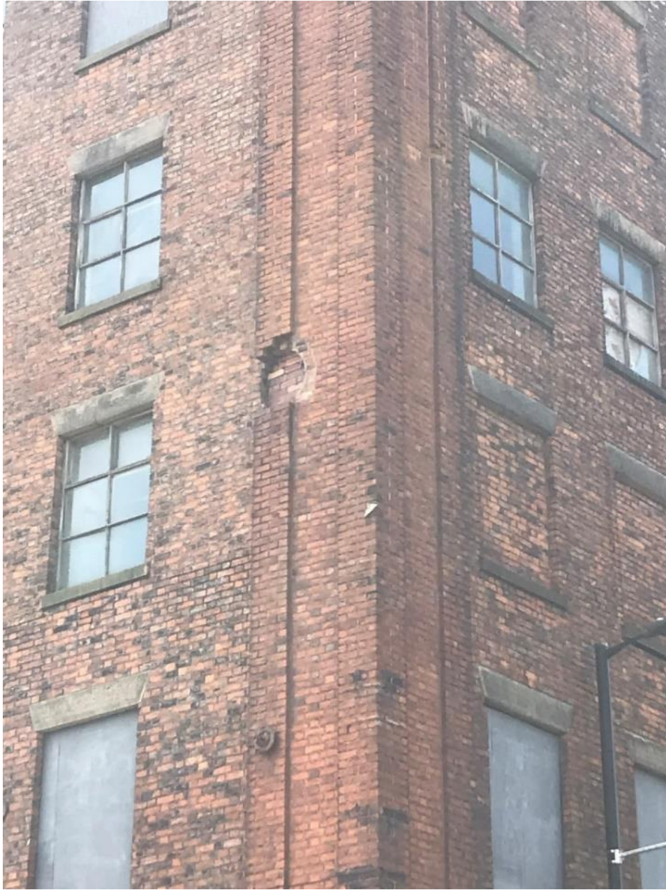
Figure 67: Localised Loss of Masonry to Pier
