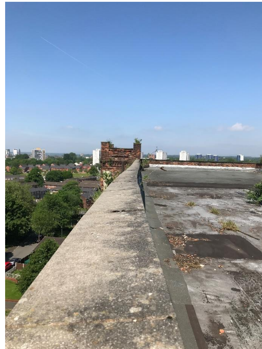
Figure 15: Significant Bowing of Southern Parapet
