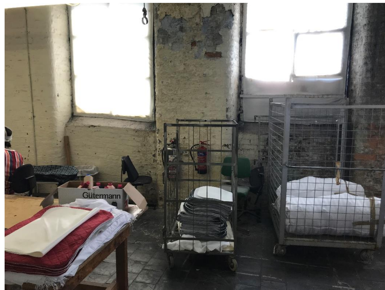
Figure 30: Obvious Drop in Cill and Floor Level
