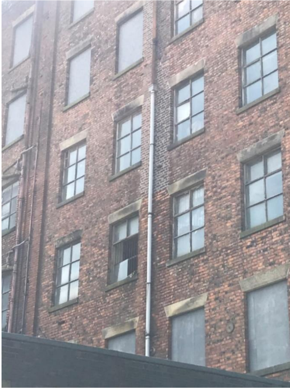
Figure 66: Localised Loss of Masonry to Pier
