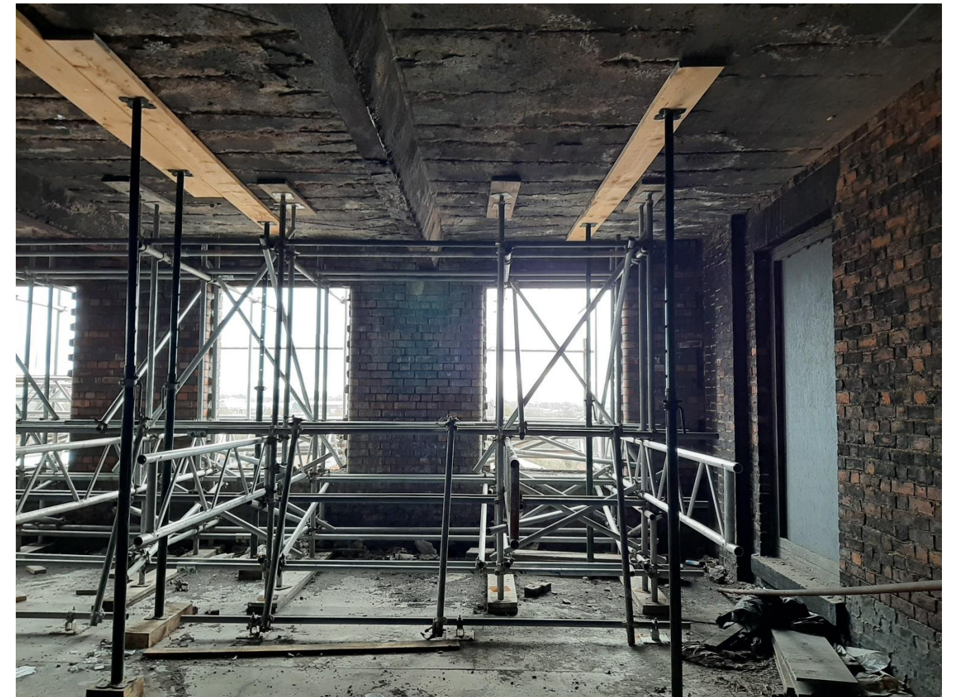
Figure 43: Propping Installed by Client to Third Floor Former Waste House and Repair work started.
