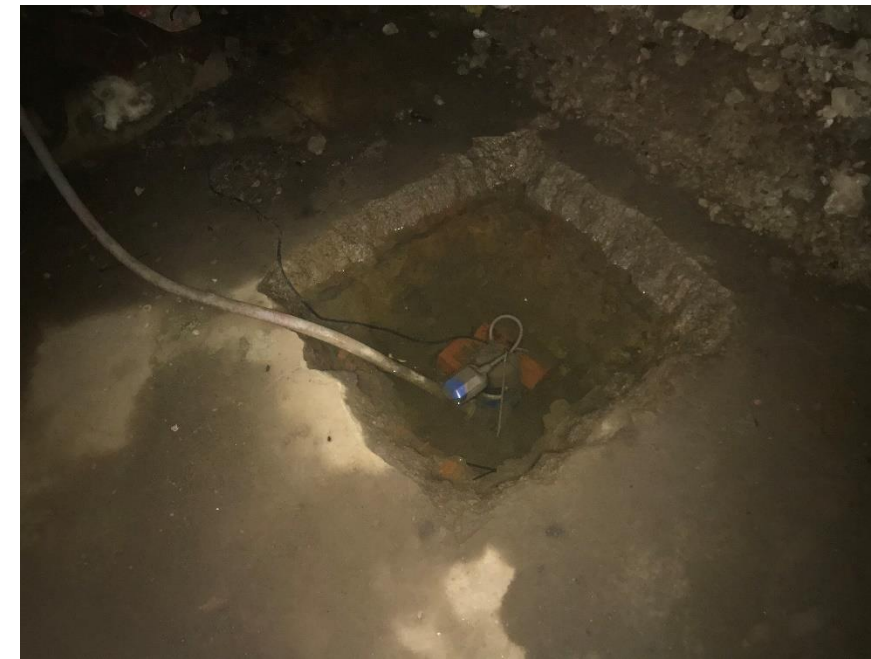
Figure 59: Sump Pump Installed
