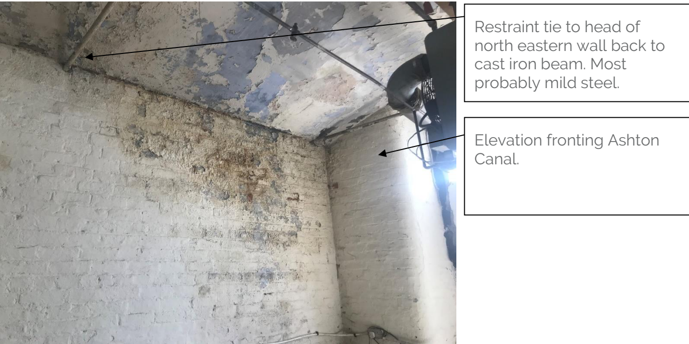
Figure 46: Restraint Bars to North Eastern Wall of Former Waste Room Second Floor
