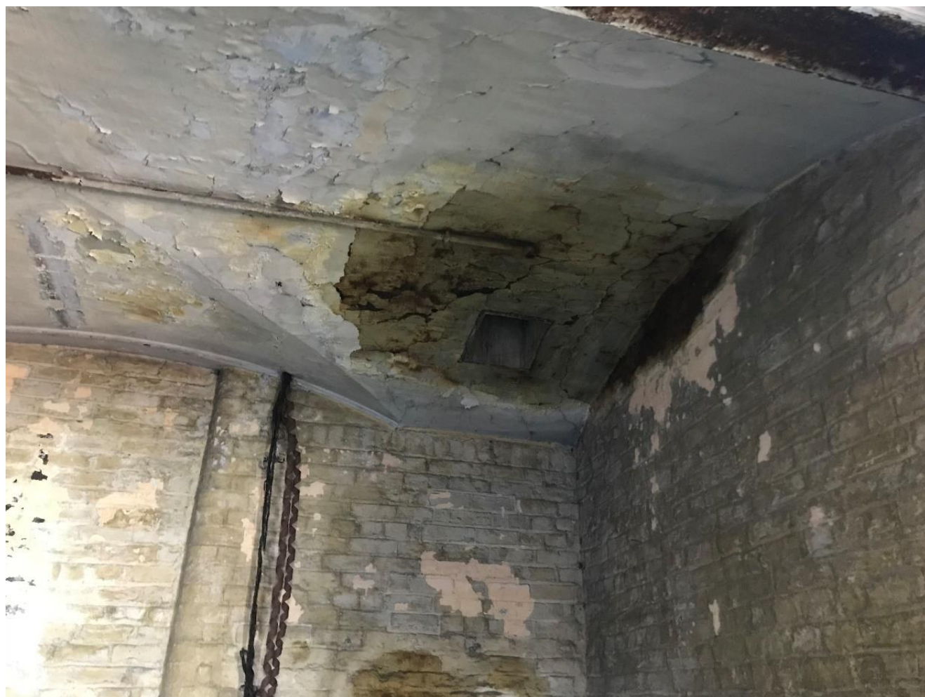
Figure 25: Water Staining and Damage to Jack Arches at Squinch Corner
