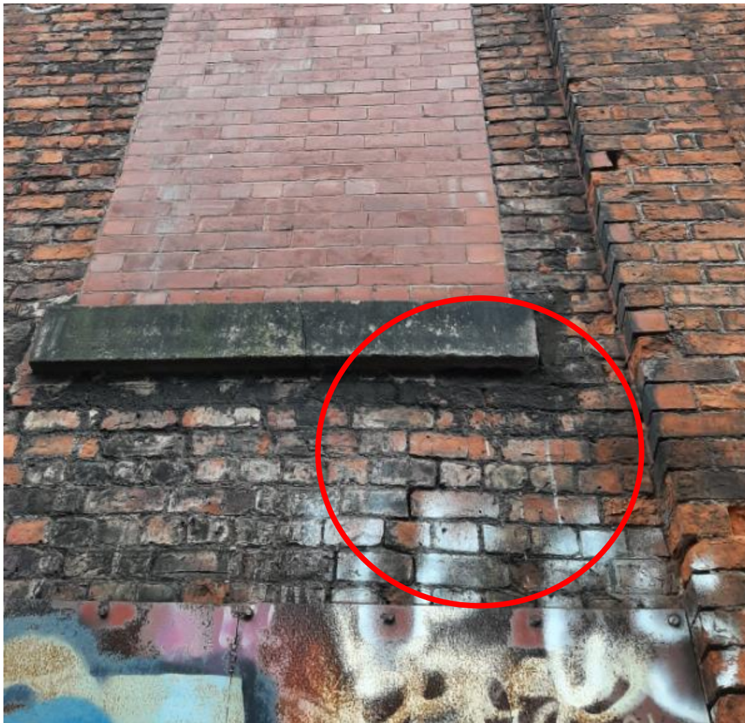
Figure 95: Cracked Masonry on External Elevation
