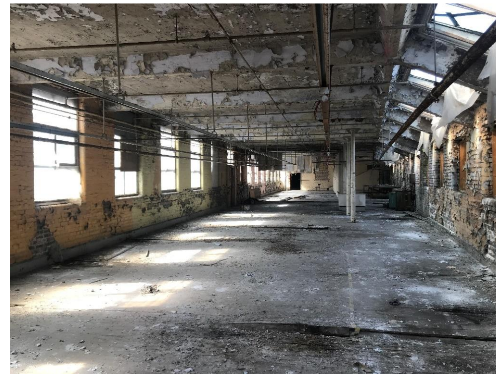
Figure 36: General Efflorescence Staining to Masonry
