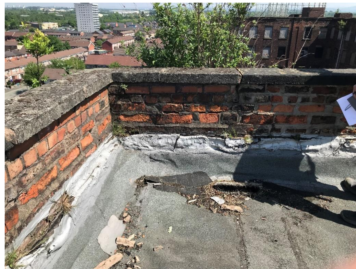
Figure 17: Cracking and Loss of Pointing Generally
