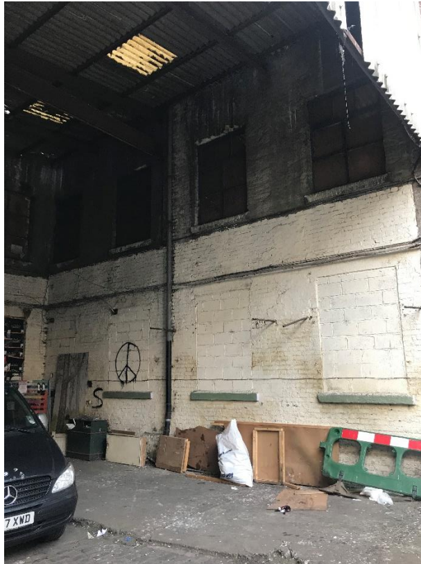
Figure 87: Brickwork Staining at Lower Levels Behind RWP
