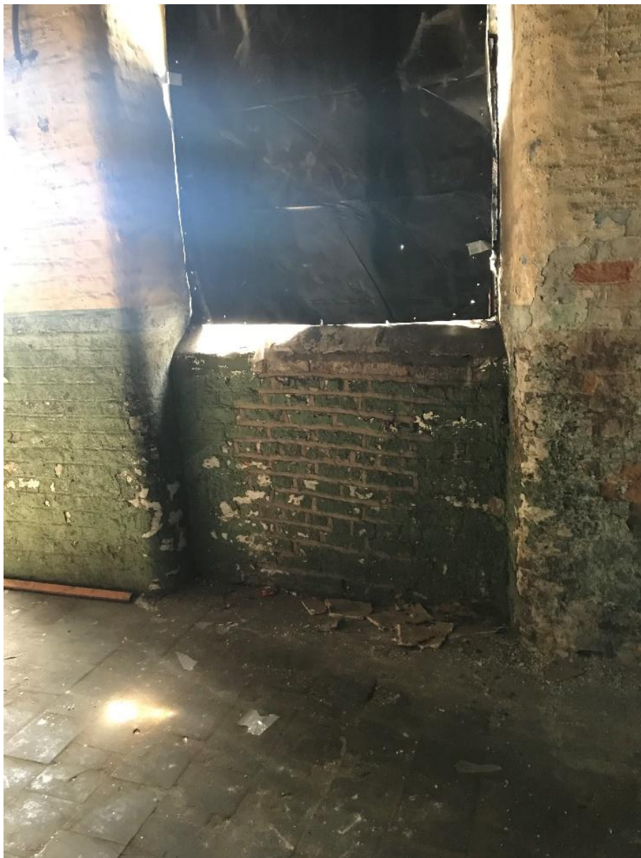
Figure 39: Settled Wall Fronting Ashton Canal
