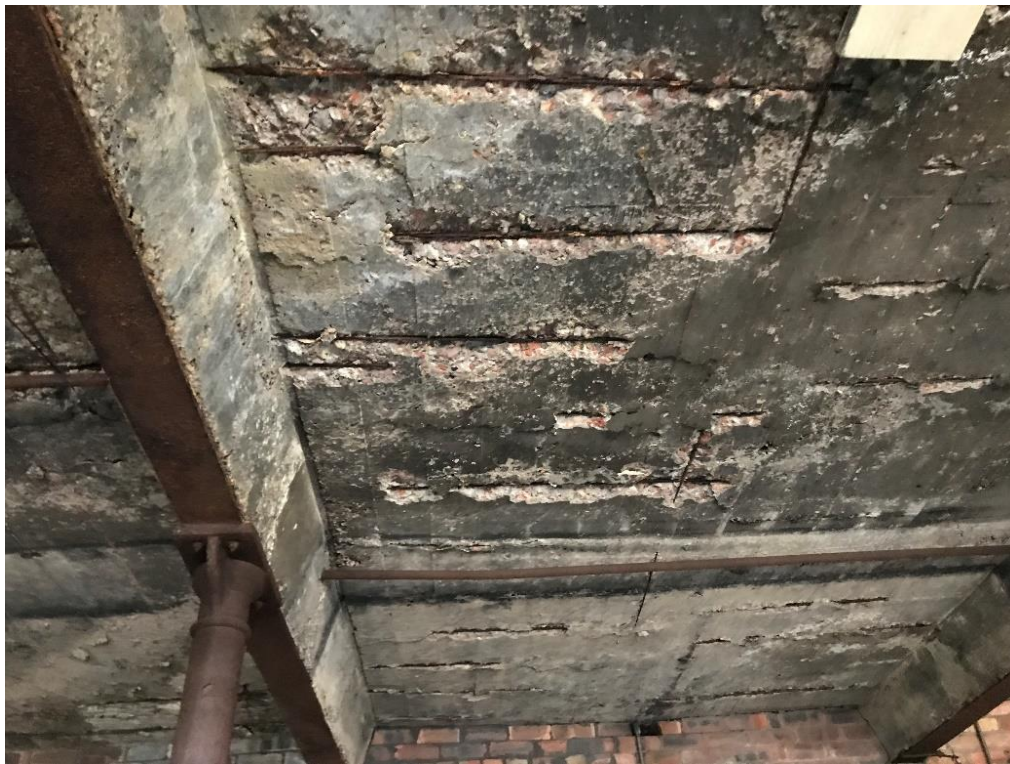
Figure 41: Spalling of Concrete due to Water Ingress and Corrosion of Reinforcement
