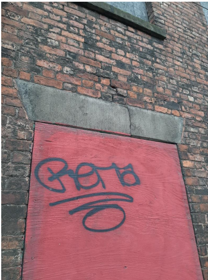
Figure 93: Typical Lintel Failure
