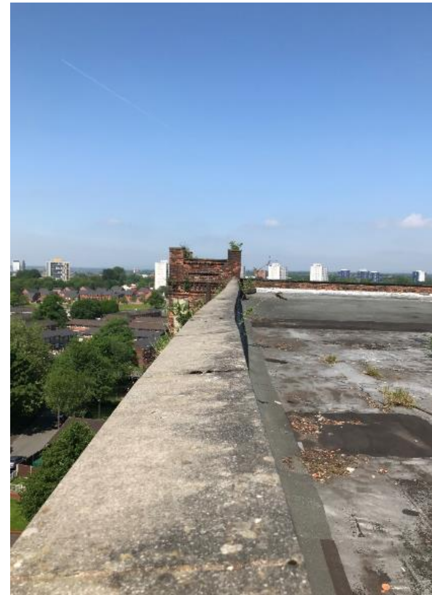
Figure 70a: Bowing Parapet.
