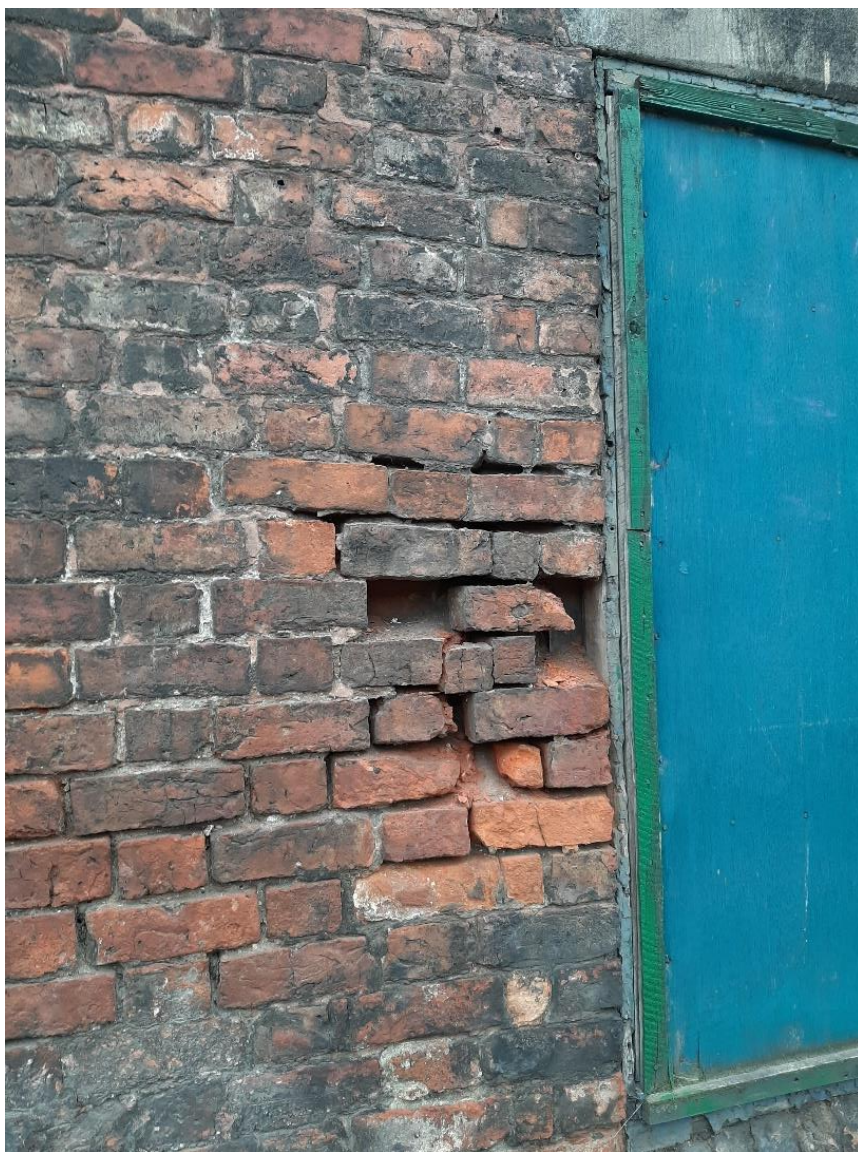
Figure 97: Masonry loss of pointing on External Elevation
