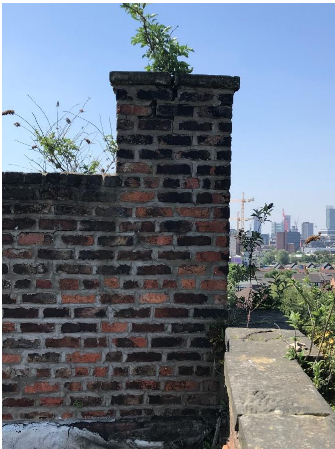
Figure 16: Leaning Dust Chute
