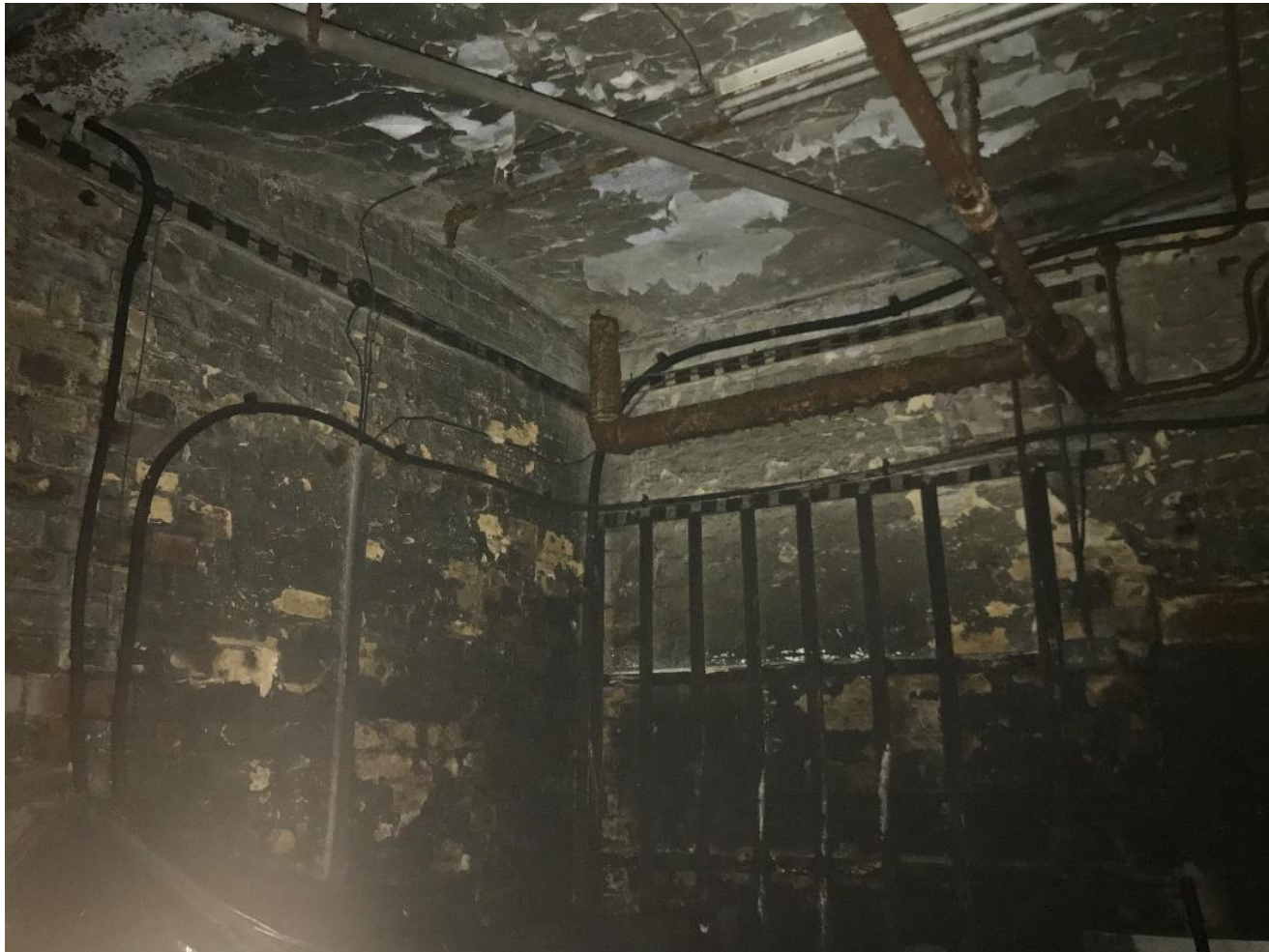
Figure 58: Significant Staining to Walls
