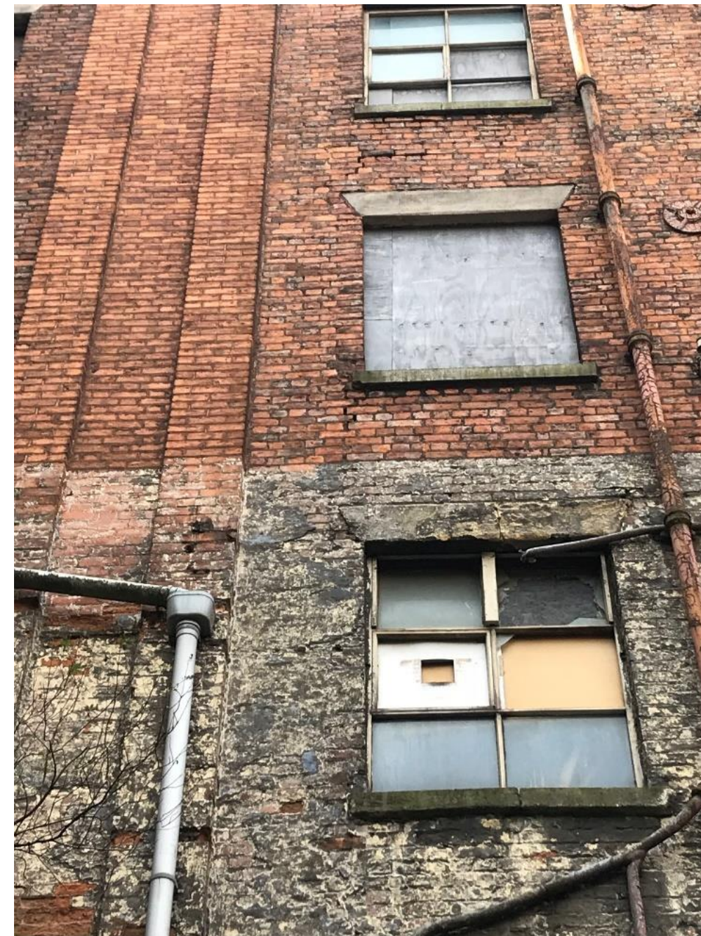
Figure 92 Localised Cracking to Masonry Panel and Lintels of Poor Condition
