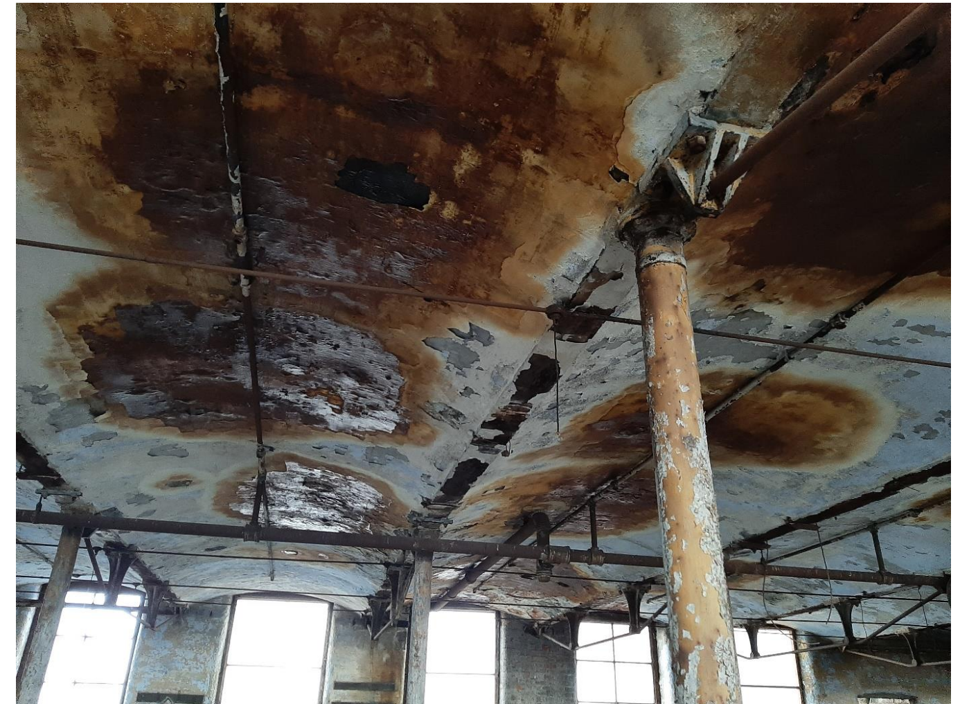
Figure 24: Significant Water Staining to Soffit. Strengthening Observed to Beams
