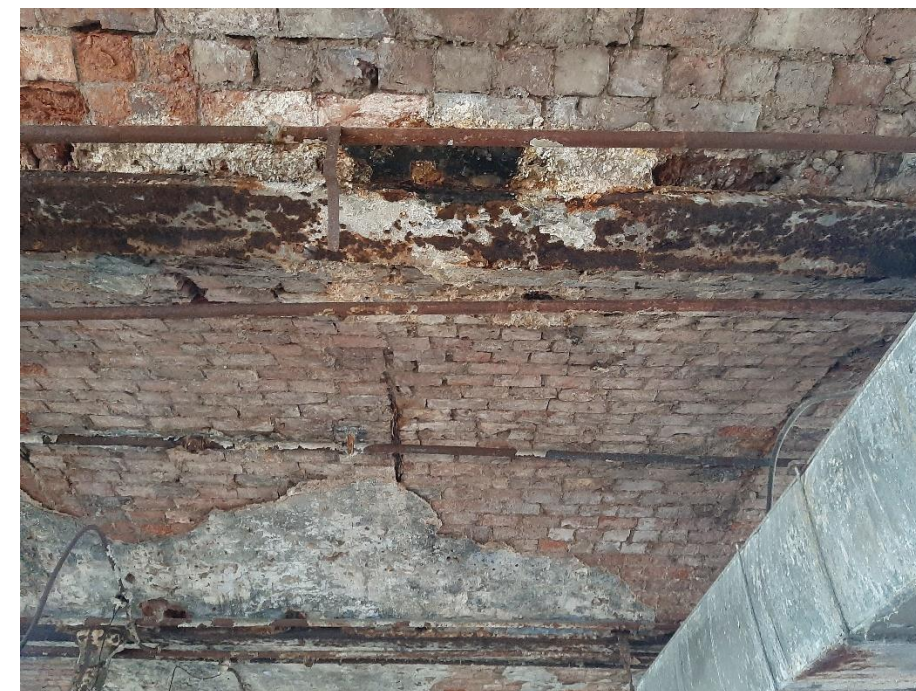
Figure 20: Significant Loss of Plaster, Masonry Units and Pointing to Jack Arches
