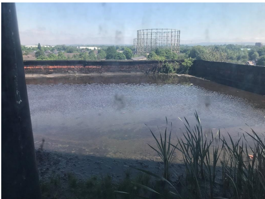
Figure 29: Water Ponding on Waste House Roof
