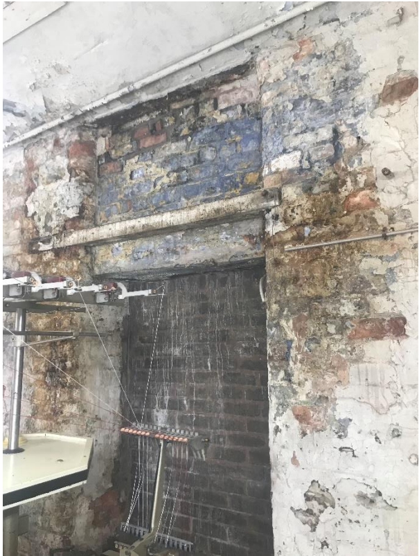
Figure 49: Significant Water Staining and Damage to Brickwork
