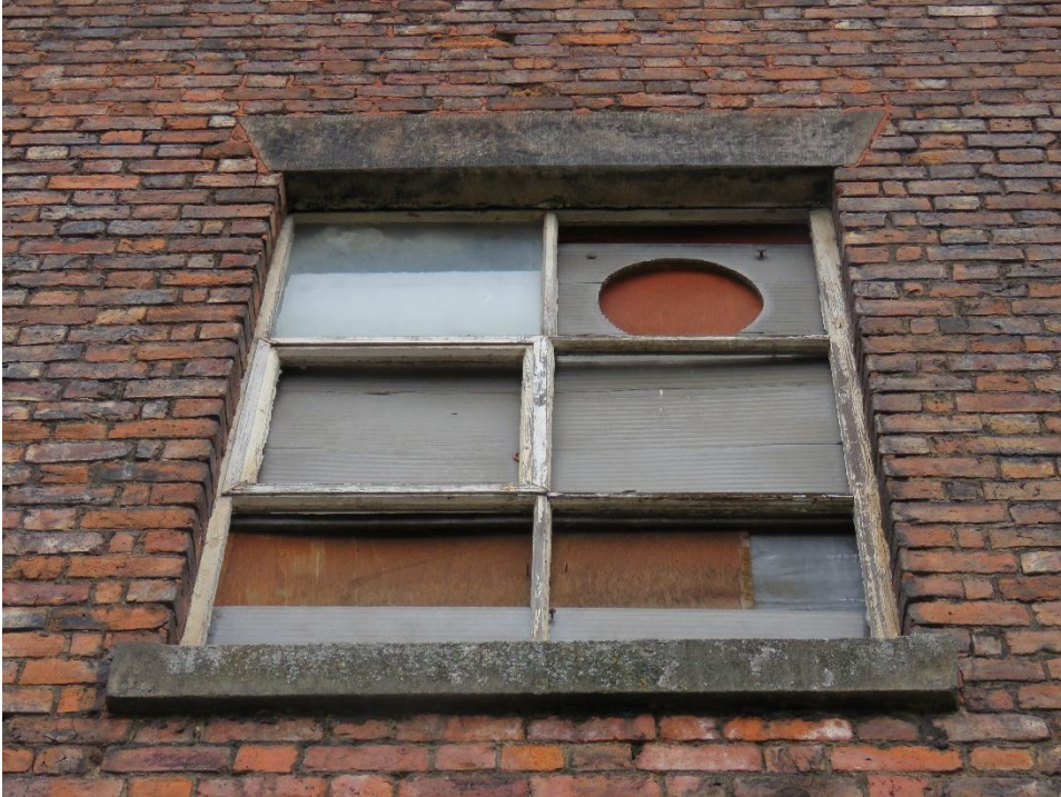
Figure 11: Typical condition of a surviving timber framed window with replaced / missing / broken panes, flaking paint and boarded over.
