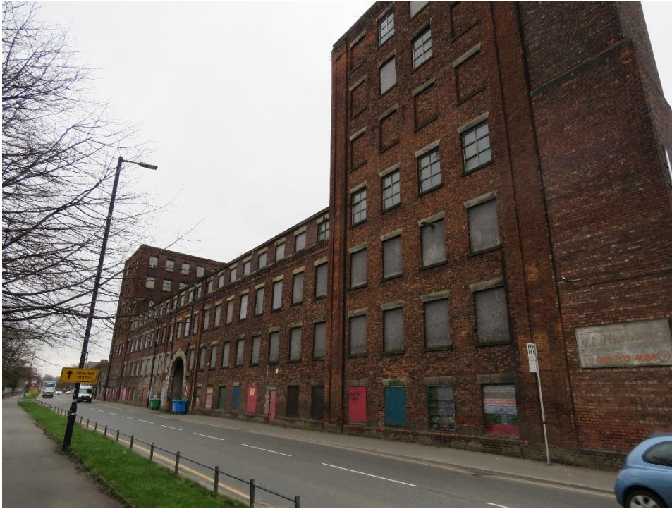
Figure 10: General view of the north elevation showing number of blocked up window openings.
