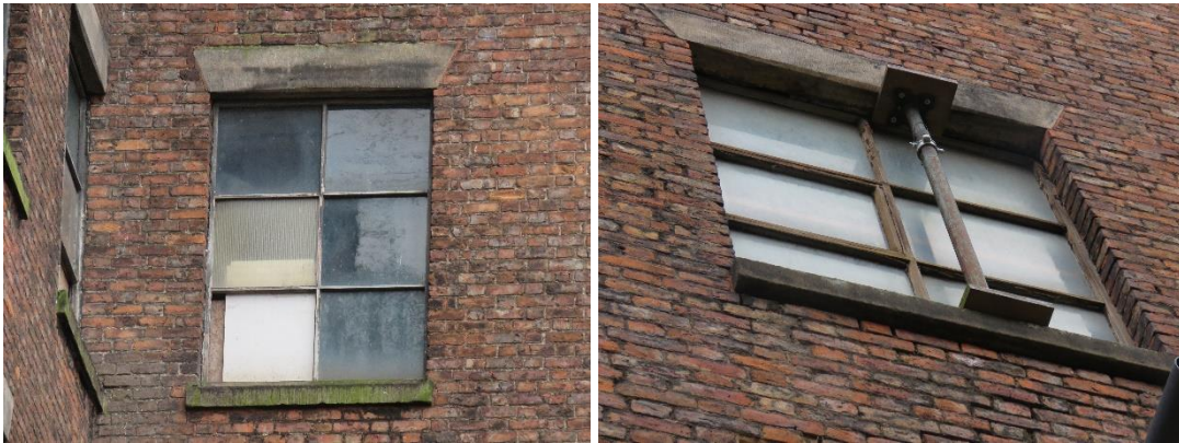
Figure 2 (left): Timber framed 6 pane window with no openable panes, and Figure 3 (right): With a single middle pane that is openable.
