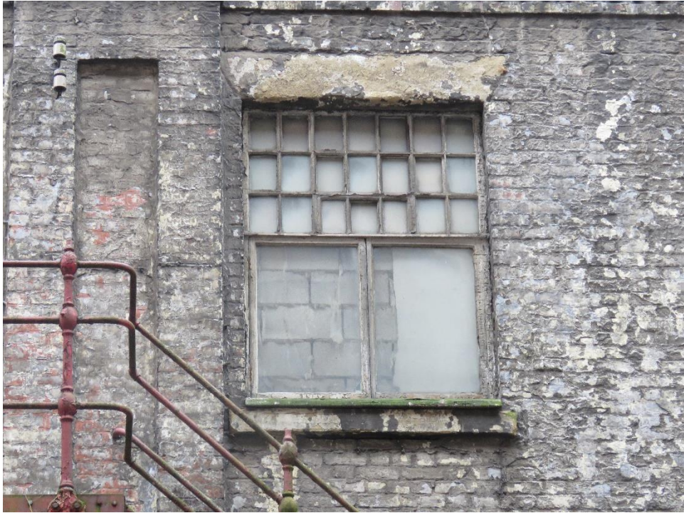
Fig. 1. The multi-pane upper section of this inner courtyard window is believed to be the only surviving section of original window to the mill.
