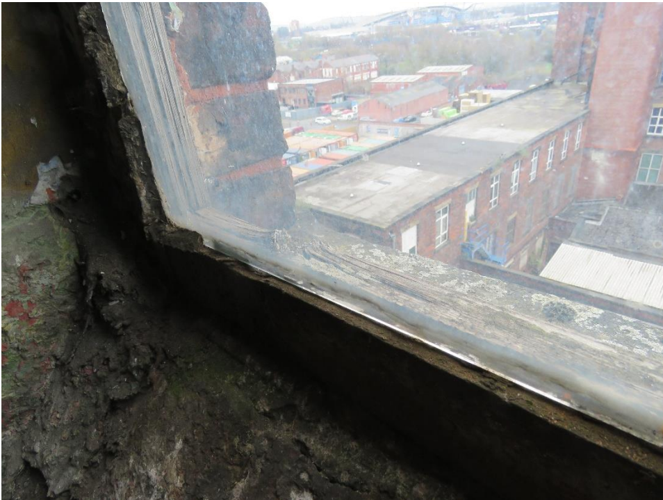
Figure 12: View of cill showing flaking paint, failed glazing putty and minor timber decay to cill.
